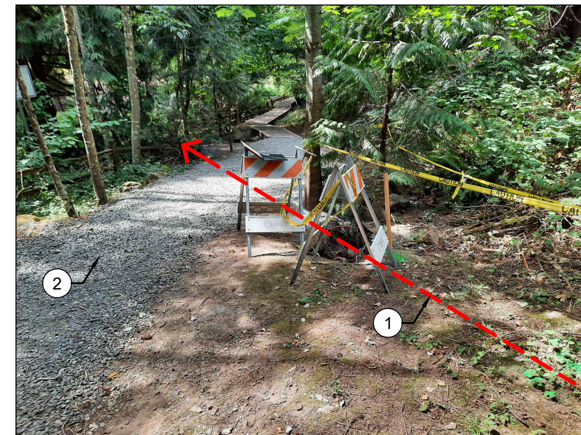
PHOTO 10 BROKEN SECTION OF swPP-014775 EXPOSED FROM GROUND SURFACE
