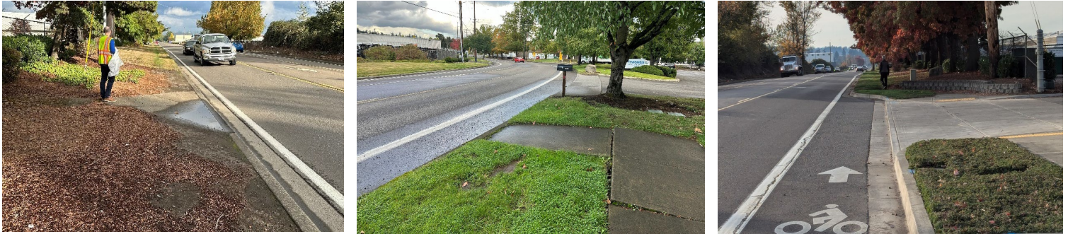
Existing conditions photos highlight gaps in the sidewalk and biking network, and non-compliant ADA curb ramps.
