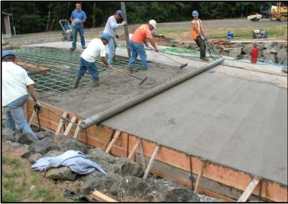
Photo 3-31 Placing fresh concrete into forms and using a power screed to level concrete with tops of forms
