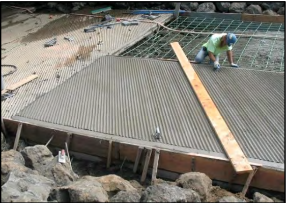
Photo 3-34 Final refinement is done with hand tools including a flat 4" border at edges. Note groove angle matches precast planks.
