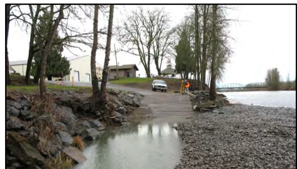
Photo 3-4 Launch ramp aligned nearly parallel to river. Development of gravel bar has made this ramp unusable at lower water levels.
