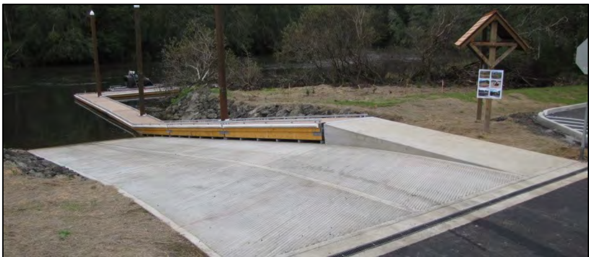
Photo 3-10 Single-lane launch ramp with boarding floats. Lane width is 20 feet with cold joint centered on launch lane.
