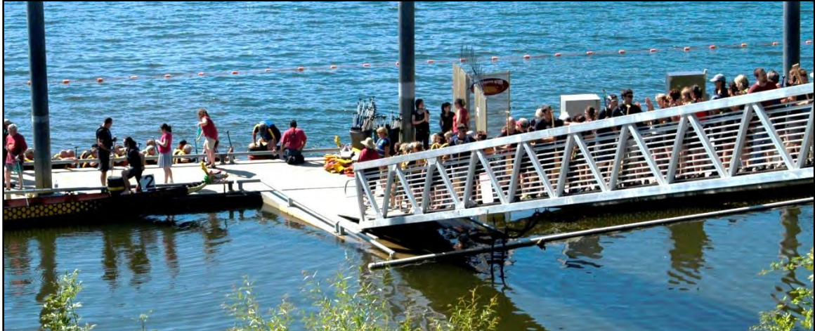
Photo 5-11 Inadequate flotation to compensate for gangway live load. Gangway support floats should be floating level under this loading condition – not submerged at shore end. Although the load is still supported this may induce stresses at the connection points and conveys a visual sense of being unsafe.
