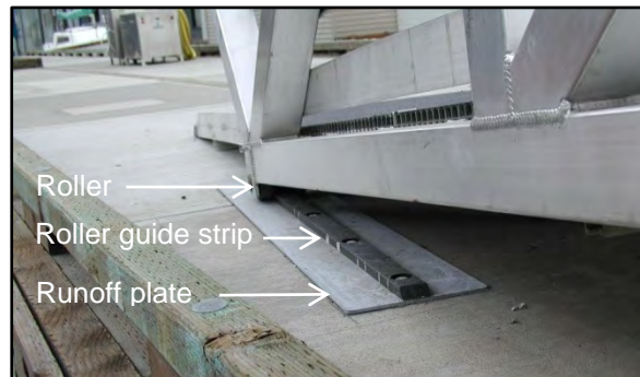
Photo 7-8 Runoff plate at float end of gangway. A grooved roller rides on the HDPE roller guide strip and provides side-restraint.
