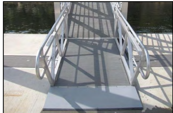
Photo 7-5 Transition plate at float end of gangway. In this application handrails are required since the slope exceeds 5%.
