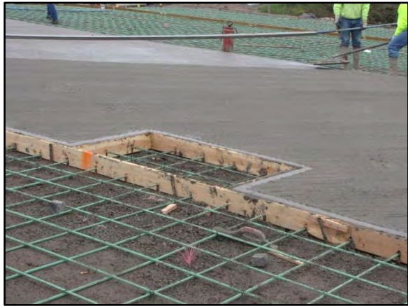
Photo 3-21 Longitudinal cold joint at edge of launch lane and form boards notched for rebar. Rebar will be blocked prior to placement of concrete.
