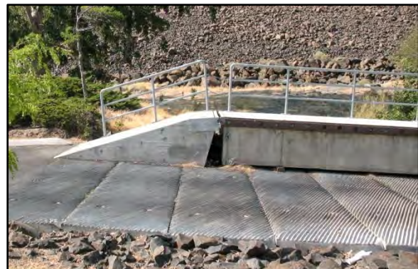
Photo 4-9 Example of floats that are too tall when grounded on the launch ramp. The slope of the abutment is also excessive.
