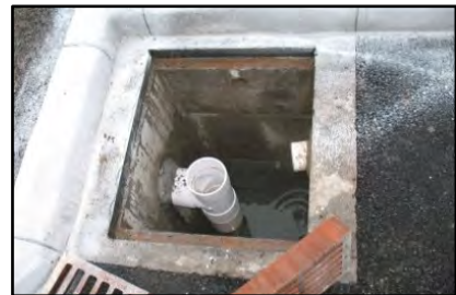
Photo 3-38 Trapped catch basin
