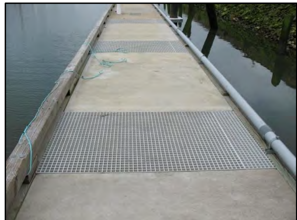
Photo 5-12 Grating in deck surface to allow for light penetration through the float
