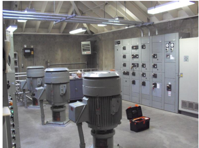
Willamette Pump Station
