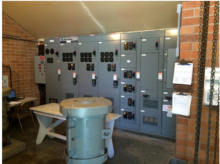
Astoria Pump Station #1 Finished MCC Lineup
