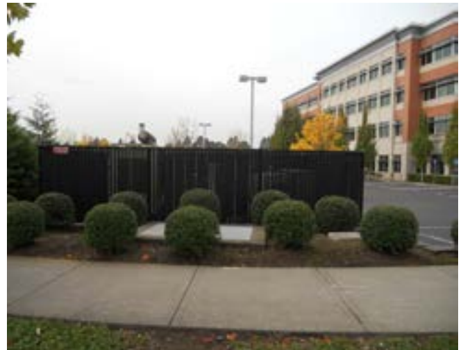
PSB generator equipment screening from Kaen Road Slatted painted chain link, 6-foot high.
