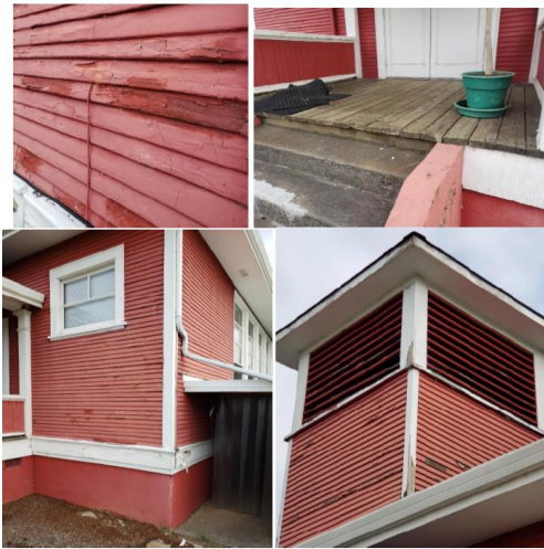
Figures 4, 5, 6 & 7 - Exterior views of subject property indicating deterioration of facade material
