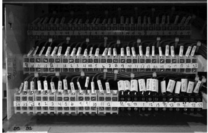
Figure 16. Master Terminal Block
