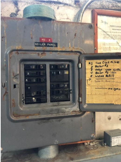
Photo E4: Example of older load centers in kitchen area
