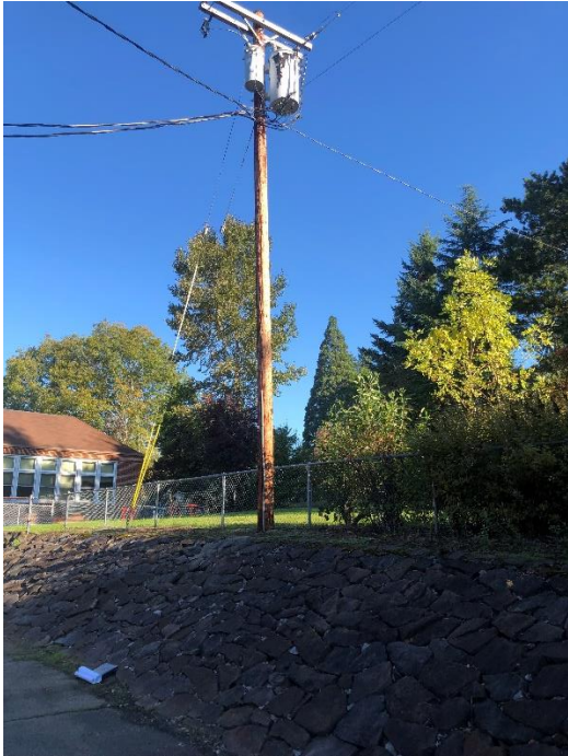
Photo E3: Outdoor pole-mounted transformer serving electrical services
