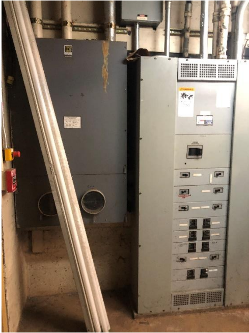
Photo E1: Existing main switchboard in boiler room.
