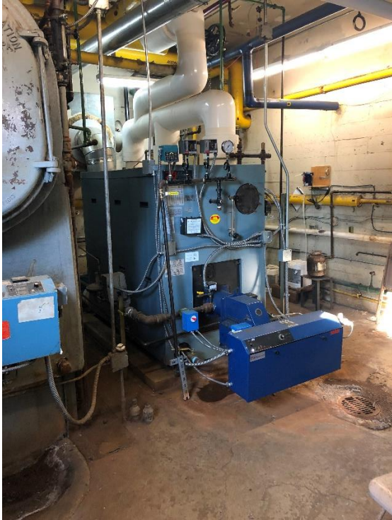
Photo M5: Steam boiler
