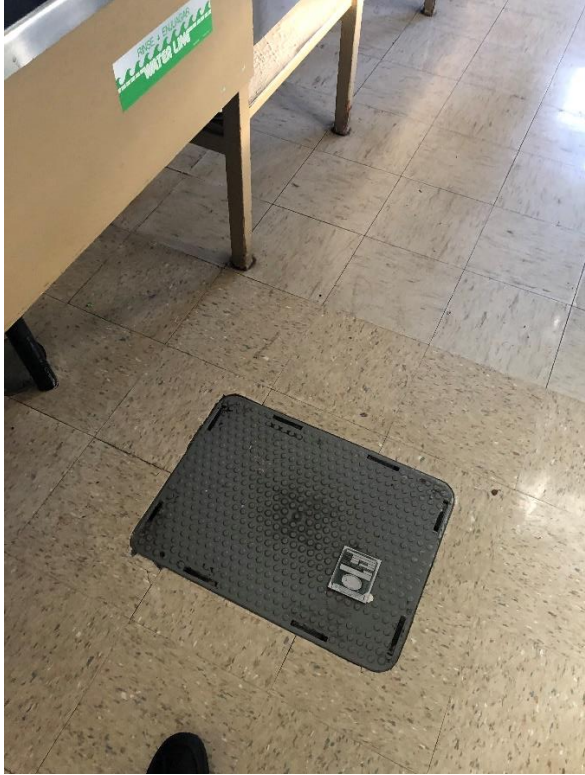
Photo M3: Kitchen grease interceptor
