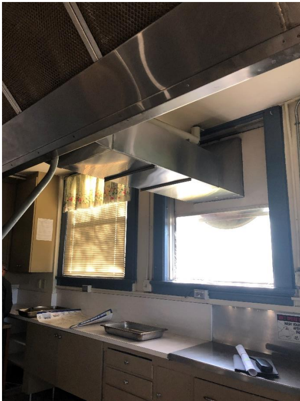
Photo M4: Kitchen grease fan/duct
