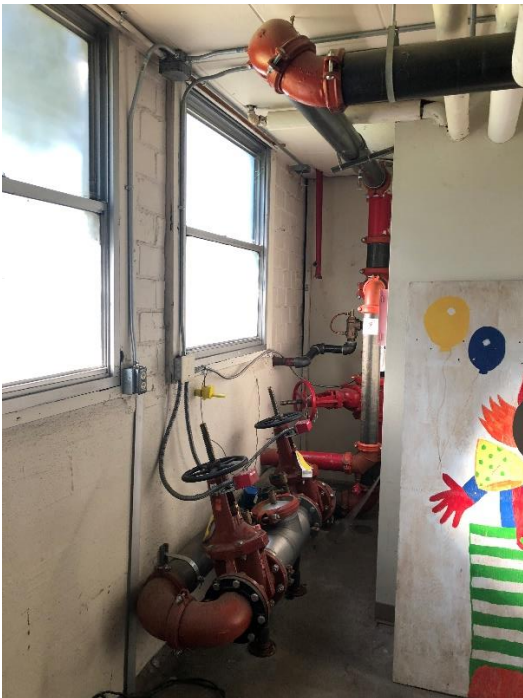
Photo M2: Fire sprinkler service
