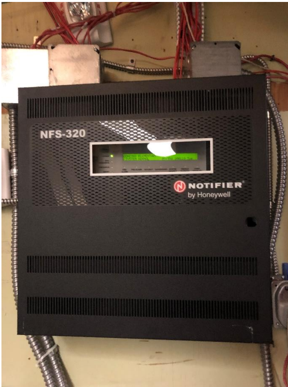
Photo E6: Existing Fire Alarm Panel
