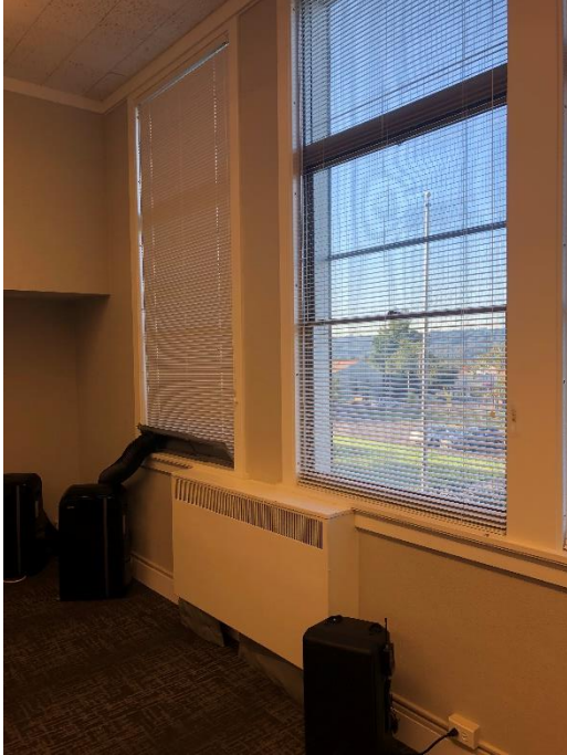
Photo M1: Classroom unit ventilation
