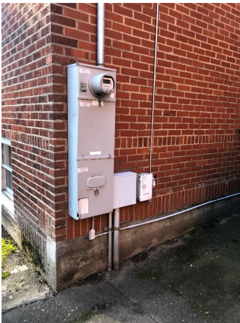
Photo E2: Separate three-phase, open delta service for elevator
