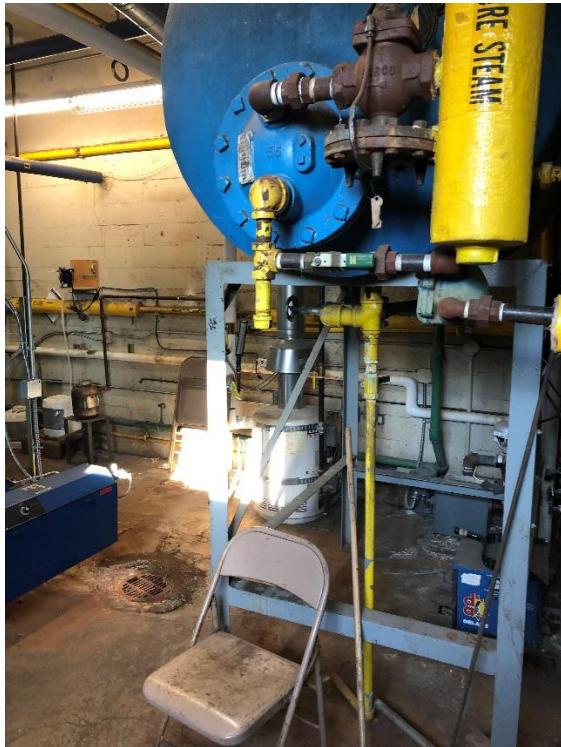
Photo P1: DHW Controller
