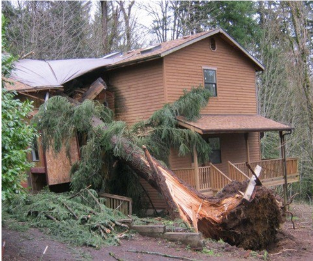
Windstorm damage – March 13, 2011
