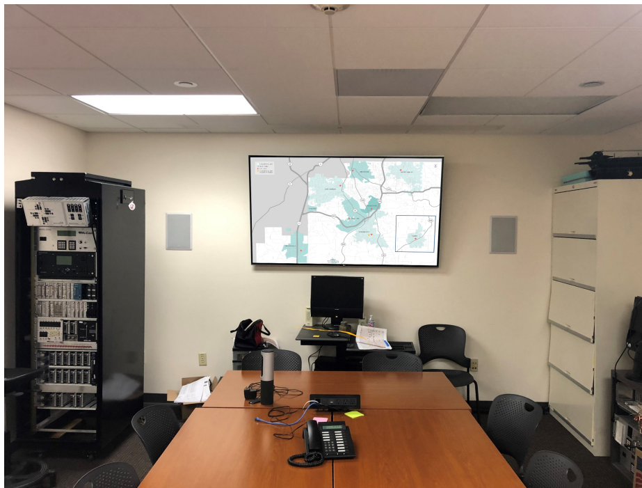
FIGURE 4: CLACKAMAS COUNTY TRAFFIC OPERATIONS CENTER (TOC)
