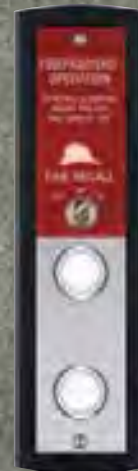
Intermediate hall station With fire services devices
