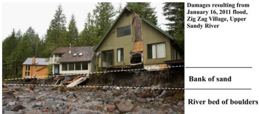
Figure 30. Home damage along the Upper Sandy River due to erosion in 2011 along right bank at Zigzag Village development, RM 45.1. Like much of Upper Sandy, the bank is composed of fine sediment that is more easily eroded than the coarse material of the river bed. Photo credit: The Oregonian newspaper.
