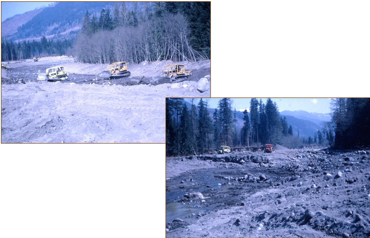
Figure 19. Army Corps of Engineers Bull Dozers Re-Grading the 1964 Channel. Following the 1964 flood the ACOE mechanically graded over the active channel to recover the pre-'64 single stem channel. The re-grading straightened and shortened the 1964 channel, increasing the channel gradient in the process. Note the large proportion of fine grained materials comprising the flood deposits. Photos courtesy of Raymond Arrigotti.
