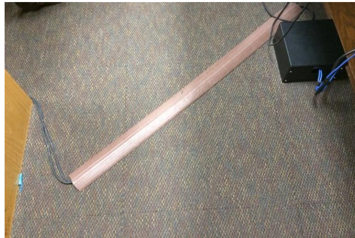
Cables at litigation well in courtroom
