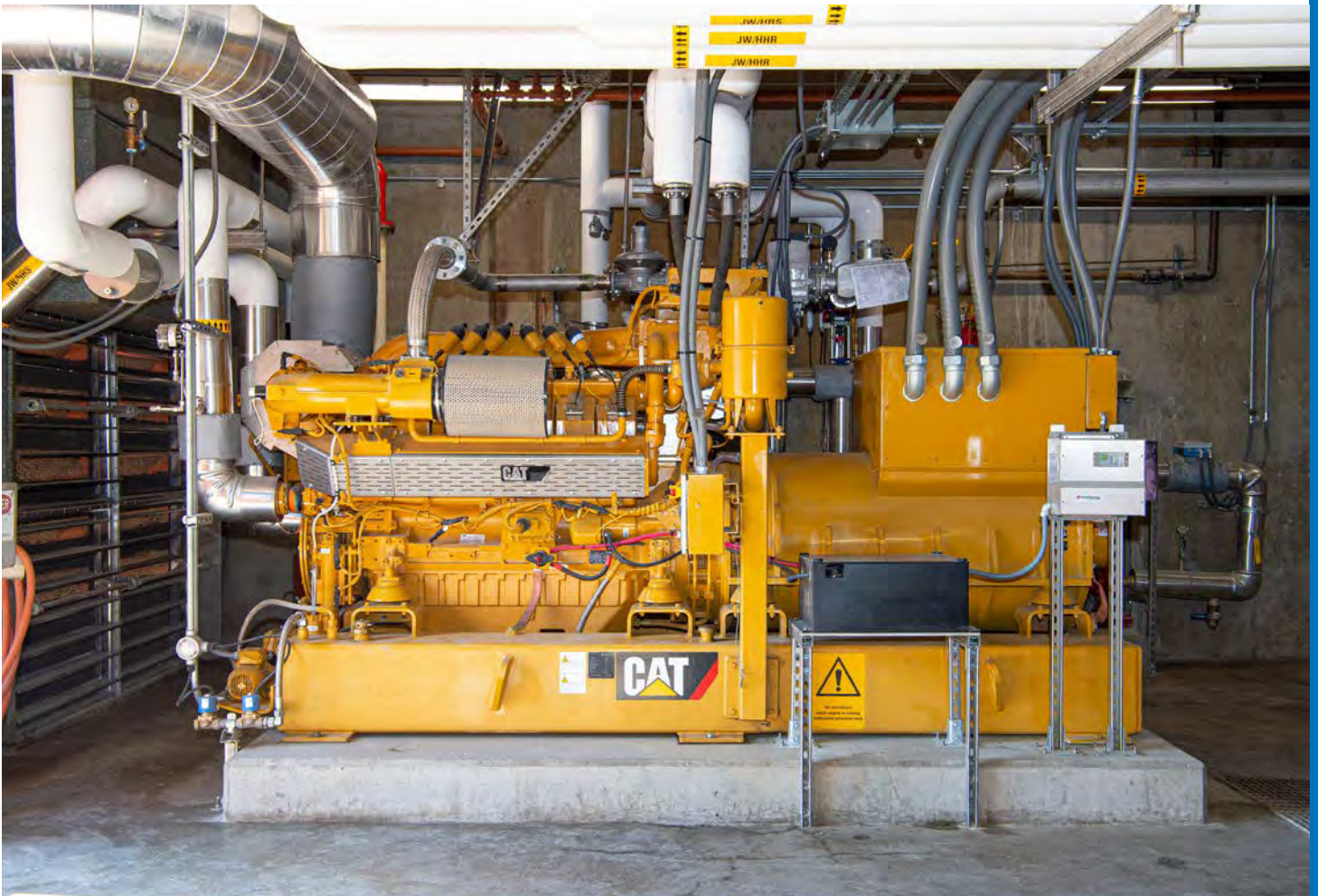
A new 600-kW lean-burn engine connects to the digester and converts the methane gas into heat and electricity — enough to power nearly half of the Tri-City facility and produce heat for five buildings.
