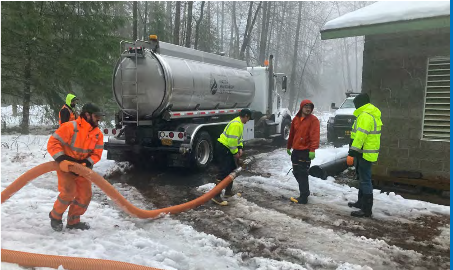
Operators braving the elements to provide 24/7 service
