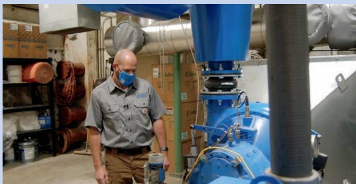
Kellogg Creek Operations Supervisor Joshua Clark inspects recently installed equipment.
