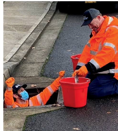
WES technicians Jeremy Bodner and Kevin Rotrock at the catch basin where they recovered the ring.
