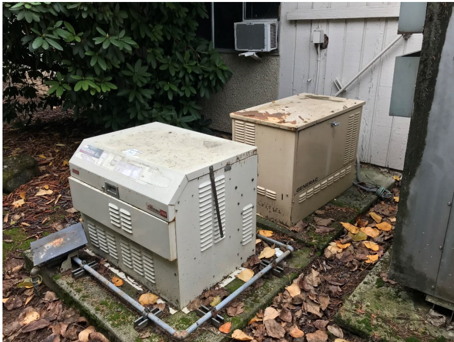
Photo 8. Backup generators. Located off the northeast corner of the building
