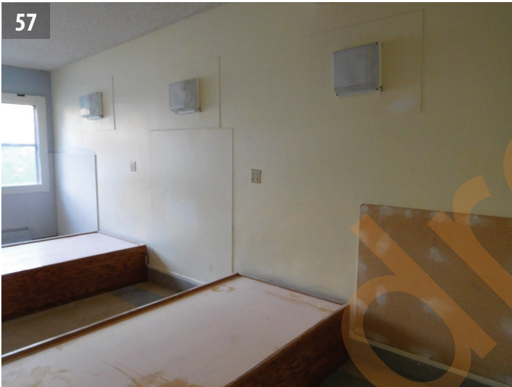
Wall patched with sheathing in lieu of GWB at Unit 18.
