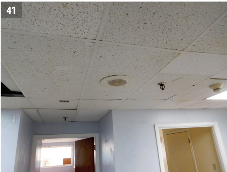
Typical condition of the suspended acoustical tile ceiling and grid, as seen at the common corridor of the east wing.
