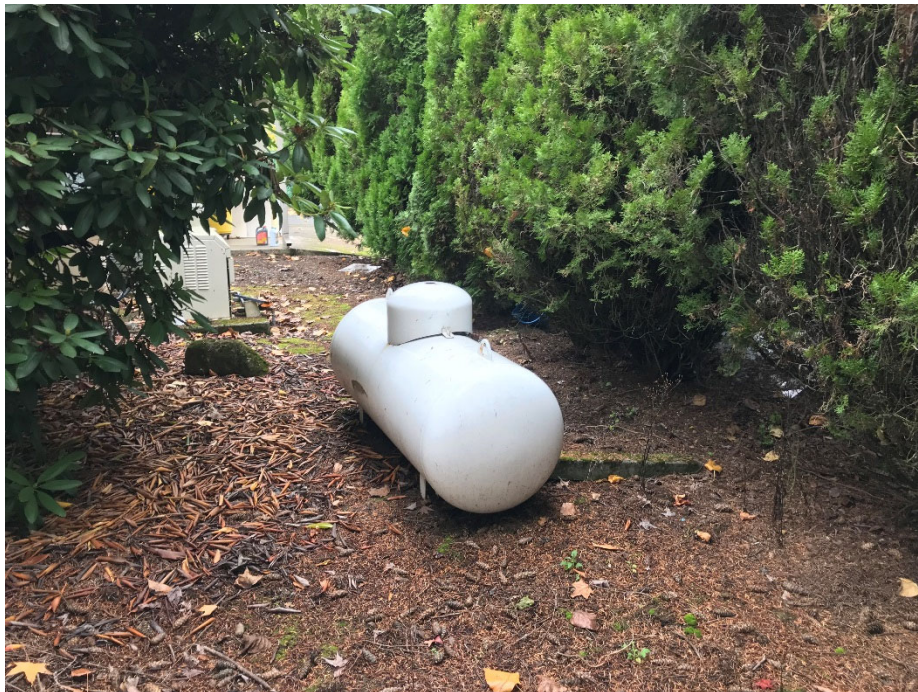
Photo 10. Small propane AST. Located off the northeast corner of the building
