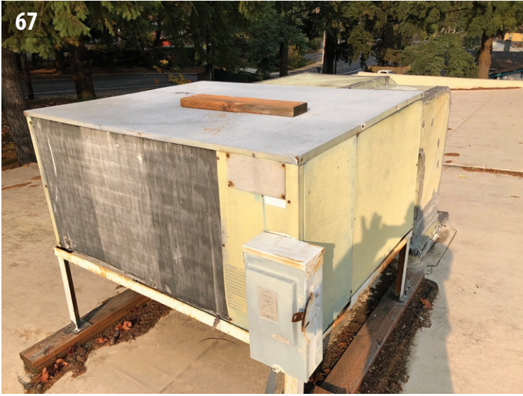
Packaged RTU serving the kitchen.
