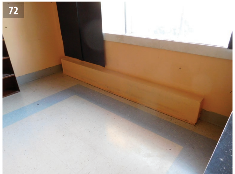
Typical covered baseboard radiator at a dwelling unit.
