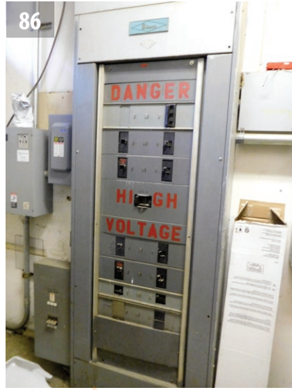
86 Main electrical-distribution panel manufactured by Zinsco.
