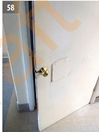
Patched interior door at Unit 18.
