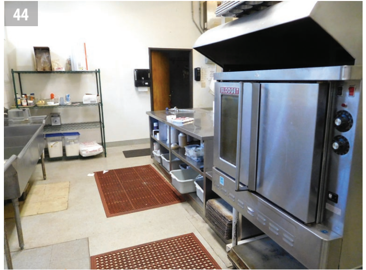
Commercial kitchen equipment.
