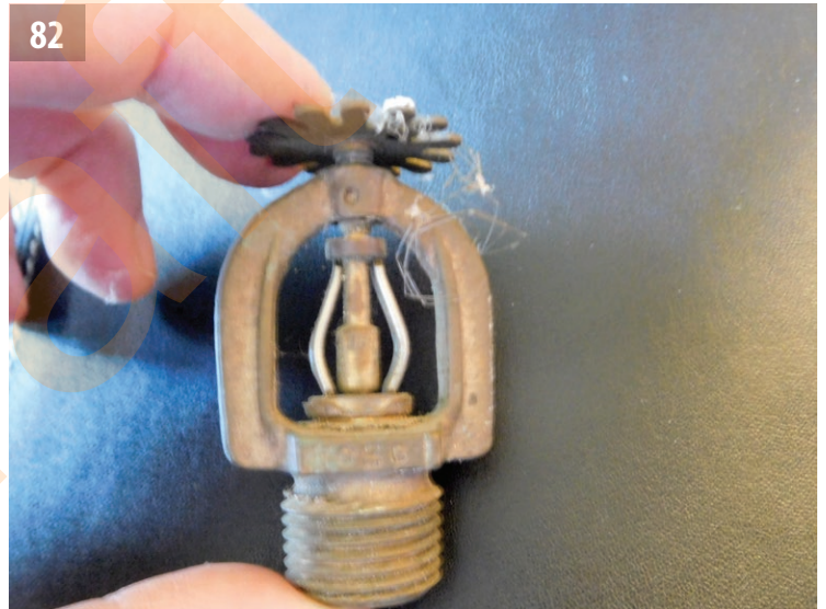
Central-manufactured (CSC) sprinkler head found in the spare-sprinkler-head cabinet.
