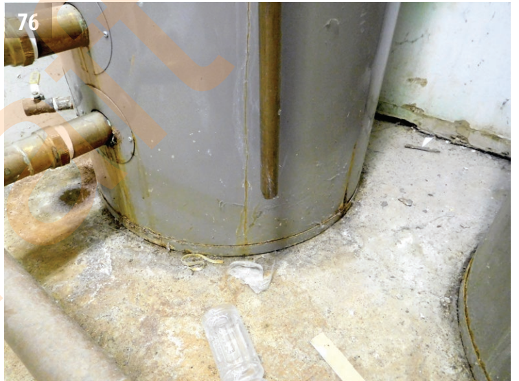
76 Corrosion at the base of the hot-water storage tank.
