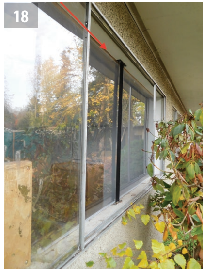
Missing glass at an aluminum-framed window, with interior plexiglass storm window pane remaining.
