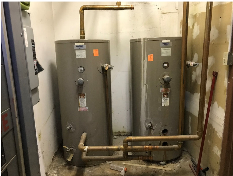
Photo 6. Interior natural gas water heaters
