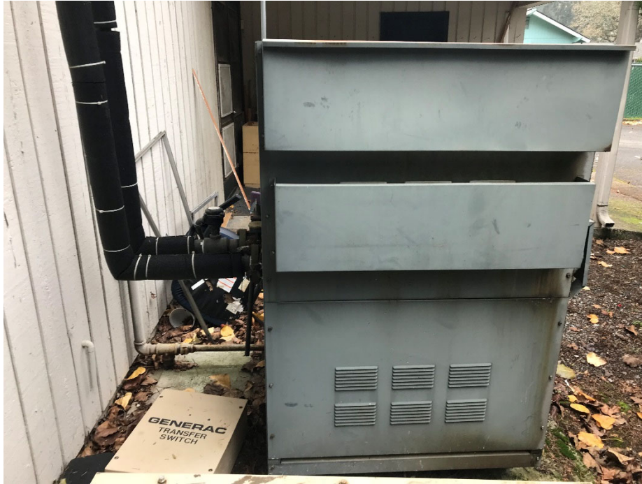
Photo 9. Exterior hot water heater. Located off the northeast corner of the building
