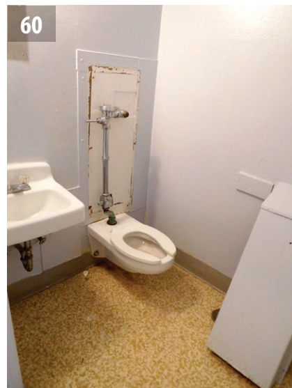
Flush-valve toilet with protective cover removed at Unit 19.
