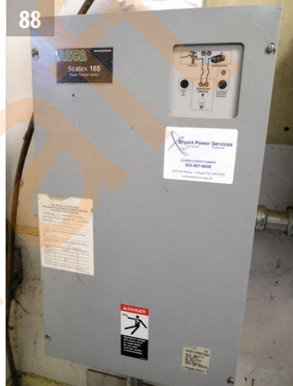
88 Automatic transfer switch for the emergency generator.
