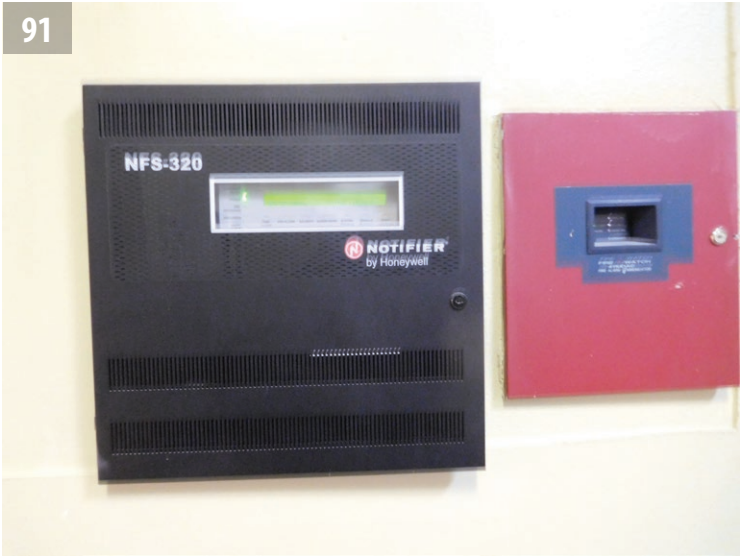
Notifier fire-alarm control panel (FACP).
