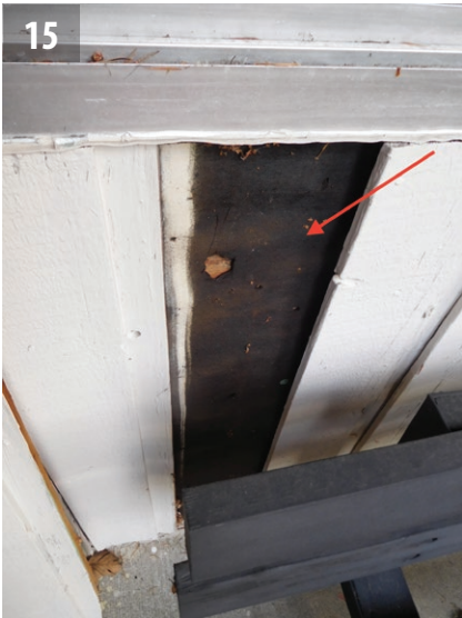
Dislodged siding with underlying building paper and plywood sheathing.
