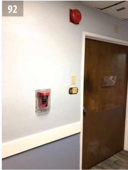
Fire-alarm bell and pull station at the common corridor.
