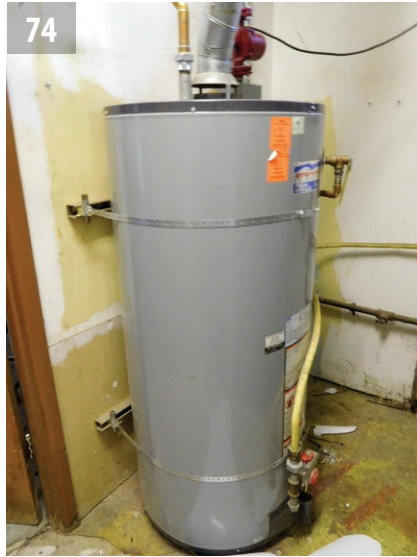
74 75-gal gas-fired water heater.
