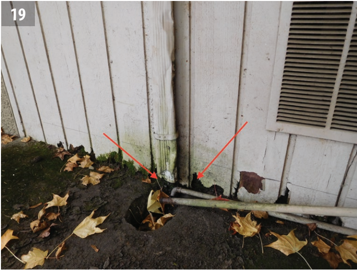
Rotted T1-11 siding at the base of the exterior wall and missing downspout boot.
