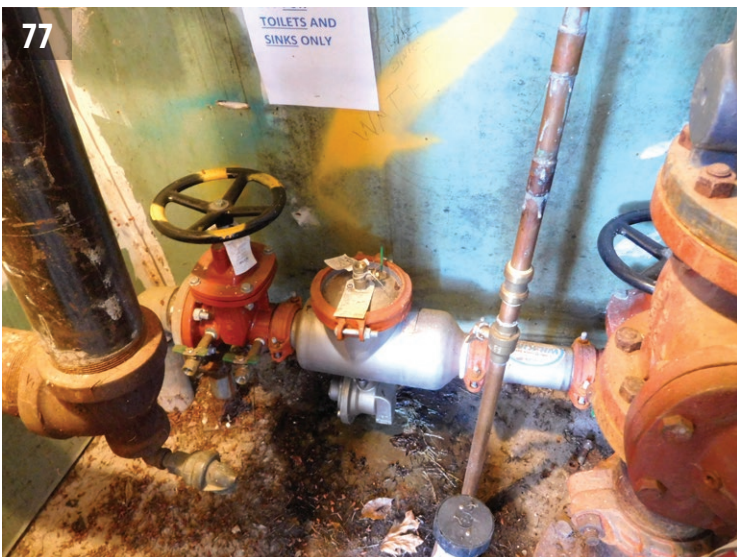
77 Backflow preventer on the domestic-water service.
