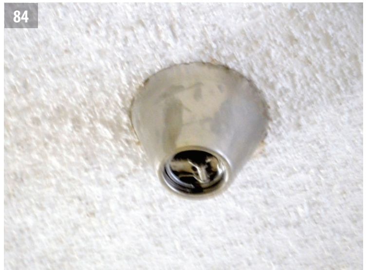
Sprinkler head at a dwelling unit.
