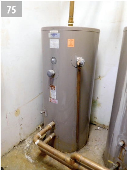
75 120-gal hot-water storage tank.
