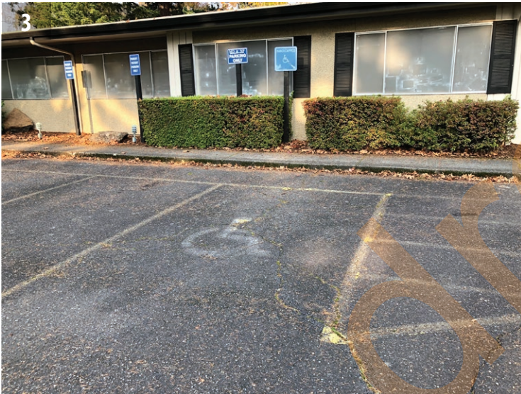
Vertical signage, faded striping, and lack of an access aisle at the parking area.
