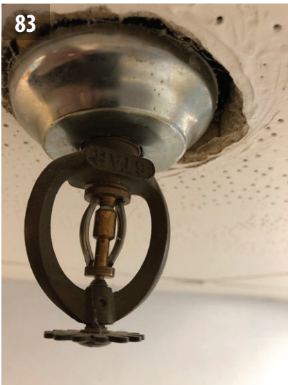
Star-manufactured sprinkler head at the common corridor.
