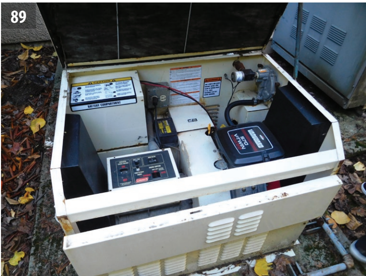
89 Coleman propane-gas-fired emergency generator.
