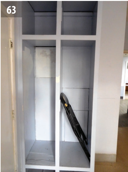
63 Painted armoire with no closet doors or shelving at Unit 24.
