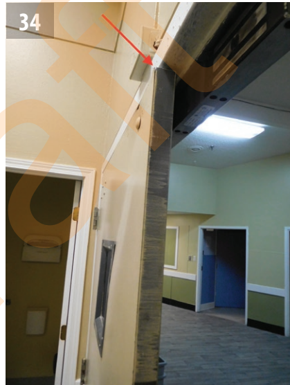
Warped vestibule door.
