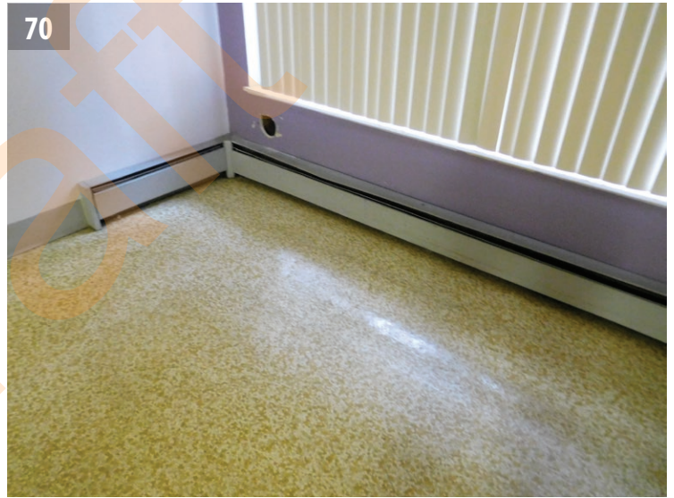
Hot-water electric heat baseboard radiator at Unit 41.
