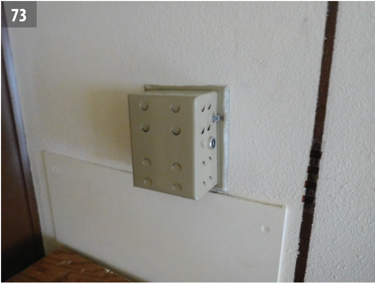
73 Typical covered thermostat at a dwelling unit.
