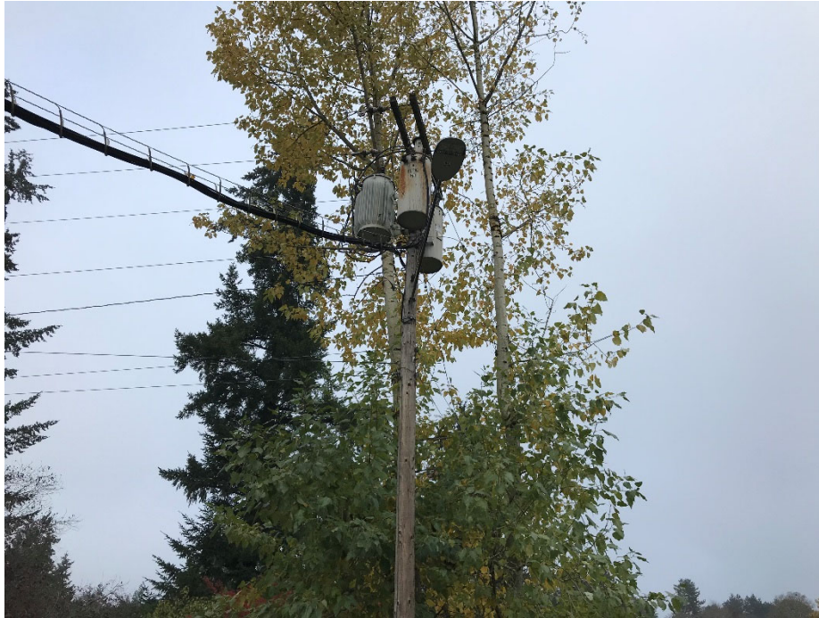
Photo 17. Pole-mounted transformers, rust and historical leaking noted
