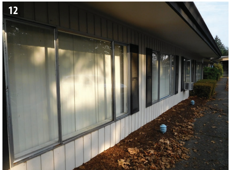
T1-11 siding and aluminum-framed windows at the south elevation of the west wing. Note that subgrade is covering the bottom of the siding.
