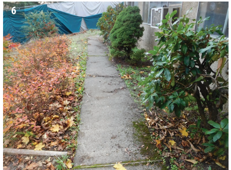
Sidewalk north of the east wing that is sloped toward the building.
