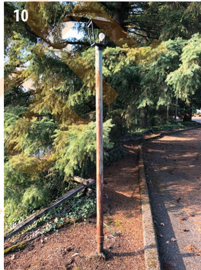
Condition of a typical site lightpole and fixture.
