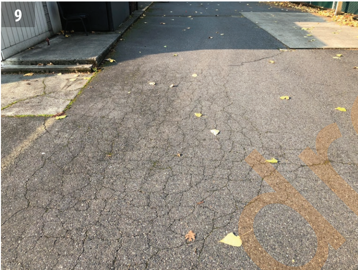
Alligatored asphalt pavement at the rear drive.
