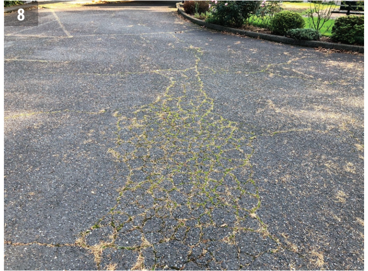
Alligatored asphalt pavement at the front drive, with vegetational growth through the cracks.
