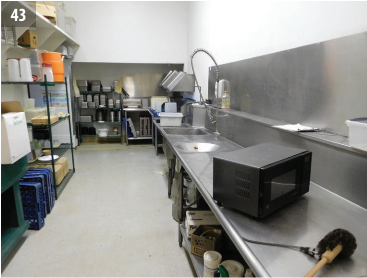
Commercial kitchen equipment.
