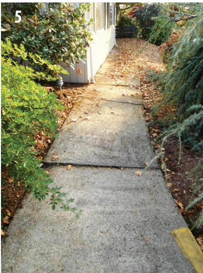
Heaved section of sidewalk.
