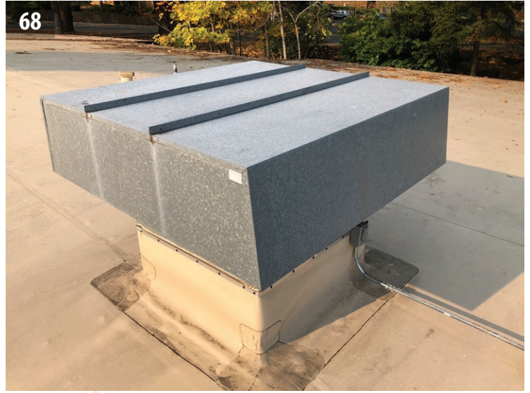
One of three rooftop exhaust fans that serve the corridors.
