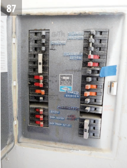
87 Smaller electrical-distribution panel manufactured by Zinsco.
