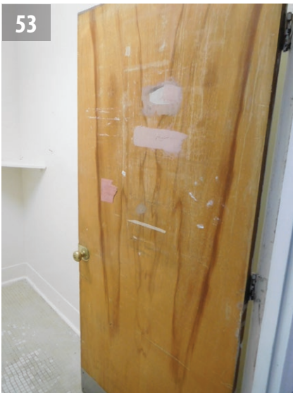
Damaged door to a shower room at the east wing.
