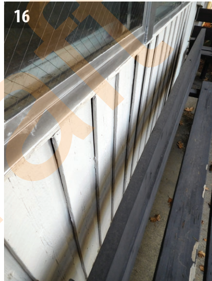
Section of cupped siding at the south elevation of the east wing.
