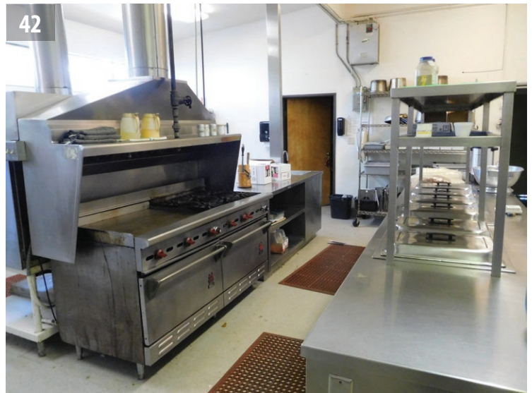
Commercial kitchen equipment.
