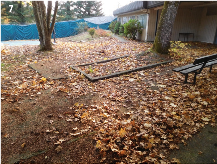
Heaved patio section at the northeast side.
