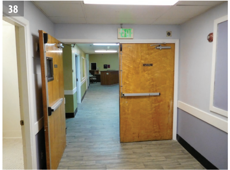
Magnetic-release, fire-rated doors at the west corridor.
