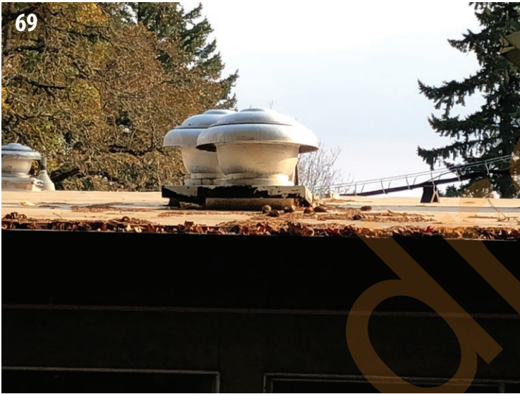
Kitchen-exhaust fans at the roof.
