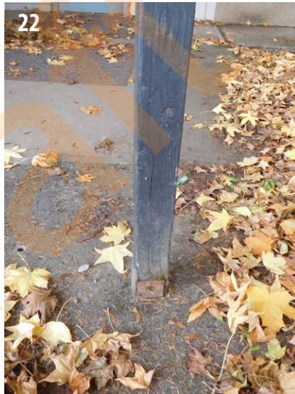
Warped wood post with some water damage evident at the base.
