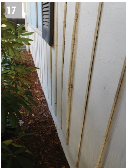
Open gaps in the T1-11 siding at the south elevation of the east wing.
