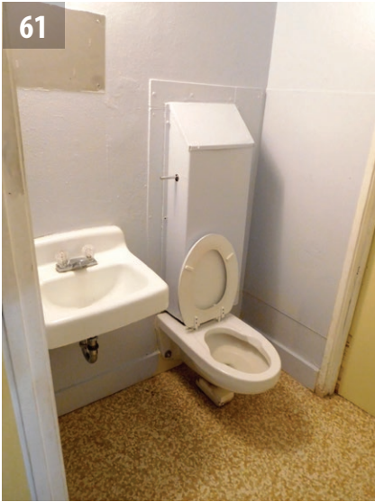
61 Flush-valve toilet with protective cover in place at the toilet room shared by Units 20 and 21.
