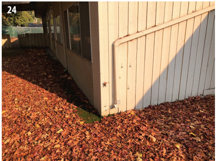
Missing downspout boot and extension at the west elevation of the north wing.
