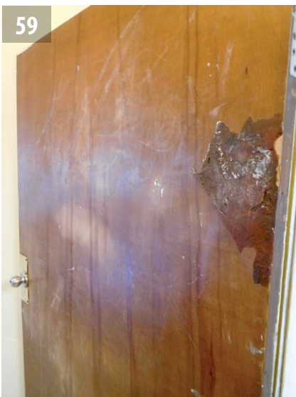
Damaged unit entry door at Unit 19.
