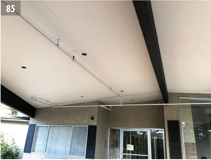
85 Sprinkler piping and heads exposed beneath the soffit of the porte-cochere.
