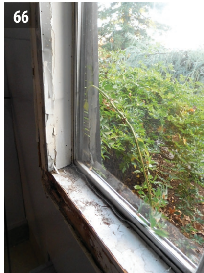
66 Water-damaged GWB around a window.
