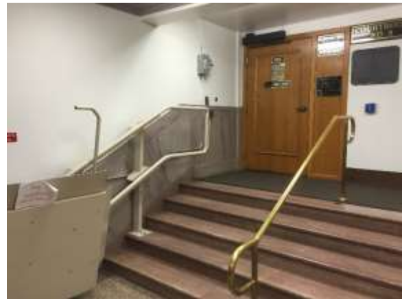
Image 7: Stairs up to Courtroom 8 and non-functioning lift due to inadequate existing wall bearing capacity
