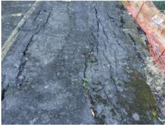
Image 16: Eroding asphalt at Willamette River elevation
