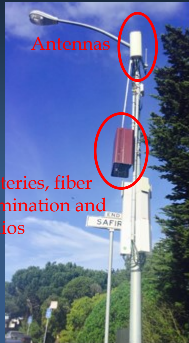
Light Pole - No Ground Cabinet
