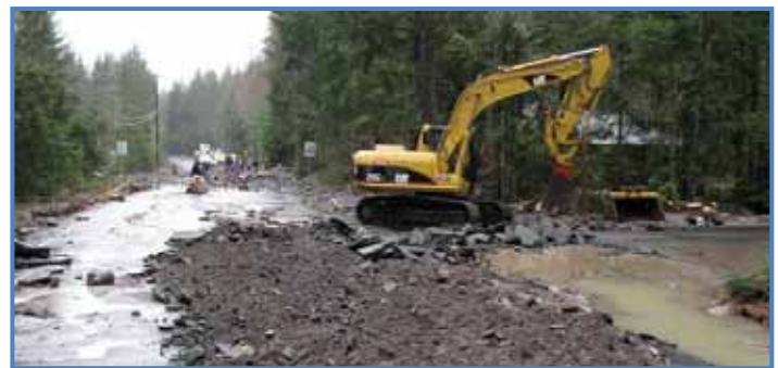
Flood Damage Closes Lolo Pass Road
