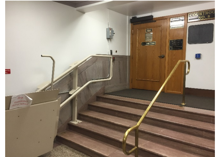
Stairs up to courtroom and non-functioning lift due to inadequate existing wall bearing capacity
