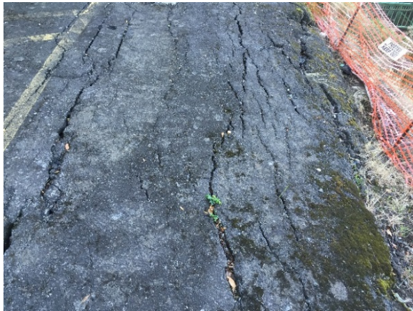
Eroding asphalt at Willamette River elevation
