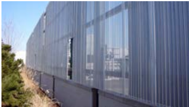
Central Utility Plant Equipment Enclosure Fence: Split face CMU with metal panels
