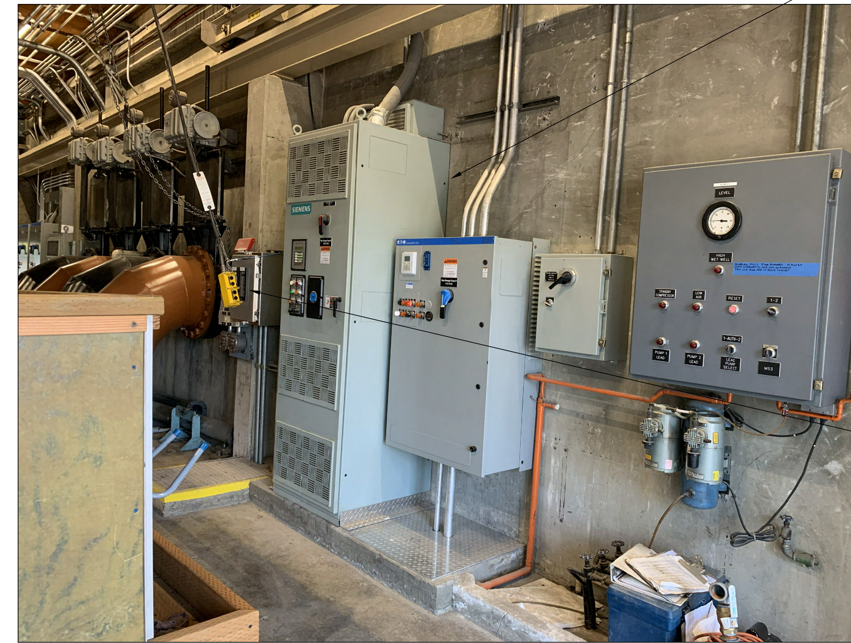
D PHOTOGRAPH 4 - RTD RELAY AND PUMP 2 VFD E-103 NO SCALE
