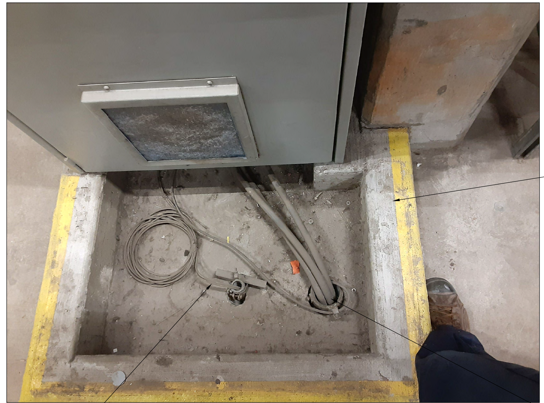
C PHOTOGRAPH 3 - PUMP 4 VFD CABLE TRENCH E-103 NO SCALE
