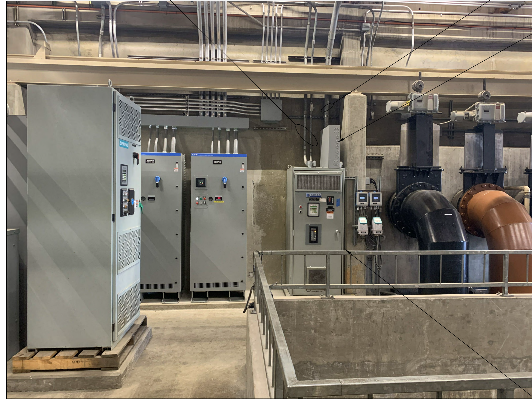
A PHOTOGRAPH 1 - PUMP 4 VFD E-103 NO SCALE
