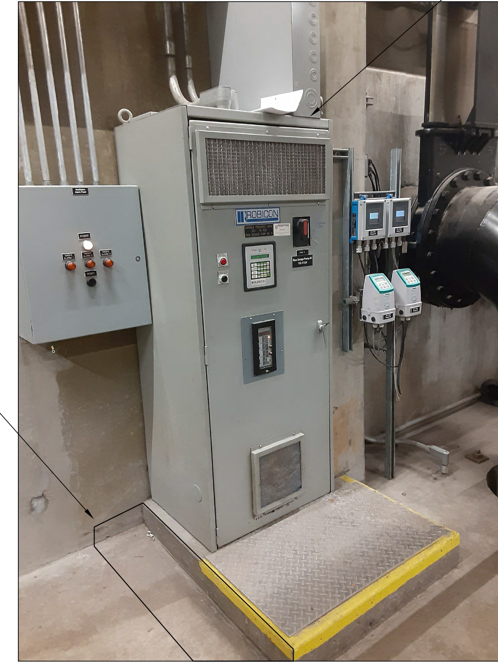
B PHOTOGRAPH 2 - PUMP 4 VFD E-103 NO SCALE
