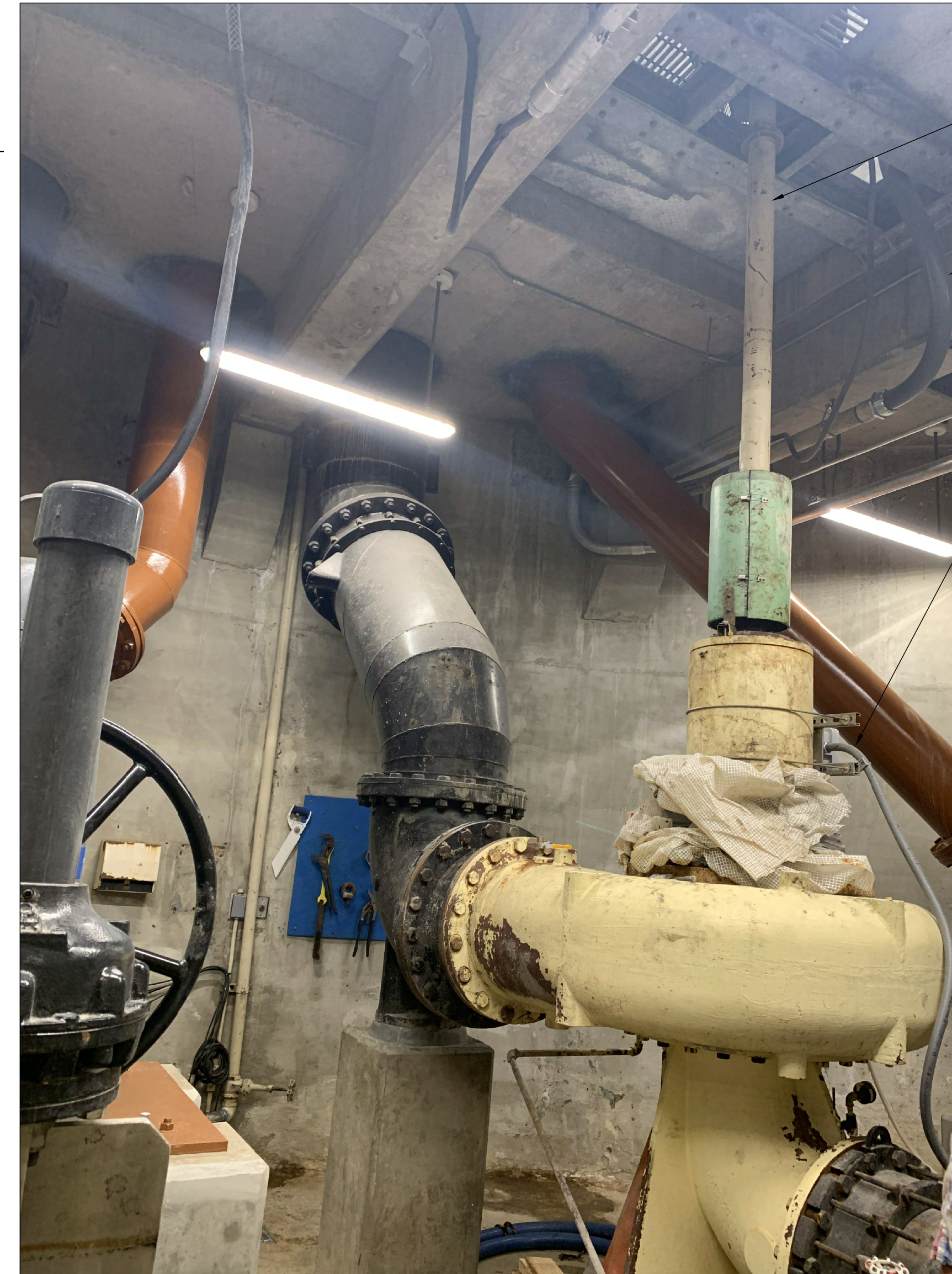
B PHOTOGRAPH 10 - EXISTING PUMP ED-101 NO SCALE
