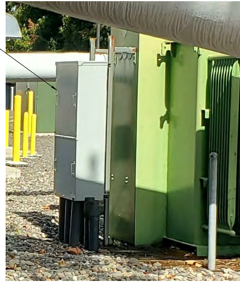
C PHOTOGRAPH 13 - ABANDONED 1000 KVA TRANSFORMER NO SCALE
