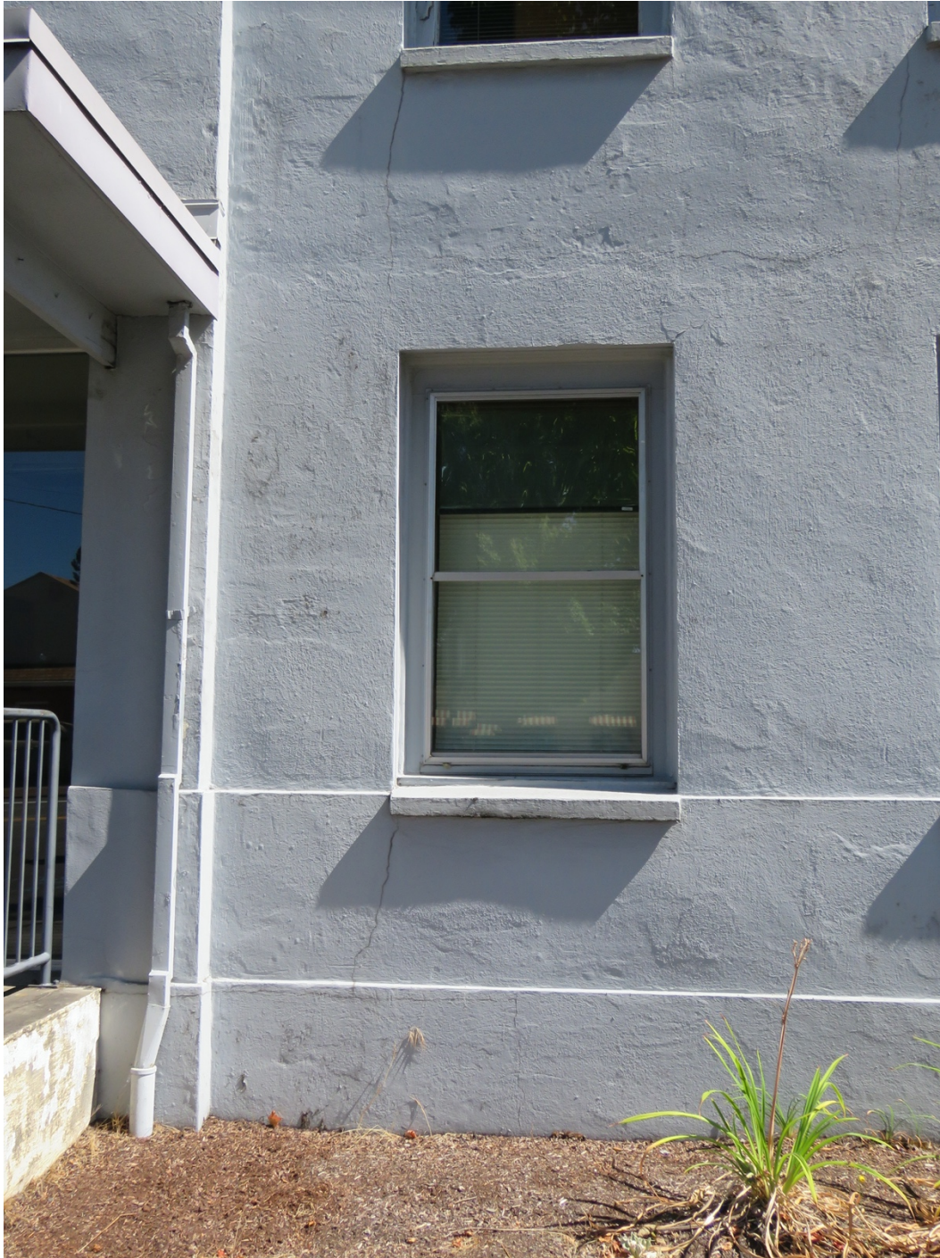
Detail of lower-story replacement window on primary (west) façade, view northeast (ARG, September 2020).
