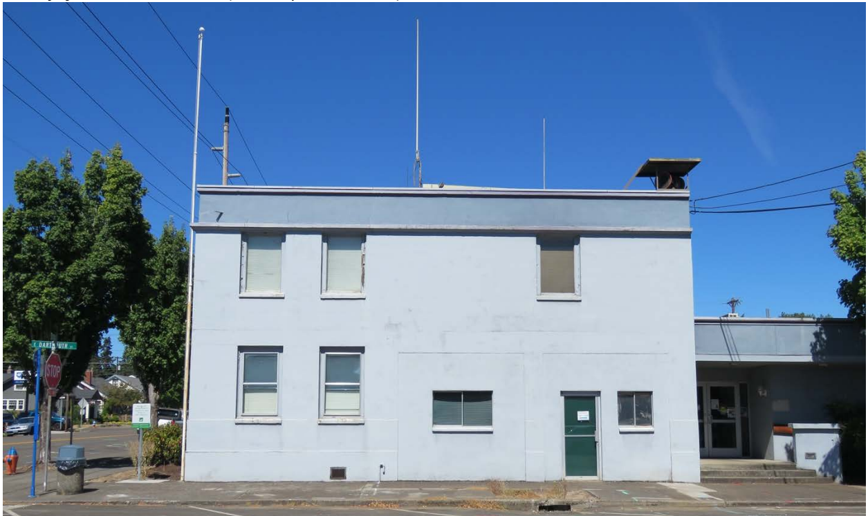
Western portion of south façade showing infilled garage doors, view northwest (ARG, September 2020).
