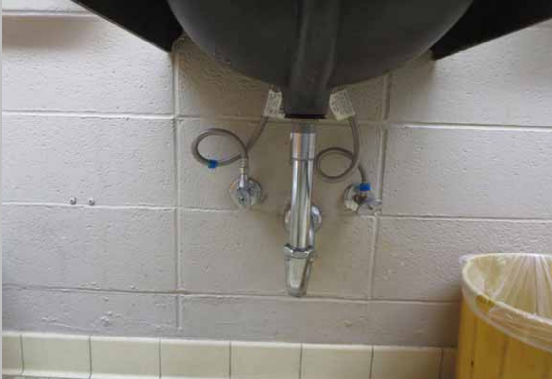
Install scald and abrasion protection at noted locations (Critical Repair)
