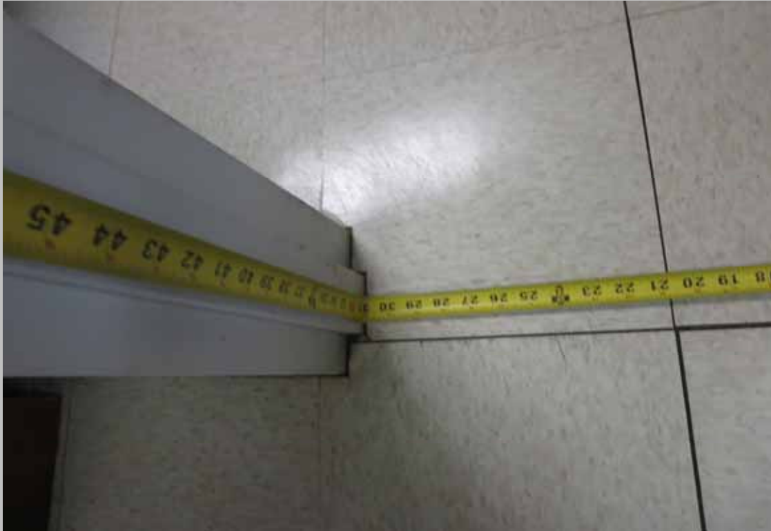
Widen door openings at noted locations (Critical Repair)
