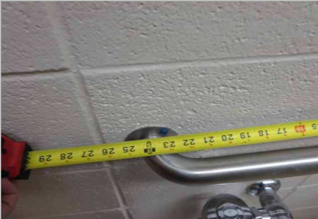
Install 36 inch rear grab bar at women's common restroom toilet (Critical Repair)
