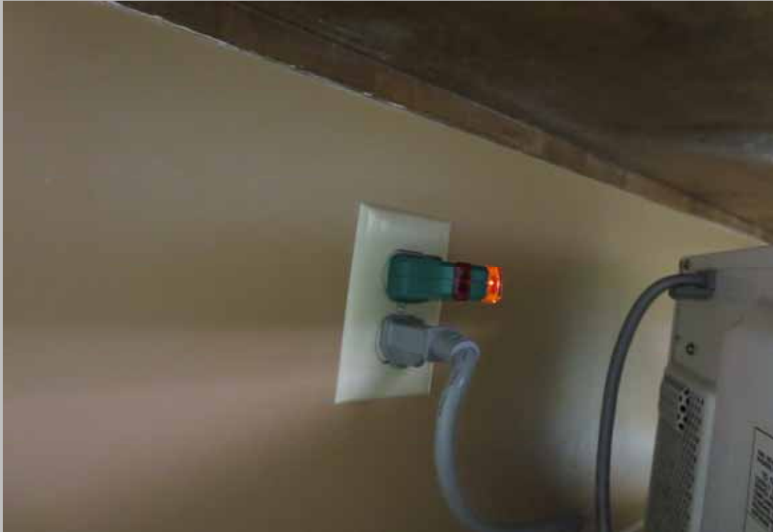
Install GFCI protected outlets at noted locations (Critical Repair)
