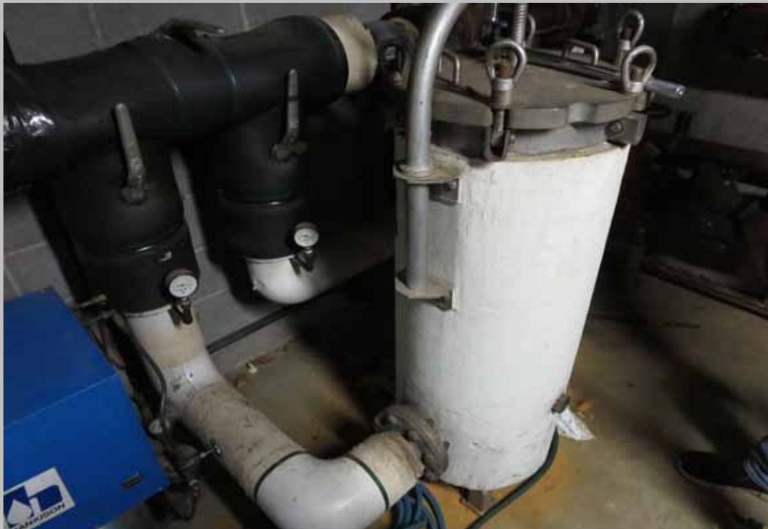
Water filtration equipment
