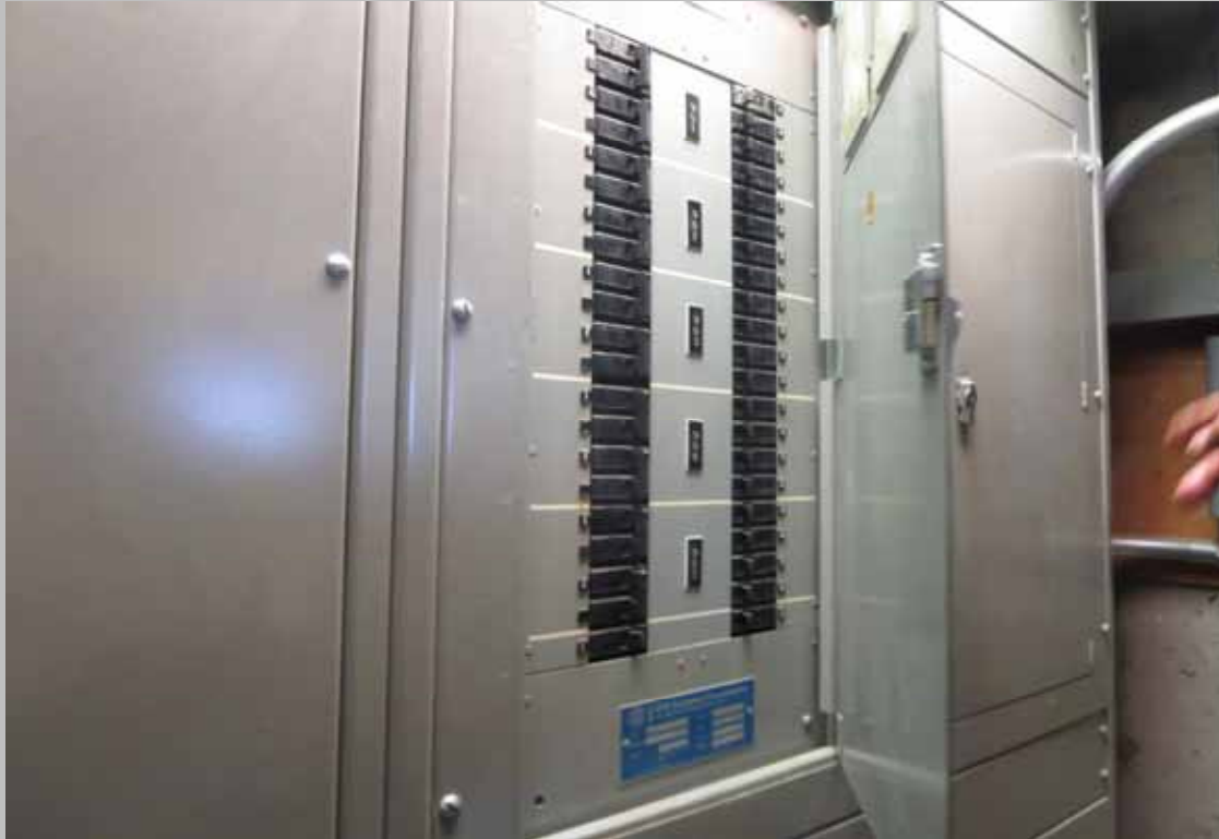
Electrical main distribution
