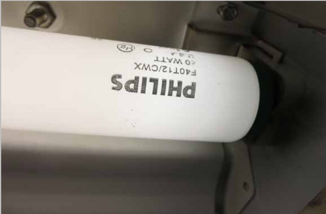
Replace inefficient fluorescent fixtures (Non-Critical Repair)
