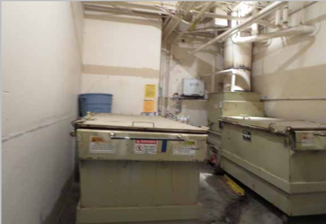
Trash compactor and dumpster
