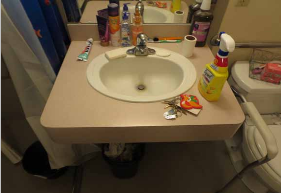
Replace dwelling unit bathroom counters (Non-Critical Repair)
