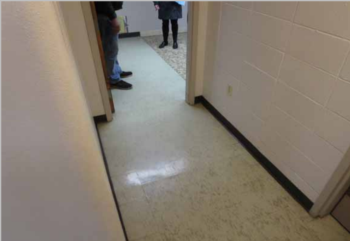
Replace common areas VCT flooring (Non-Critical Repair)
