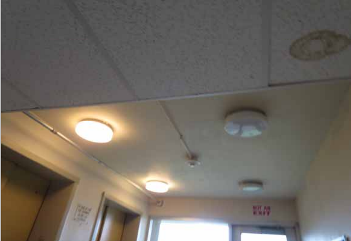
Replace inefficient incandescent fixtures (Non-Critical Repair)
