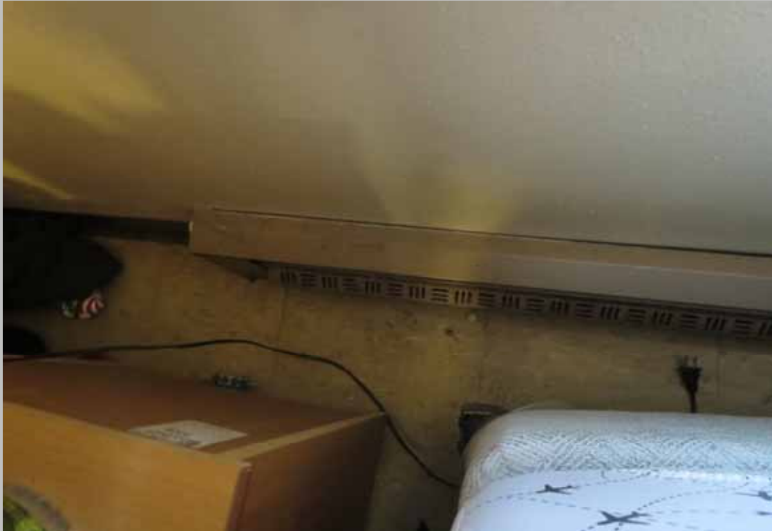
Dwelling unit baseboard heater
