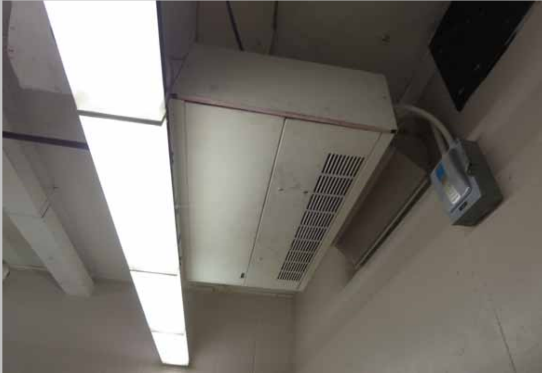
Air handler unit
