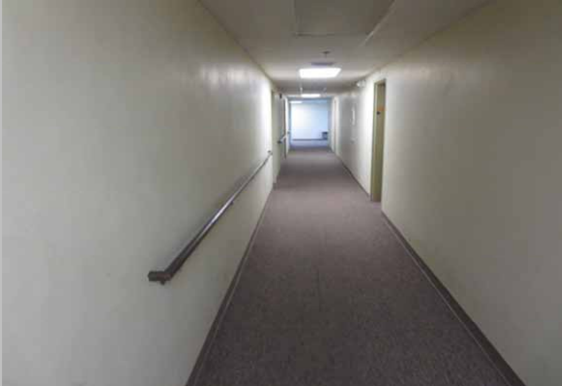
Replace common area carpeting (Non-Critical Repair)
