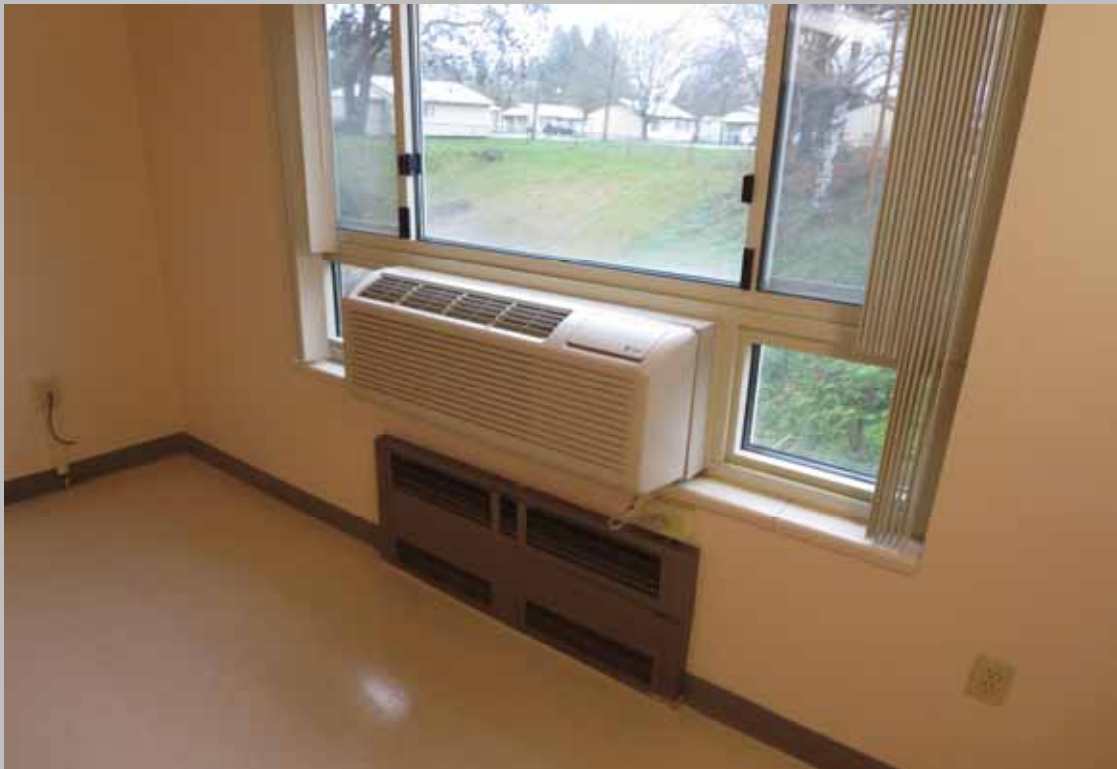
Dwelling unit PTAC
