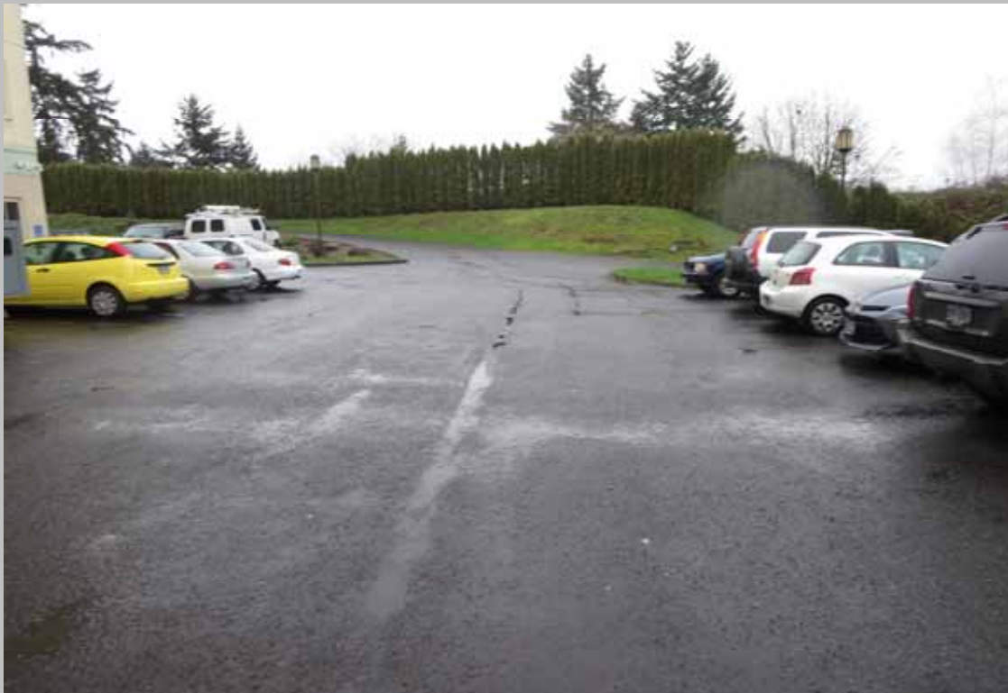
Seal coat parking areas (Non-Critical Repair)
