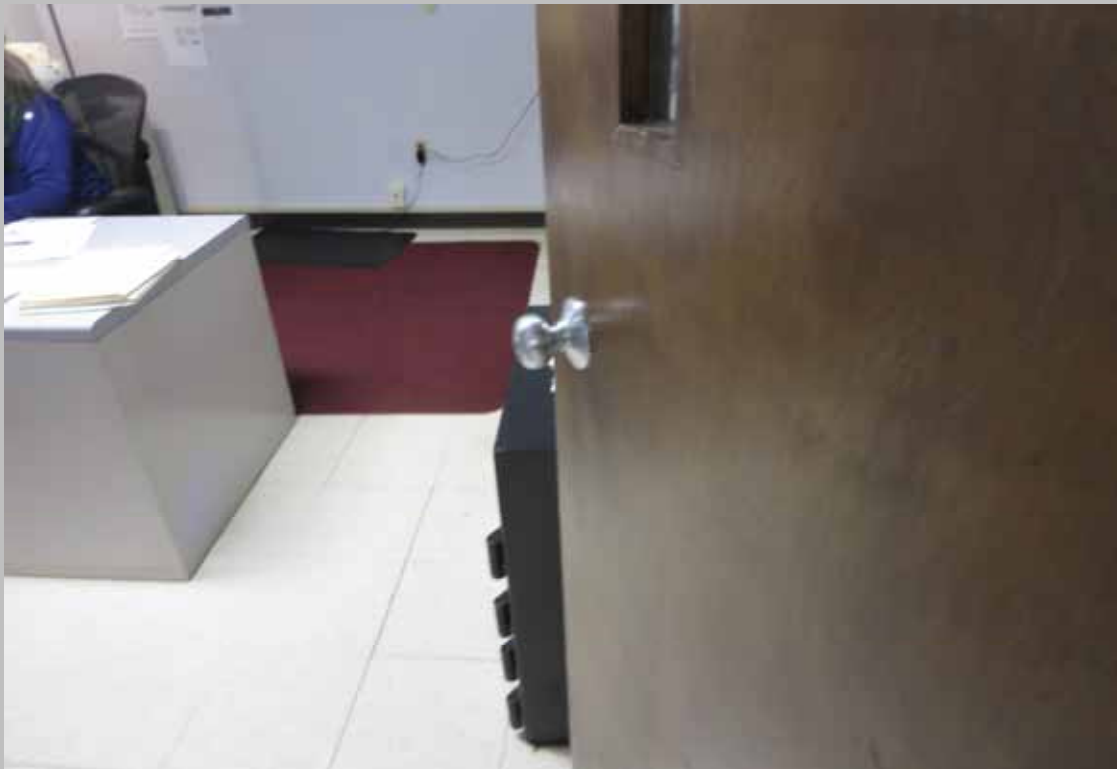
Install levered handle door hardware at noted locations (Critical Repair)
