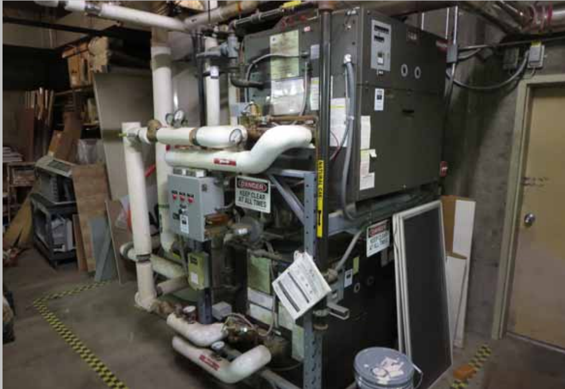
Domestic hot water boilers
