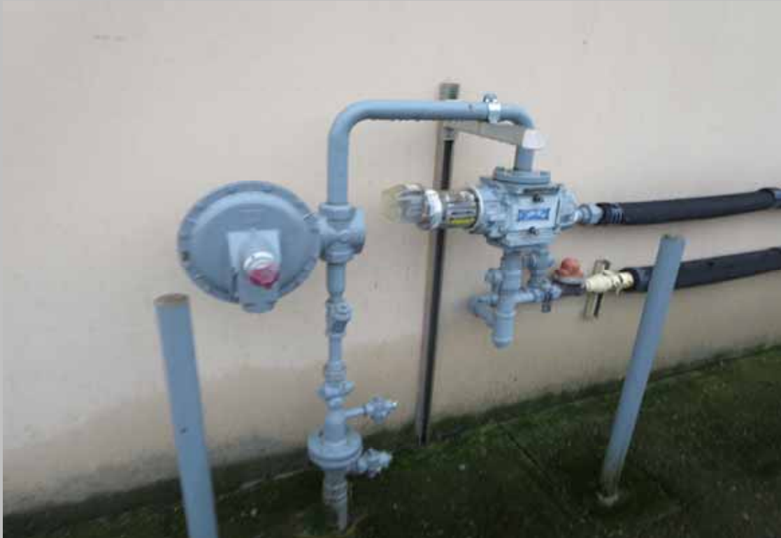
Natural gas riser
