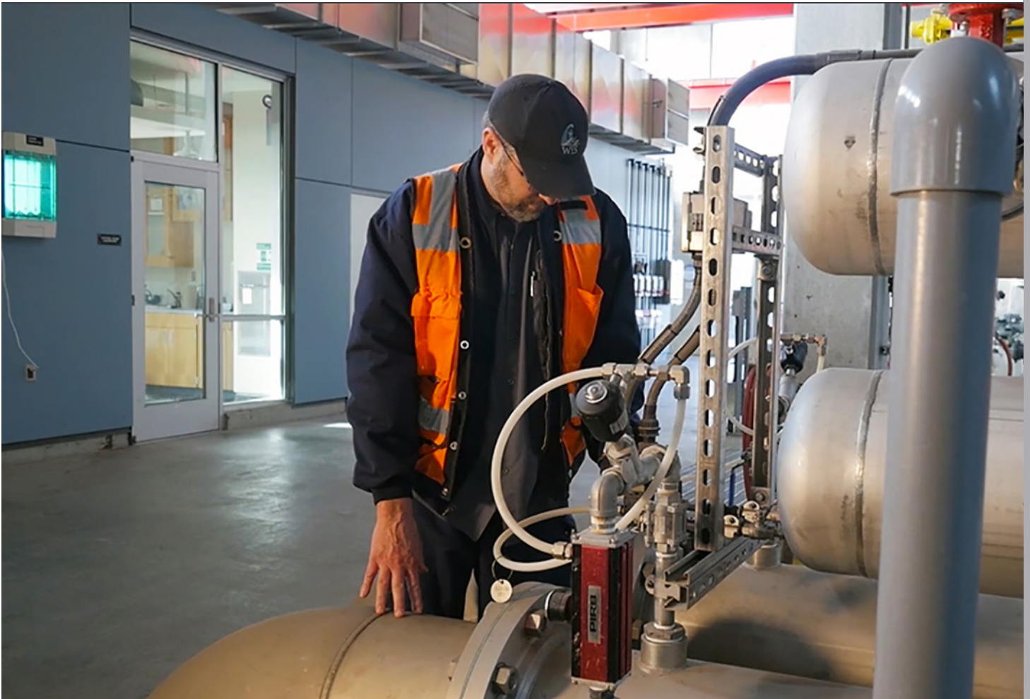
Tri-City Water Resource Recovery Facility
