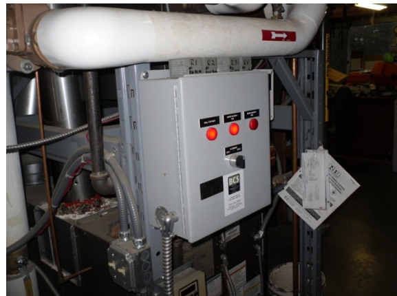
Photo #34: Water heater control panel
