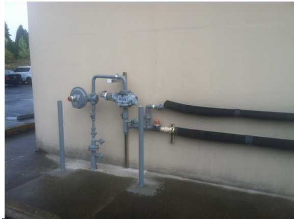
Photo #32: Gas meter
