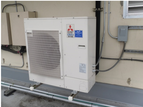
Photo #45: Split Air Conditioner unit
