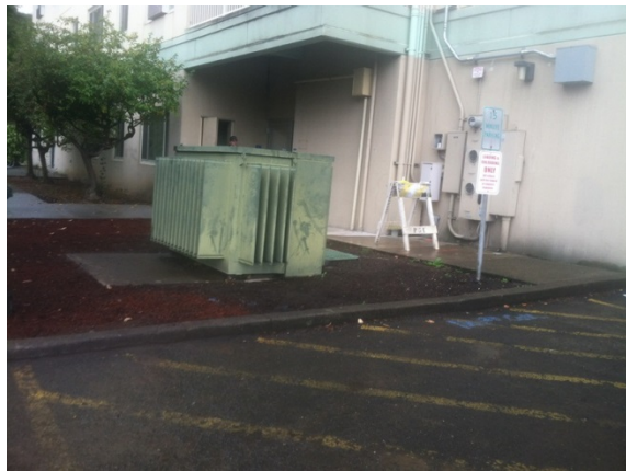
Photo #35: Main transformer
