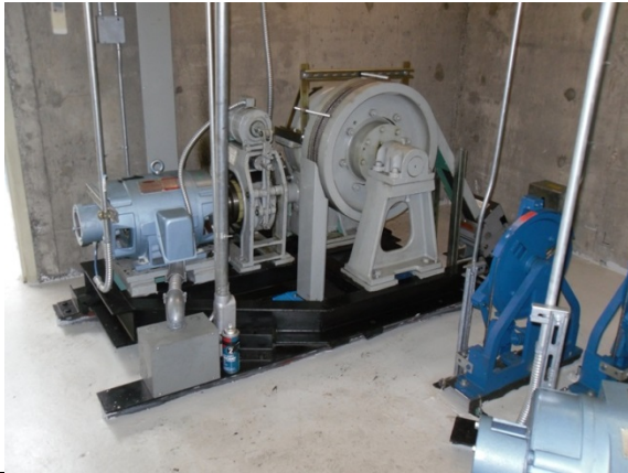
Photo #43: Elevator equipment
