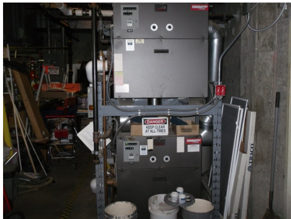
Photo #33: Water heaters
