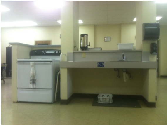
Photo #15: Common area kitchen equipment
