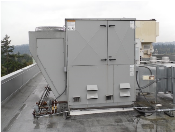
Photo #41: Package unit
