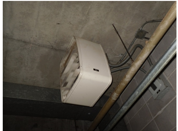
Photo #42: Space heater
