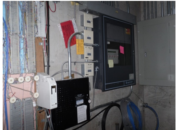
Photo #40: Fire alarm
