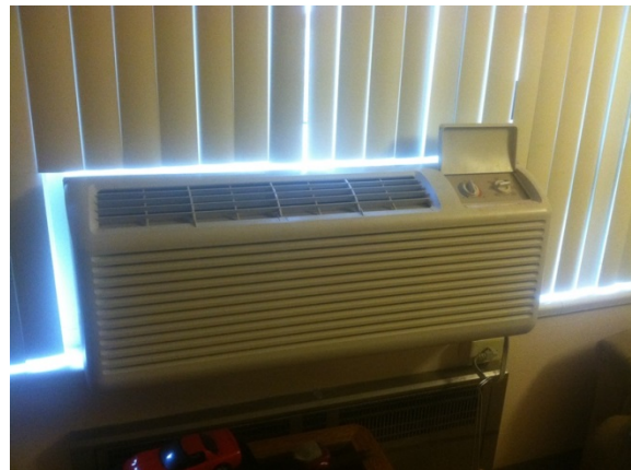
Photo #36: Typical PTAC at apartment unit
