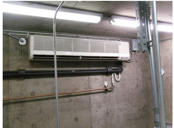
Photo #46: Split Air Conditioner unit
