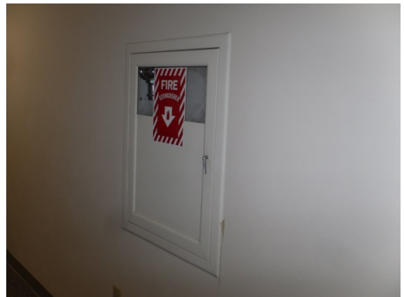
Photo #48: Fire protection equipment
