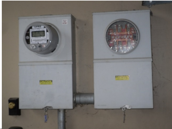
Photo #31: Electrical meter
