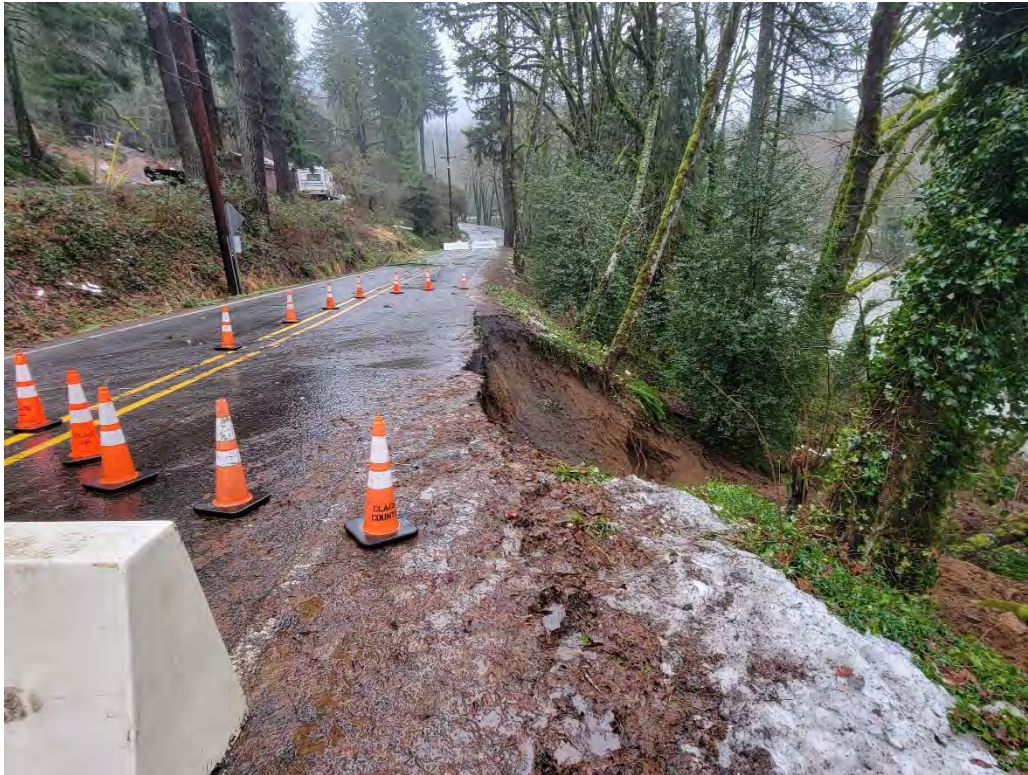
A: View looking East at landslide encroaching outboard lane. (East Barlow Trail Road)
