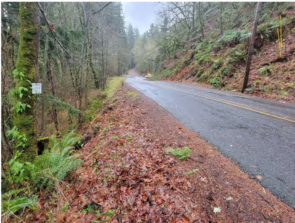
B: View looking east at western extent of cracked pavement and subsidence in background. (SE Bull Run Road between SE Ten Eyck and SE Phelps Roads)
