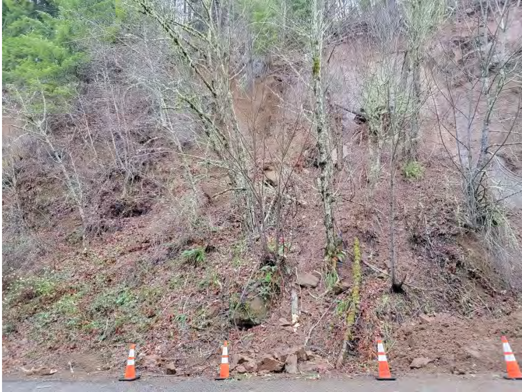
A: View looking north at rock debris retained on slope and potential hazard trees. (SE Bull Run Road near SE Laughing Water Road)
