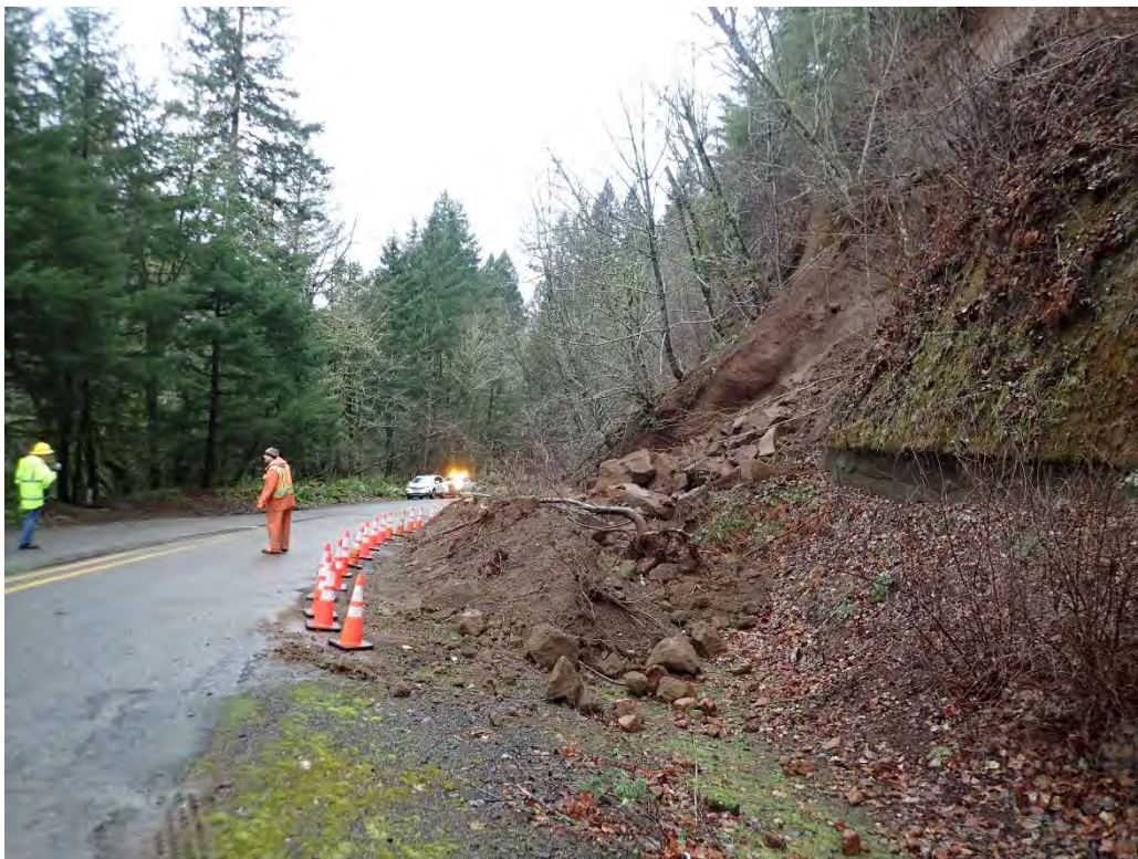
B: View looking northwest at slide debris in ditch, and the approximate original location of maximum block size as noted by person in the inboard travel lane. (SE Bull Run Road near SE Laughing Water Road)
