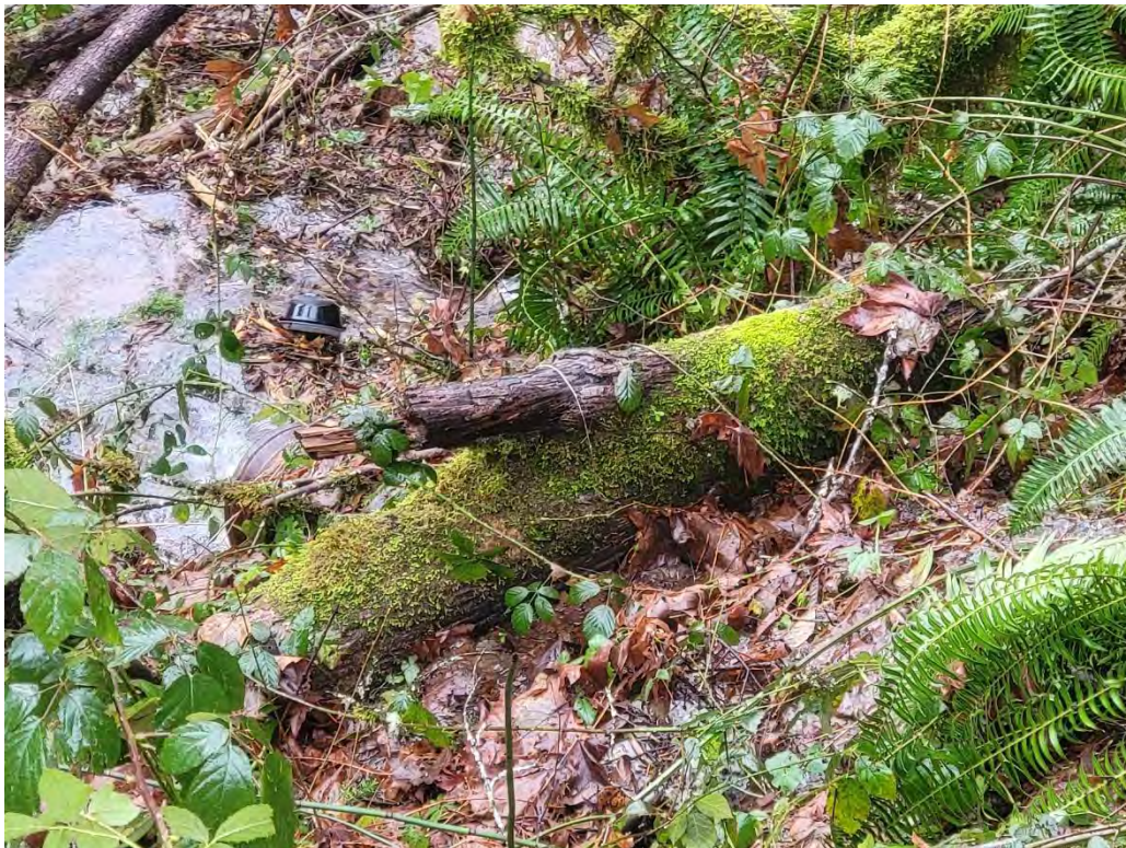
B: Zoomed in view of discharge from culvert east of the landslide. Note water flowing out of embankment above culvert outlet as well as the outlet. (East Barlow Trail Road)
