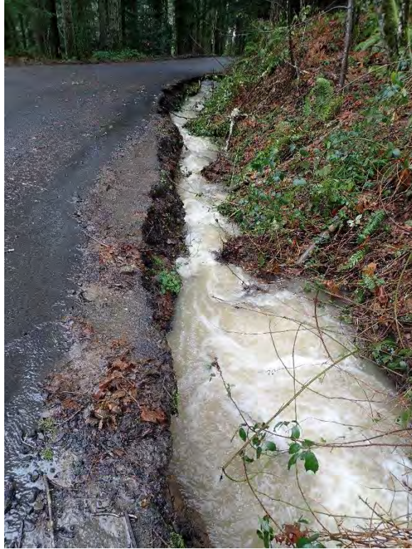
A: View of discharge flowing in unlined ditch along E Boulder Creek Lane, towards North Boulder Creek, located above E Barlow Trail Road. (East Barlow Trail Road)
