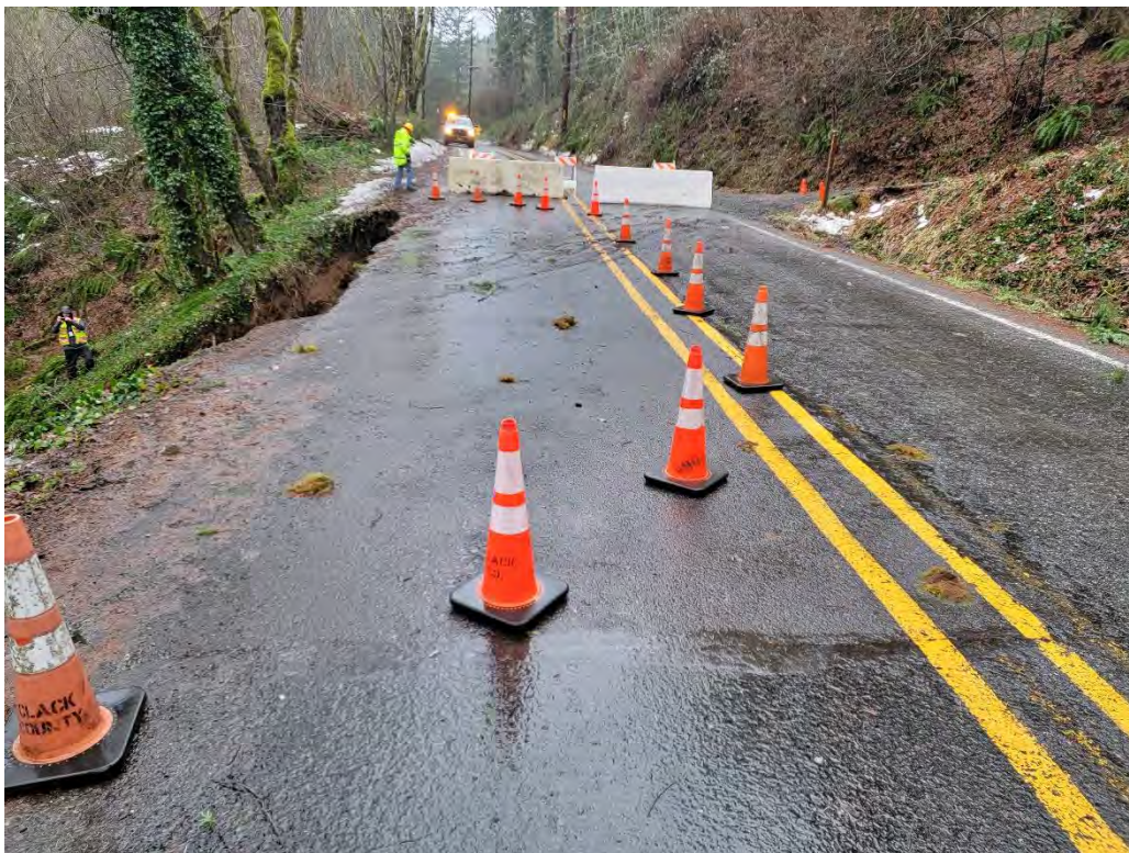
B: View looking west at landslide encroaching outboard lane. (East Barlow Trail Road)
