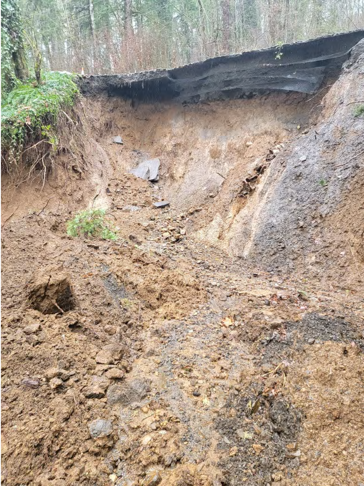
View looking northwest at headscarp and undermined road. (East Barlow Trail Road)
