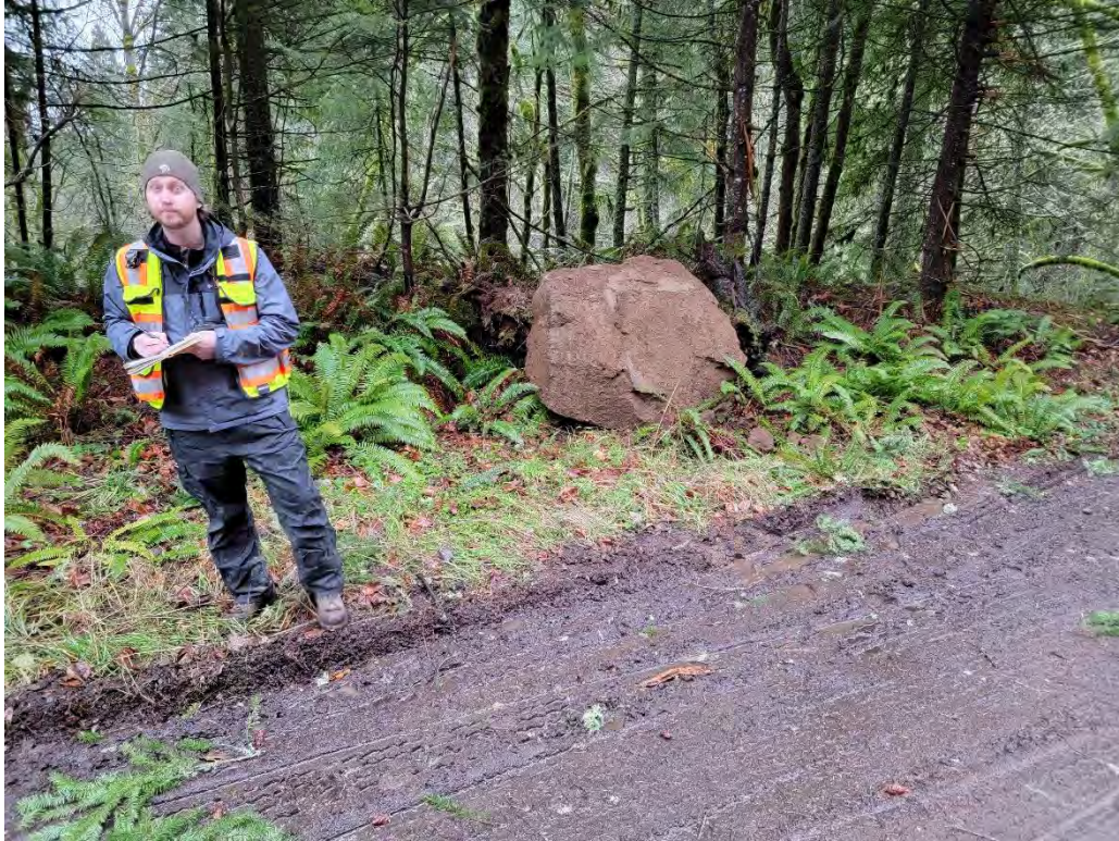
A: Maximum rock block observed approximately 6'x4'x2'. (SE Bull Run Road near SE Laughing Water Road)
