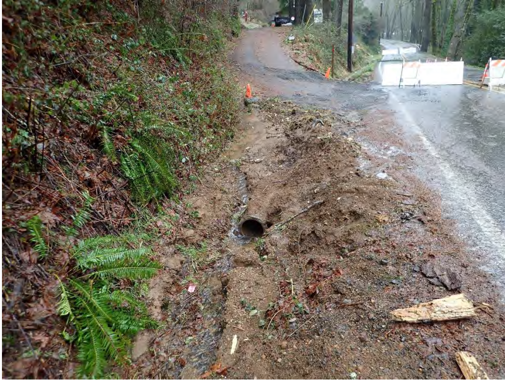
A: View looking east at inboard ditch culvert inlet, upslope of landslide. (East Barlow Trail Road)
