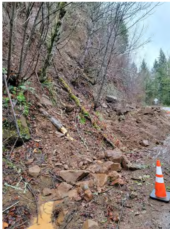
B: View looking southeast at debris and ponded water retained in ditch line. (SE Bull Run Road near SE Laughing Water Road)
