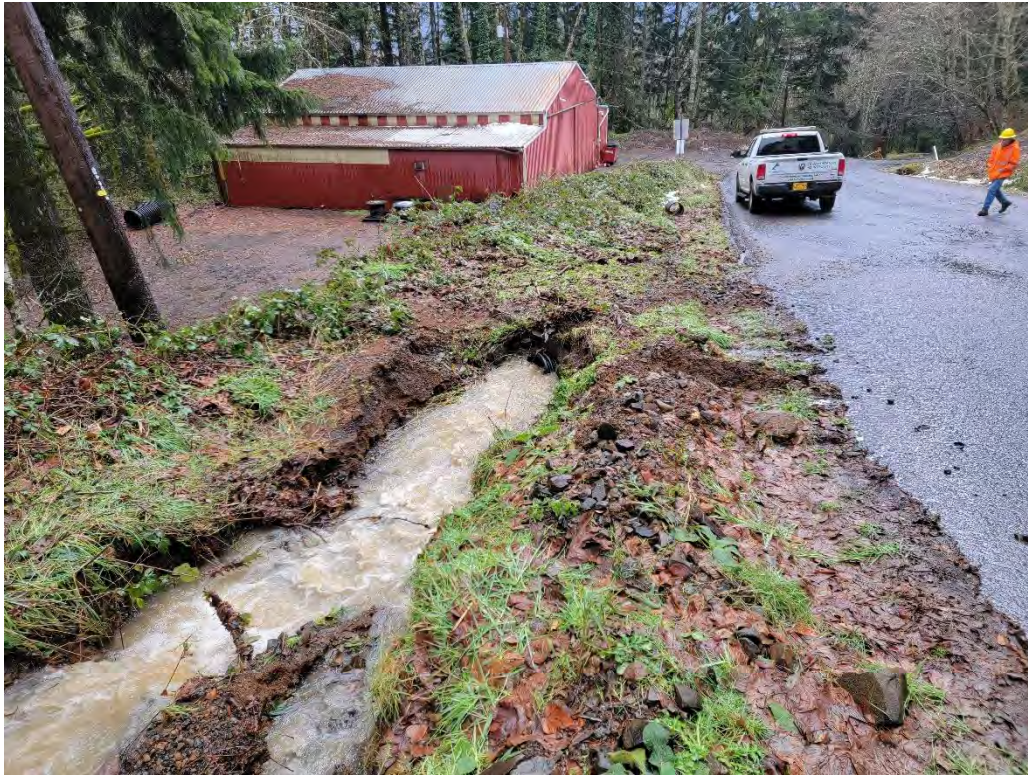
A: View of culvert leading from catchment to settlement pond, reported clogged with debris during landslide. (East Barlow Trail Road)
