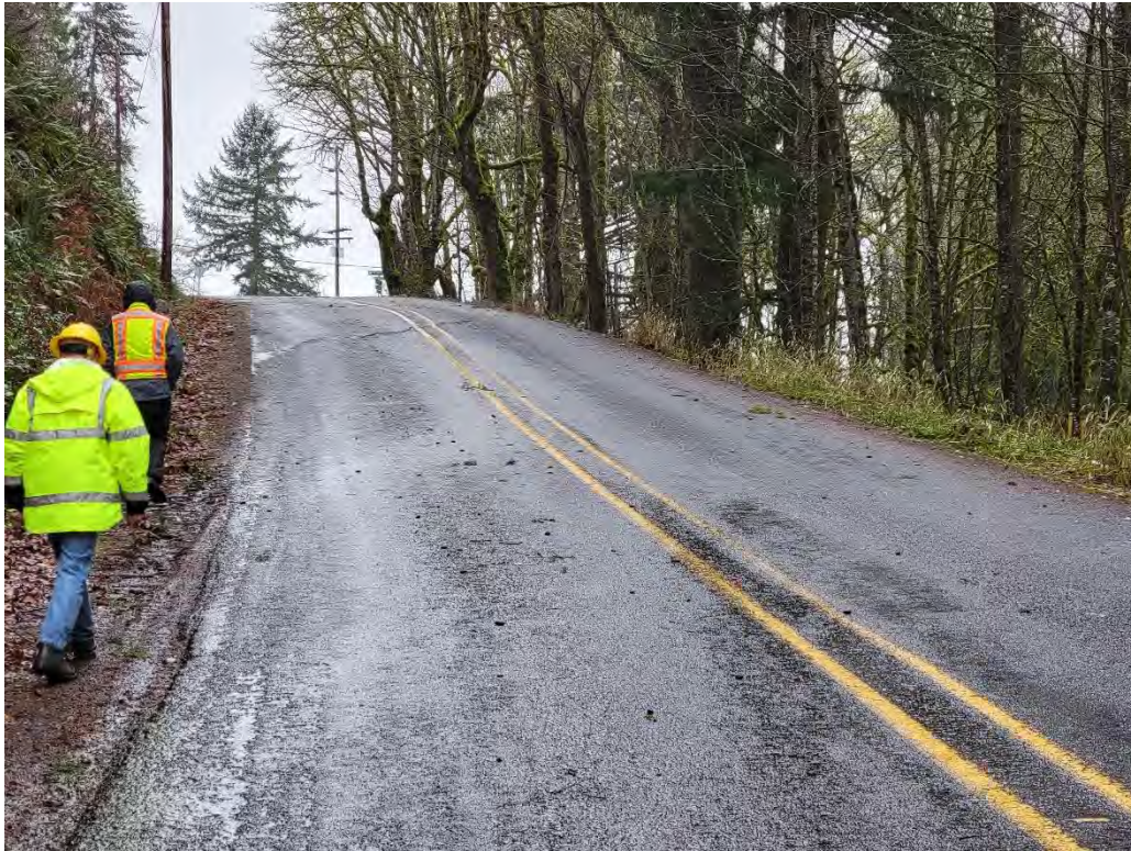
A: View looking west at crack in pavement and subsidence of road. Downtrop is towards foreground. (SE Bull Run Road between SE Ten Eyck and SE Phelps Roads)
