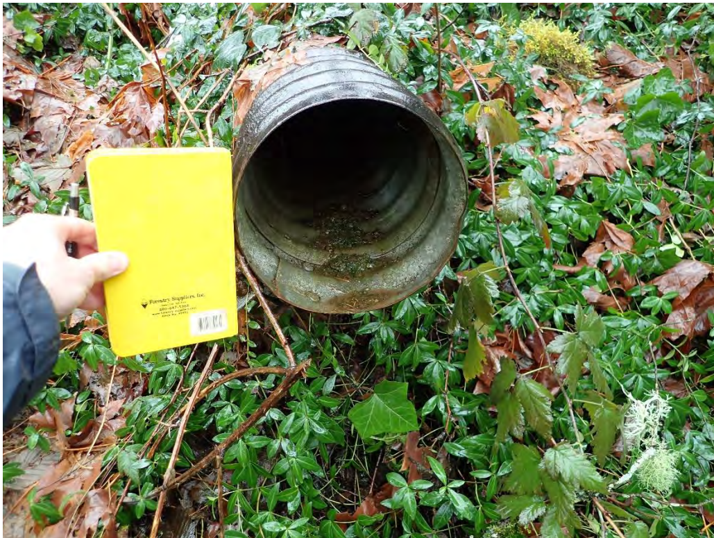
B: View of outlet of blocked culvert underneath road, west of landslide. (East Barlow Trail Road)
