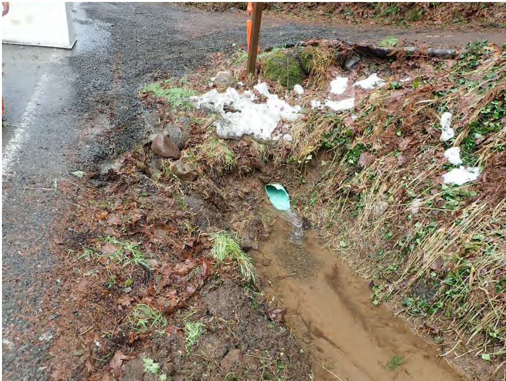
B: View looking west at inboard ditch culvert outlet, upslope of landslide. Note different culvert material from inlet side. (East Barlow Trail Road)
