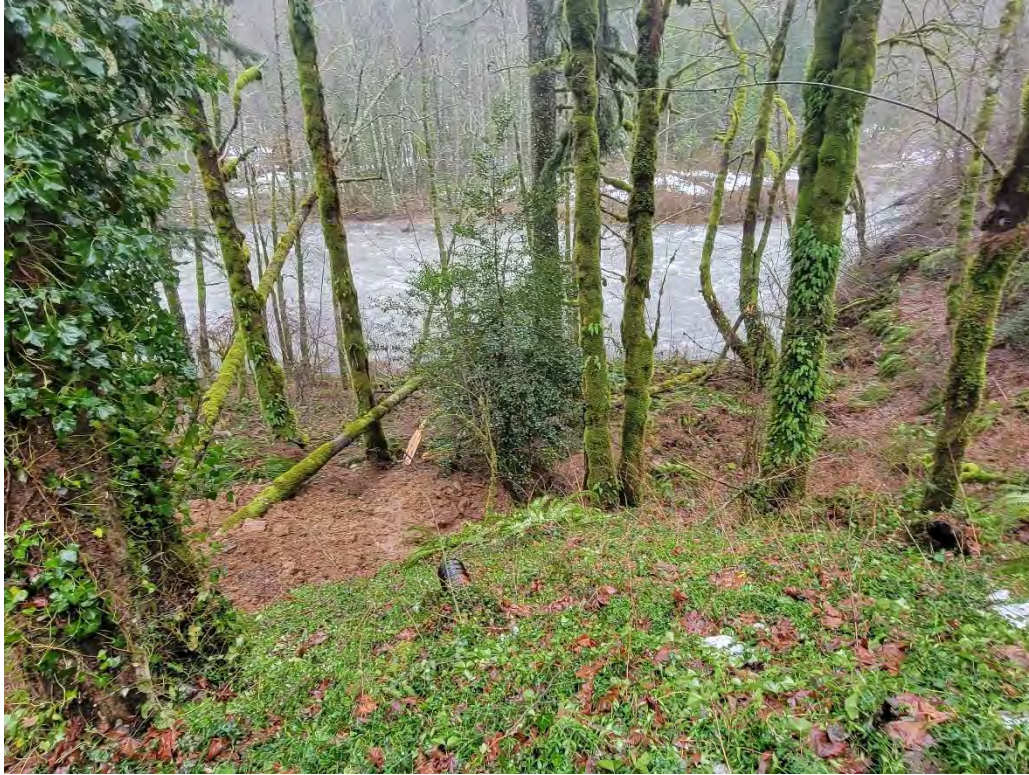
A: View looking south at blocked culvert running underneath road, upslope of landslide. (East Barlow Trail Road)
