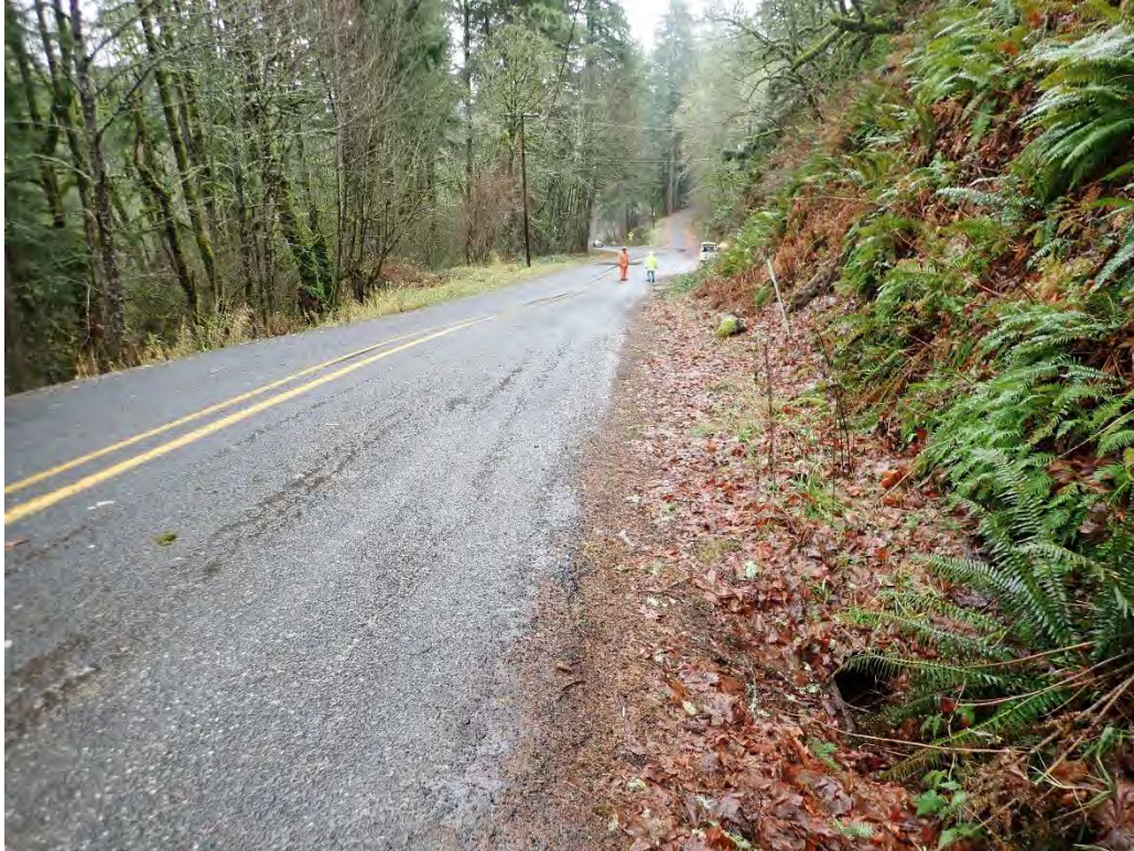
A: View looking east along inboard ditch line and culvert entrance. (SE Bull Run Road between SE Ten Eyck and SE Phelps Roads)
