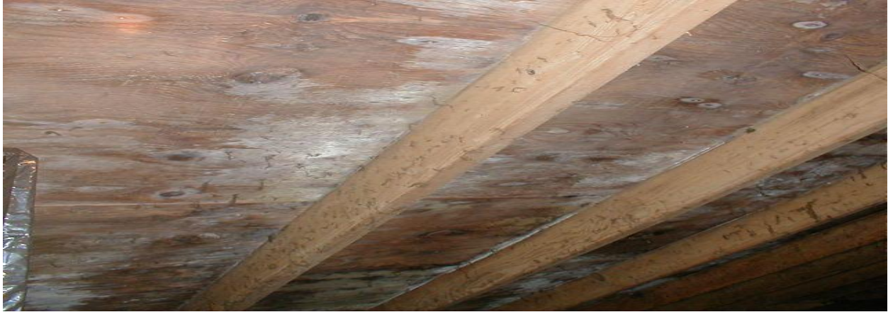
Figure 8. Condensation: Mold growing on roof "sheathing" in an attic. In winter months, moisture (water vapor) leaking through the ceiling of the living area with the force of warm air rising will condense on the cold attic sheathing, causing property damage and mold exposure to occupants. Left uncorrected, the roof will fail and need replacement.
