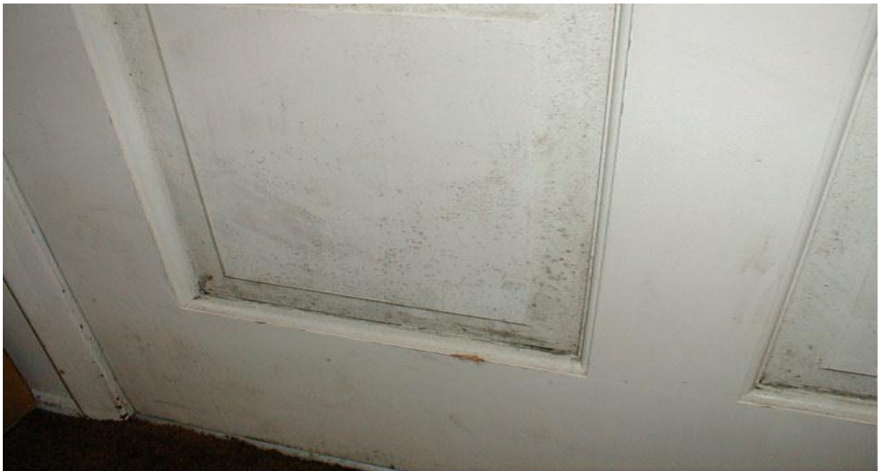
Figure 6. Condensation: Mold growth on inside surface of exterior door. Again, cold surface meets moist air, gets wet and supports mold growth. This can be washed off and repainted.
