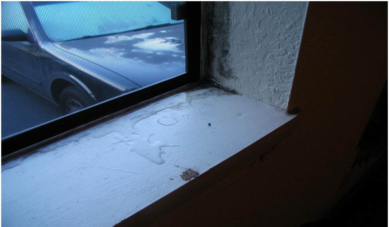
Figure 1. Condensation from excessive indoor moisture on the window glass drained and ponded on the window sill, soaked into and wicked up the drywall, and provided plenty of moisture to cause the black mold growth visible next to the window.
