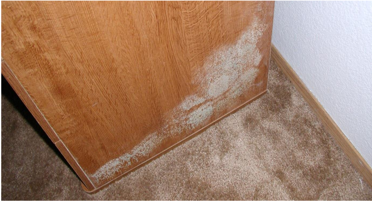
Figure 3. Mold growth caused by condensation on the cool cabinet placed against an exterior wall in a rental unit. The excessive indoor relative humidity (regularly exceeding 60%) was the culprit. This surface can be cleaned with soapy water.
