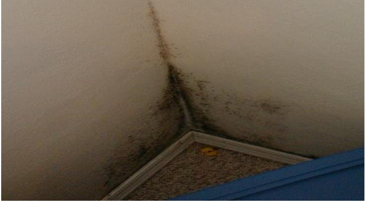
Figure 5. Condensation: Mold growth in bedroom corner of exterior wall. The combination of high relative humidity from occupants breathing all night (exhaling water vapor) and the cool surfaces of the exterior wall led to condensation and mold growth.
