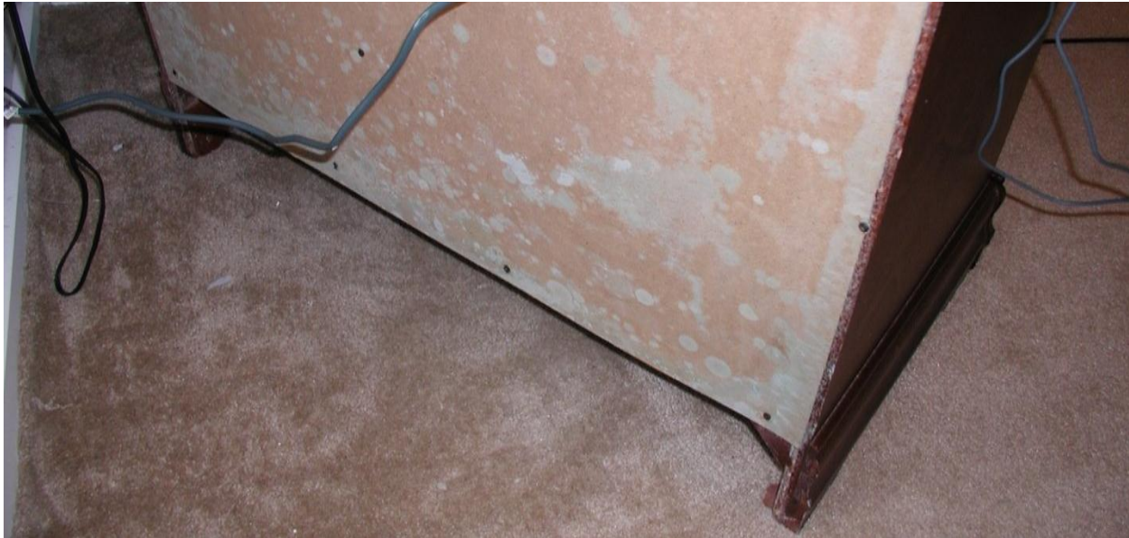
Figure 4. Condensation: Tenants kept the apartment at 60 degrees, cold enough that the back side of their dresser was below “dew point”, the temperature at which typical moisture levels in the air will condense on a surface. With the dresser chronically wet, mold got started and amplified. This can probably be scrubbed off (outside!) and painted. To prevent a recurrence of the mold, surfaces need to be kept warmer either by increasing the apartment temperature and/or allowing air circulation behind the dresser, or lowering the relative humidity in this space.
