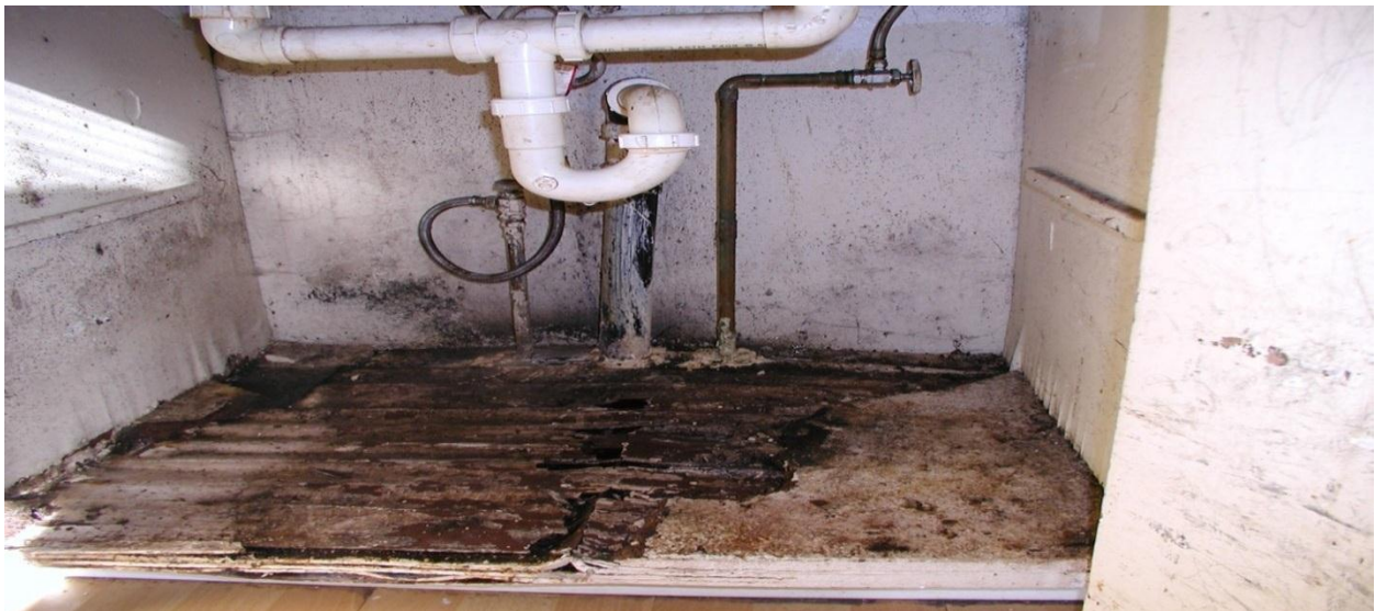
Figure 9. Plumbing leak: Prompt communication with a landlord could have prevented this damage.
