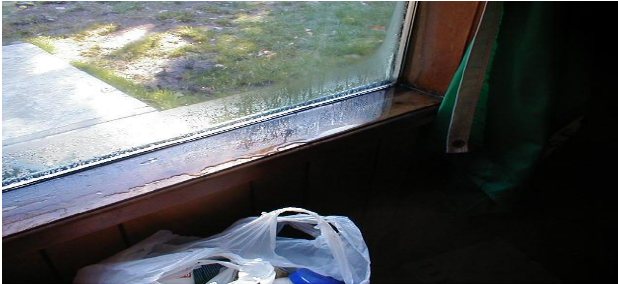
Figure 2. Too much moisture in the air (high relative humidity) leads to unwanted condensation on cool surfaces like double pane windows in cold weather. The moisture drips down, accumulates on sills, and can leak into wall cavities below causing hidden mold growth on wood and paper backed wallboard. Single pane windows will be colder still, resulting in condensation even with normal indoor humidity levels (below 40%) and may require daily drying of sills with towels to prevent mold growth and water damage.
