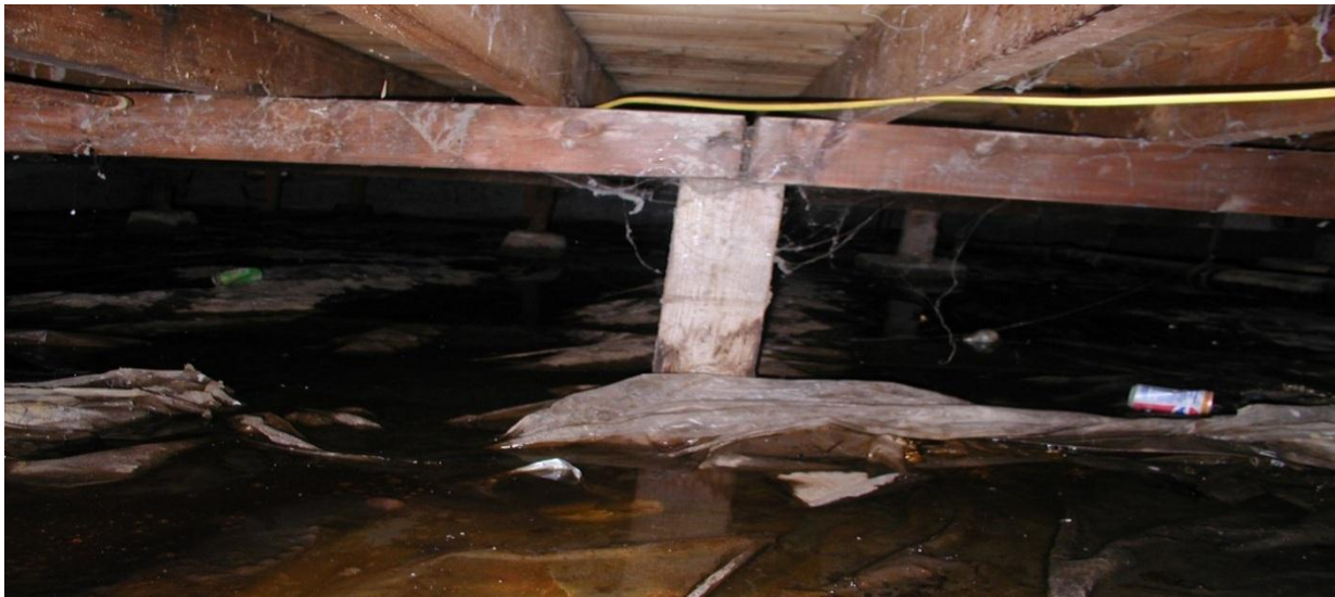
Figure 7. Standing water in a crawlspace: 40 percent of the air you breathe can come from the crawlspace, pulled up by the force of warm air rising. Excess crawlspace moisture is bad for your health, bad for the structure, and a significant factor driving relative humidity UP upstairs.
