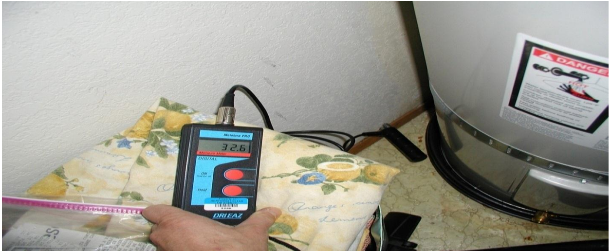
Figure 11. Plumbing leak: Hot water tank leaked and was replaced, but wallboard is still sopping wet (meter says 32.6; 28 is very wet) and mold will grow. This is where a moisture meter comes in very handy; finding damp materials adjacent to a leak before mold grows saves time and money for landlords...the meter may well “pay for itself.” This wet drywall, IF it can be saved, needs to be opened and aggressively dried using professional dehumidification techniques.
