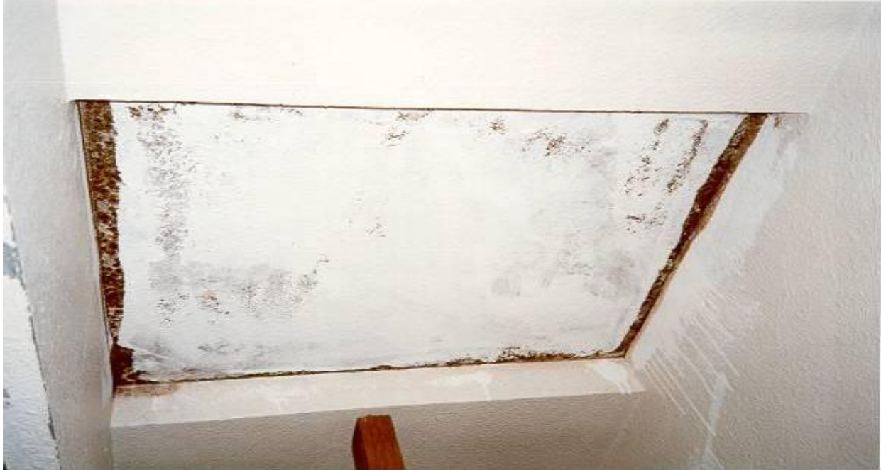
Figure 13. Drywall covered with mold needs to be carefully removed. Painting over mold is not acceptable work practice.
