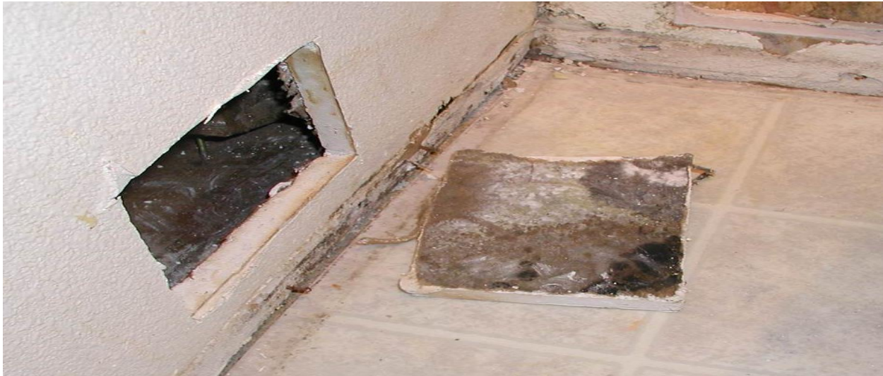
Figure 12. Saturated wallboard must be aggressively dried or mold WILL grow, often on the hidden paper backside of the wallboard in the wall cavity. This moldy wallboard should be carefully abated using a negative pressure enclosure and respiratory protection for workers.
