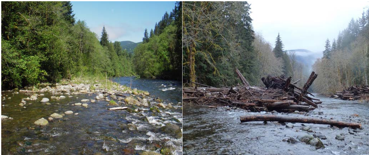
Before (left) and after (right) of Salmon River with completed wood jam structure.
