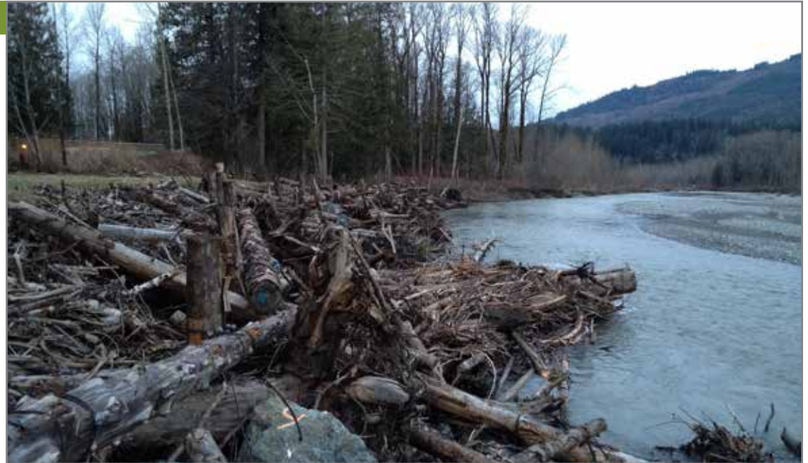
Figure 21. An engineered large wood revetment built by the Lummi Nation created a rough streambank very different than traditional rock revetments found along Sandy River. The structure along the South Fork Nooksack River in northwest Washington is stabilized with timber piles and rock collars.
