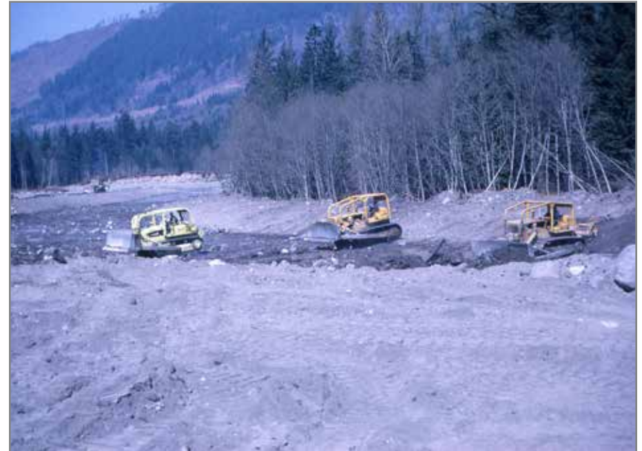
Figure 13. The the U.S. Army Corps of Engineers moved an astounding amount of flood debris in response to the December 1964 flood, here they are re-building the pre-flood channel, confining miles of the Sandy between levees, and stripping off streamside vegetation. Note the fine grained material of sand and gravel. The wide expansion of the river channel and its floodplain that occurred in the 1964 flood left behind large deposits of fine grained material not found in segments of the river that are constrained. The finer substrate not only reflects a less erosive river, but is much more beneficial to salmon. Where the river is allowed to migrate and widen its floodplain, it will create a more sinuous and multi-thread channel that is more effective at dissipating energy and creating more desirable fish and wildlife habitat. (Photo courtesy of the Arrigotti family and Clackamas County)
