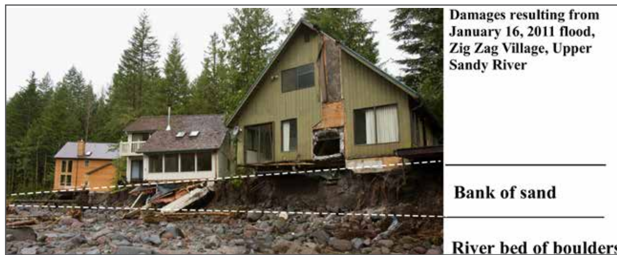
Figure 8. Home damage along the Upper Sandy River due to bank erosion. Note the bank is primarily composed of easily erodible sand whereas the river bed consists primarily of boulders. Photo: The Oregonian.
