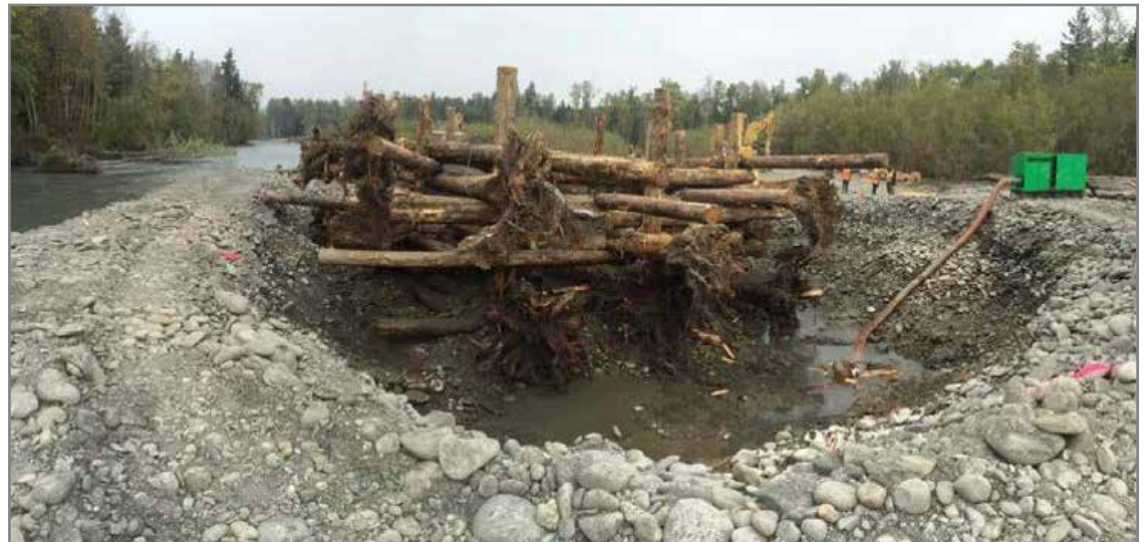
Figure 22. Example of engineered logjam that doesn't have self-settling elements of previous examples. This structure is deeply embedded into the river so that it can withstand scour without being compromised. Note people on right side of the structure. Pit is 16 feet deep and timber posts extend deeper. Elwha River 2014.
