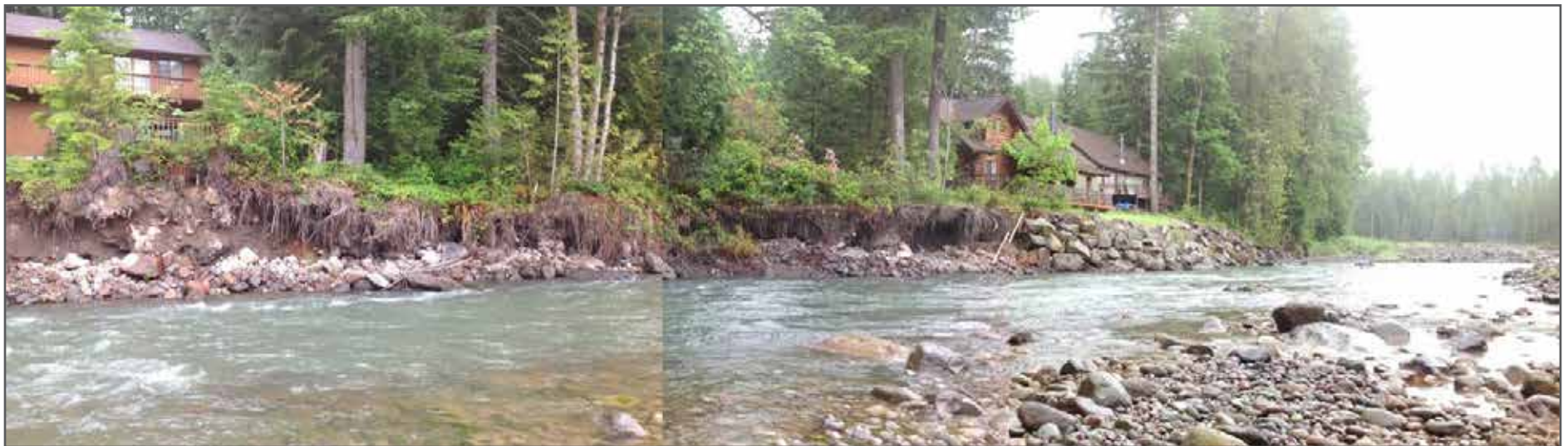
Figure 14. Tree roots can help stabilize banks by adding cohesion, but only to depths of about three feet and thus can be undercut along high banks. A traditional rock revetment (Sandy RM 39.5) is visible in the right background. The relatively smooth surface of these types of traditional bank stabilization structures can intensify erosive energy along natural banks, creating a condition where the structure can accelerate its own demise. Revetments such as this one temporarily slowed river's natural expansion toward its pre-floodplain prior to the Old Maid mudflows. The wider the floodplain, the more the river's erosive power is reduced. Allowing the river space to move and create new floodplain not only reduces flood and erosion risk, but enhances salmon habitat.
