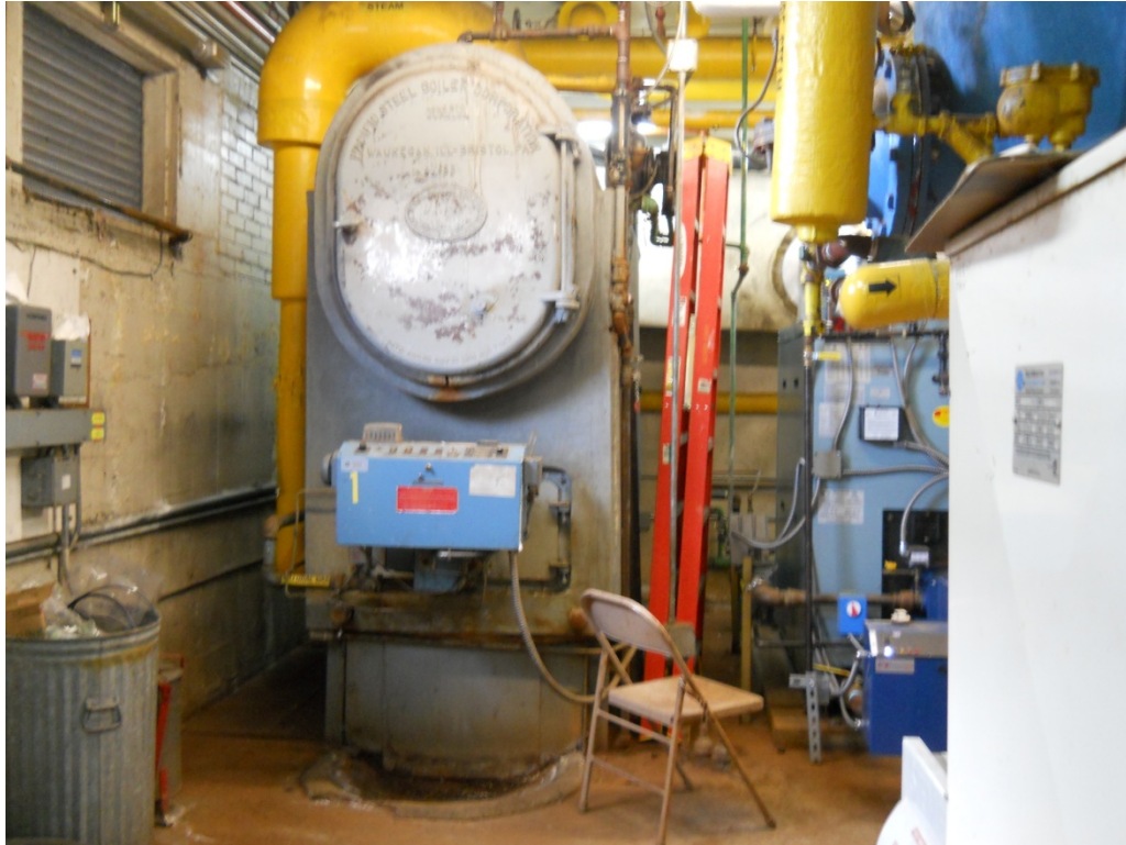
PHOTO 21: Old boiler system located next to the current natural gas furnace system
