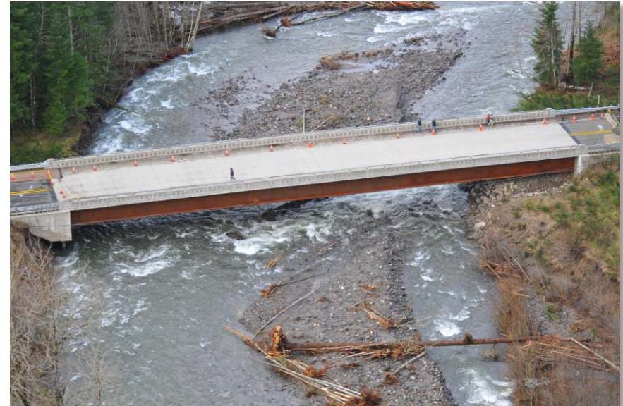
Above: Zigzag River Bridge carrying E Lolo Pass Road across the Zigzag River. Photo taken during 2011 flood damage repair work.
