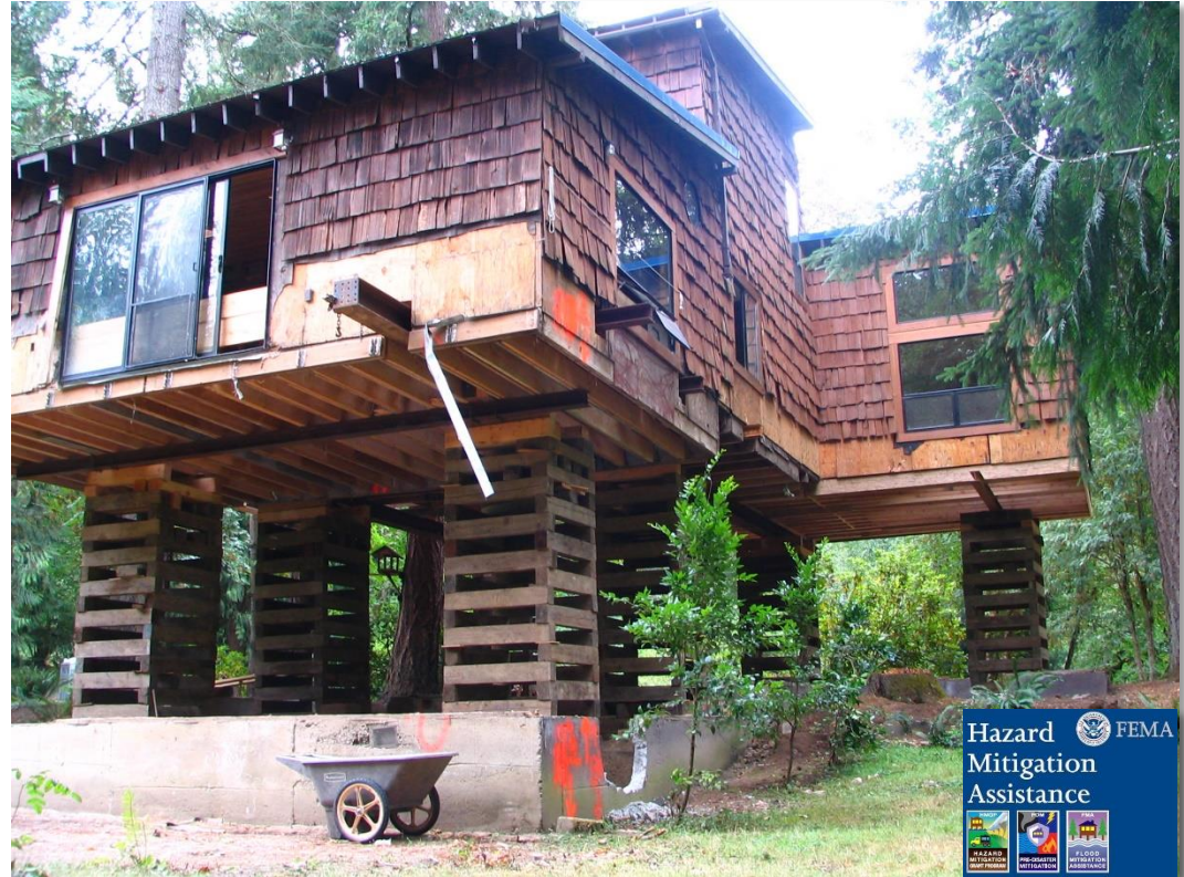
Above: Flood-damaged home along Abernethy Creek undergoing process of being elevated through FEMA Hazard Mitigation Grant funds.
