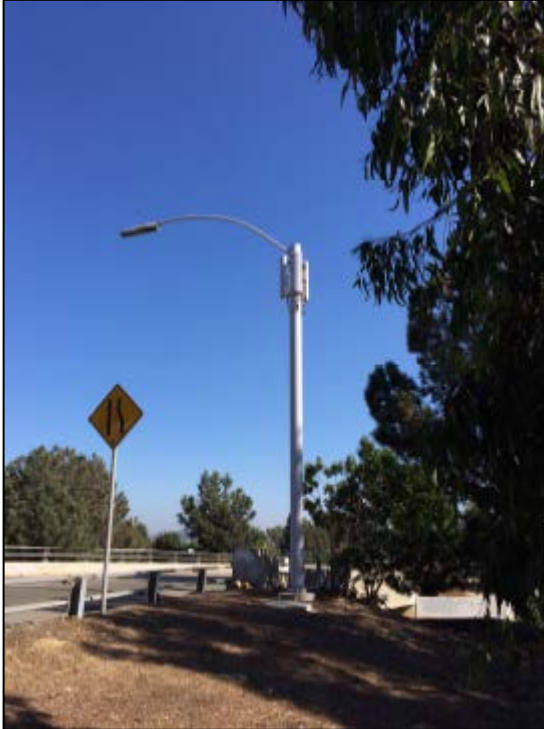
Figure 27: This right-of-way installation has three antennas mounted flush to the pole with no pipe mounts and no antenna shroud. This is an older installation with no chin covers; they are now required.
