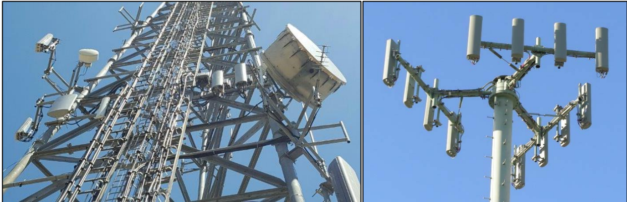
Figure 33: Lattice towers and monopoles don't integrate. They do not meet the requirements of the Wireless Ordinance.
