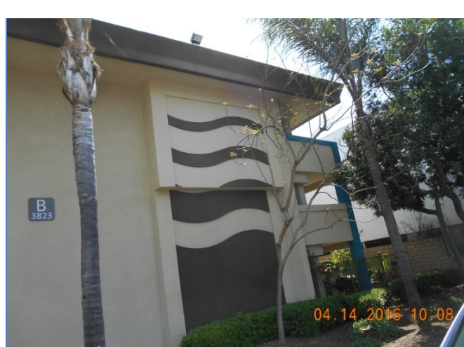
Figure 15: Although façade-mounted boxes are not preferred, this is still an excellent example of integration.
