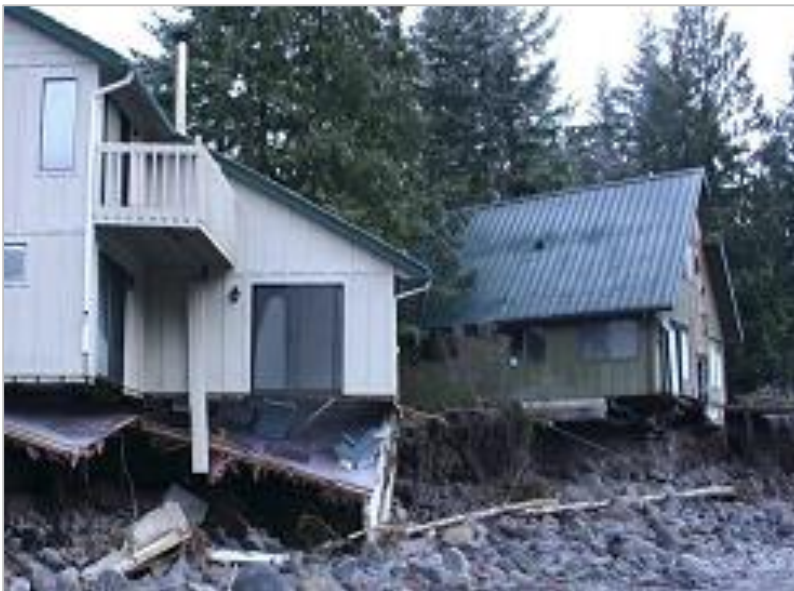
Figure 4-1: Residencies Damaged by Flooding and Erosion
