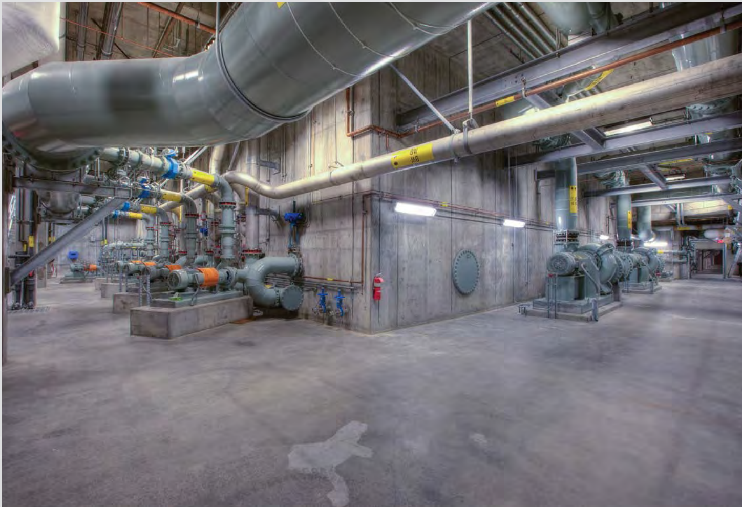
Membrane Bioreactor Process Gallery at Tri-City Water Resource Recovery Facility in Oregon City, OR
