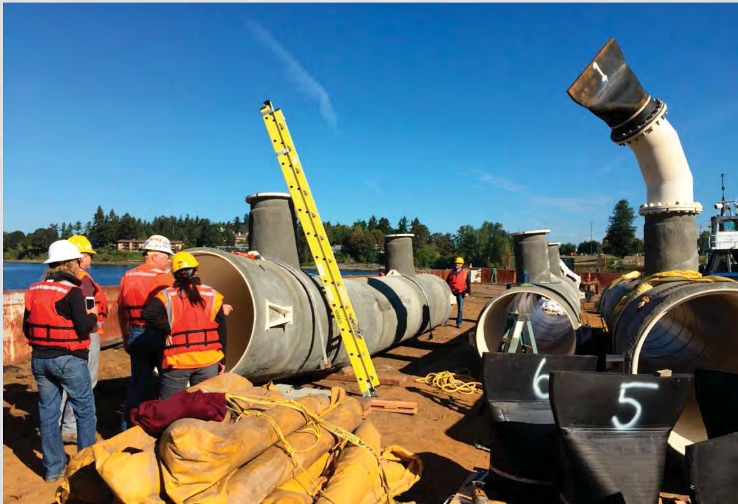
Crews work on replacing the outfall pipe at Kellogg Water Resource Recovery Facility in Milwaukie, OR
