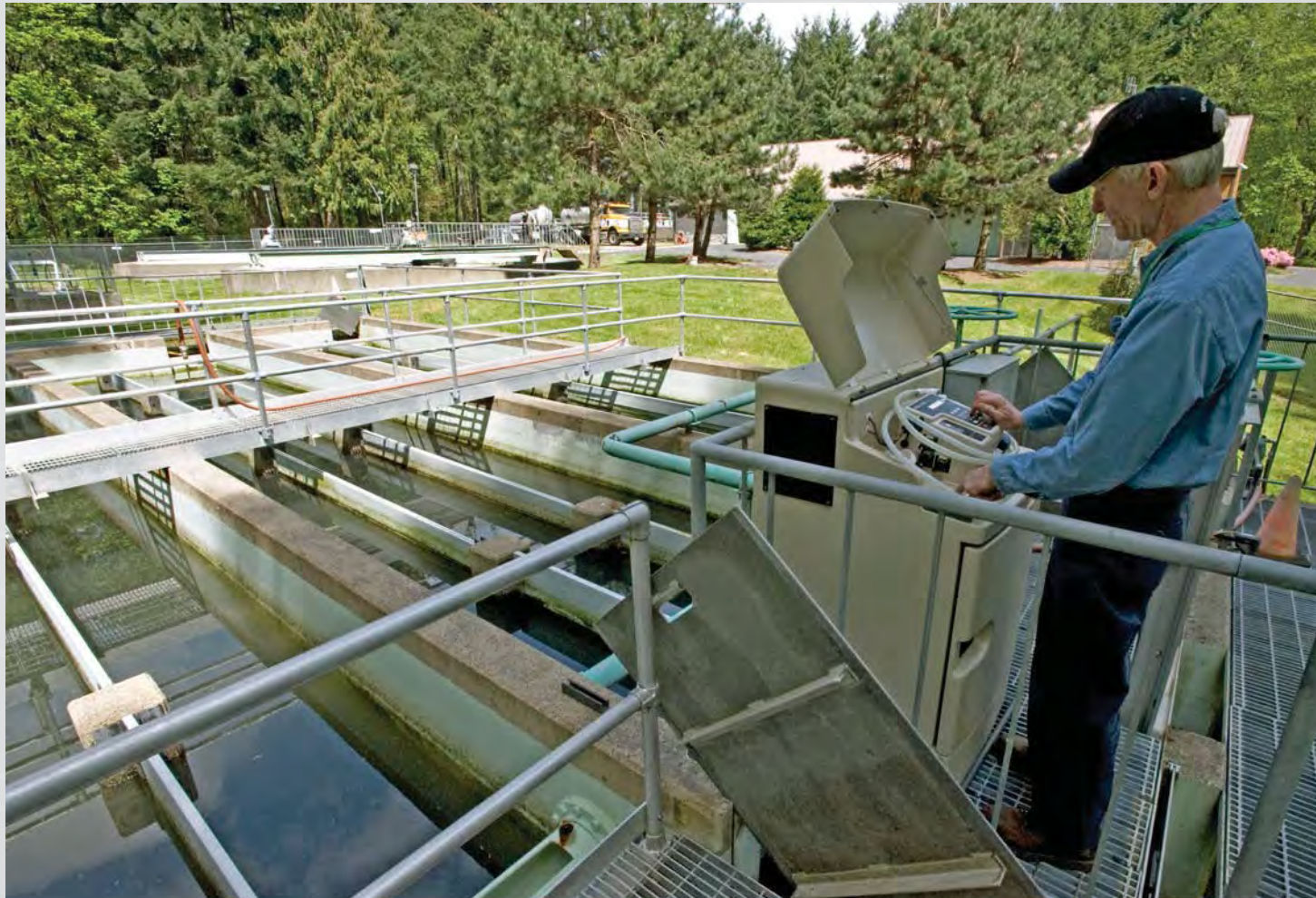
One of WES' Wastewater Plant Operators performs sampling of the effluent in the chlorine contact basin at the Hoodland Water Resource Recovery Facility in Welches, OR
