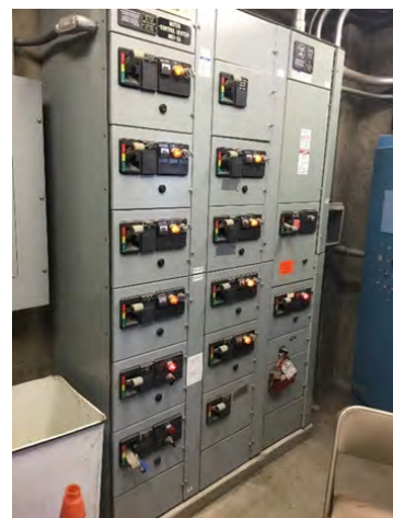
Picture 21. Motor Control Center MCC-2A
