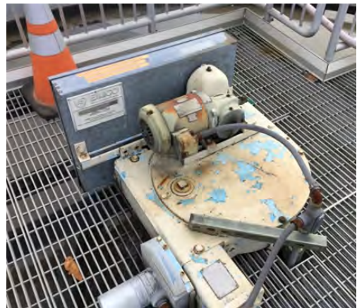
Picture 23. Secondary Clarifier Basin 1 Drive Assembly
