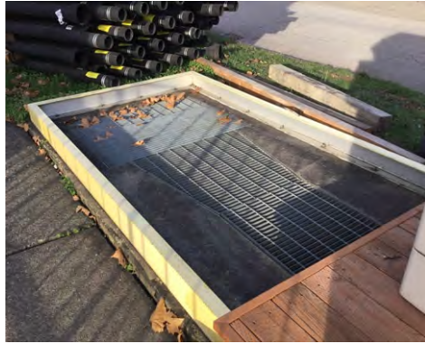
Picture 24. Secondary Influent Splitter Box
