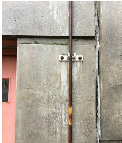
Picture 7. Screening Building
