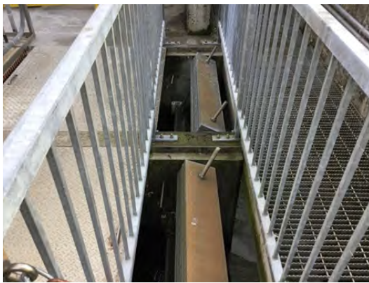
Picture 34. UV Influent Gate No. 2
