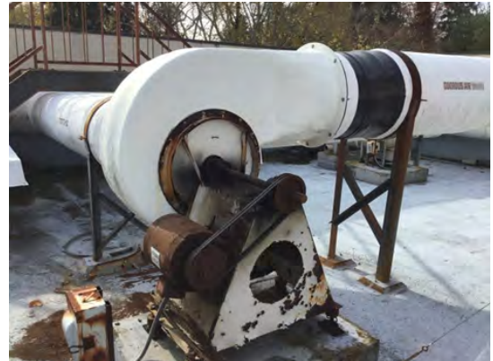
Picture 35. Digester Building Exhaust Fan 5
