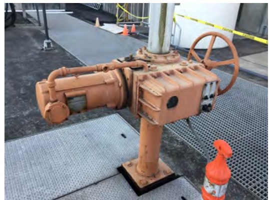
Picture 40. CCB 2 Isolation Gate
