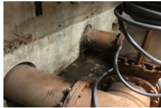
Picture 29. Activated Sludge Recirculation Pump Station Building
