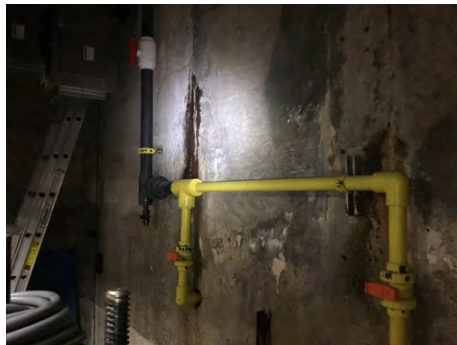
Picture 30. Activated Sludge Recirculation Pump Station Building
