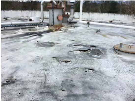
Picture 53. CAS Anaerobic Digester Tank 1
