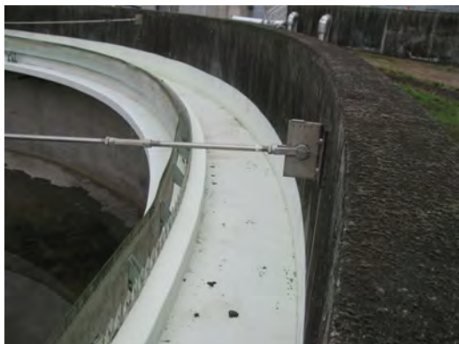
Picture 31. Secondary Clarifier Basin 1
