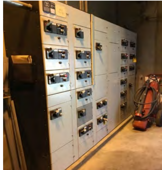
Picture 58. CAS MCC 7A-7B
