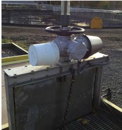
Picture 22. Secondary Clarifier 1 Motorized Actuated Influent Gate
