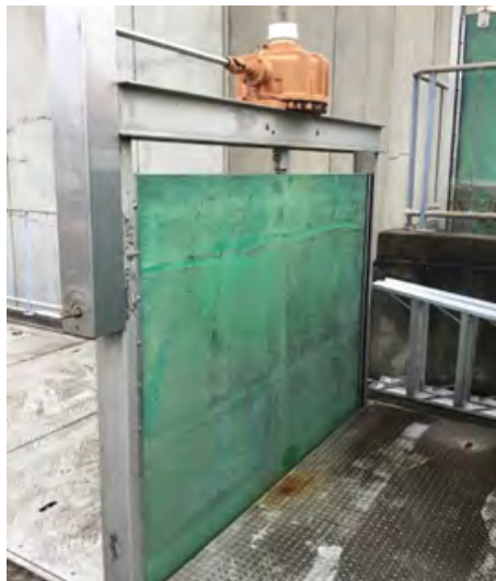
Picture 13. Primary Influent Channel Isolation Gate No. 1
