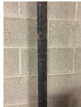
Picture 55. Chlorine Building Piping General
