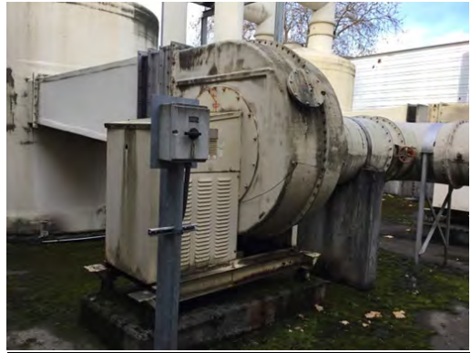
Picture 45. Carbon Vessel Digester 1 Exhaust Fan
