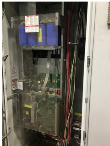
Picture 20. AHF-2 Active Harmonic Filter
