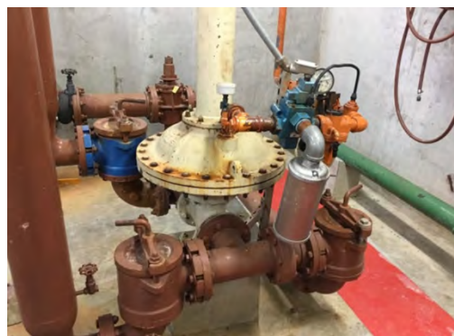
Picture 13. Primary Sludge Pump 2
