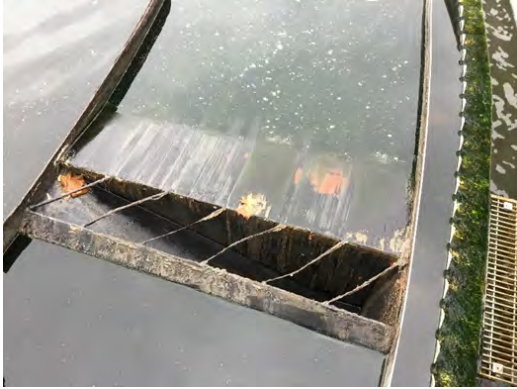
Picture 26. Secondary Clarifier Basin 2 Scum Skimmer
