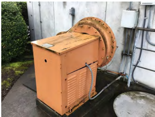
Picture 5. Influent Wet Well Odor Air Fan
