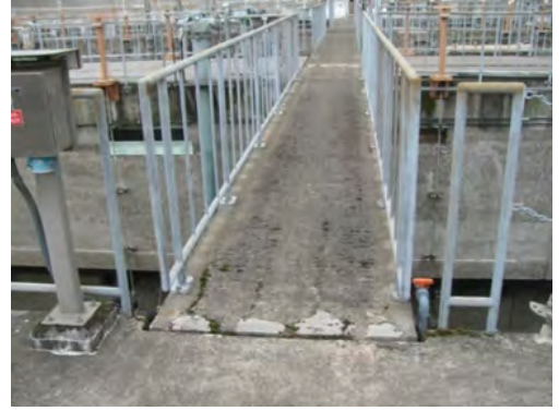
Picture 18. CAS Aeration Basin 1
