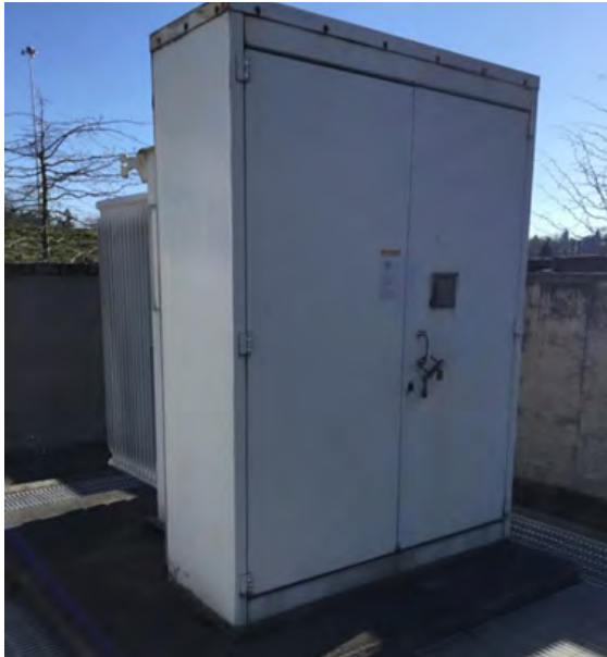
Picture 63. High Voltage Transformer 1A
