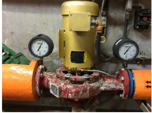
Picture 43. Heat Exchanger Hot Water Circulation Pump 2
