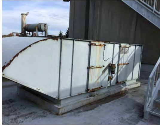
Picture 37. Digester Building Air Supply Unit
