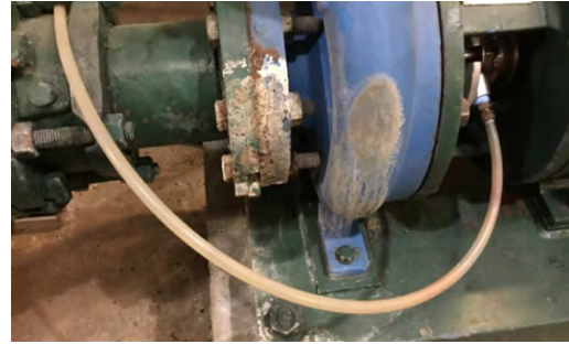
Picture 53. DAFT Recirculation Pump 2
