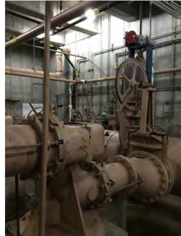
Picture 36. CAS RAS Pump 3
