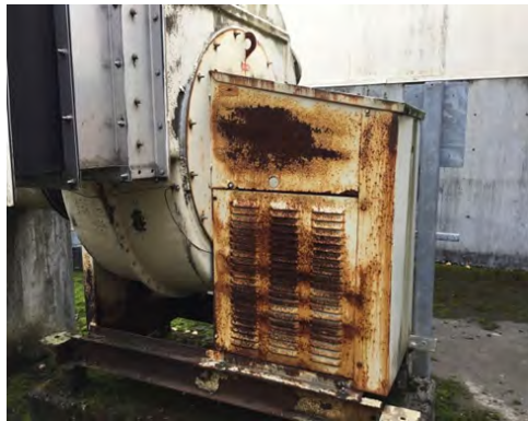
Picture 46. Carbon Vessel Digester 1 Exhaust Fan
