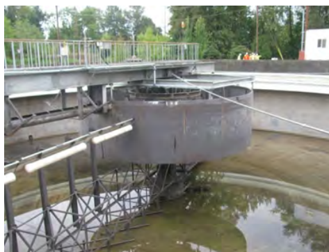
Picture 30. Secondary Clarifier Basin 1
