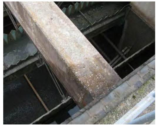
Picture 12. Primary Sedimentation Basin 1
