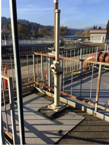
Picture 14. AB1 Main Step Feed Gate
