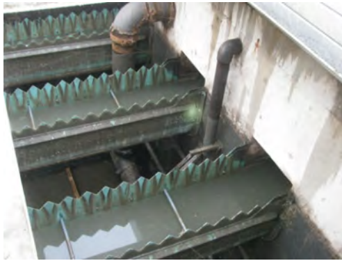
Picture 11. Primary Sedimentation Basin 1
