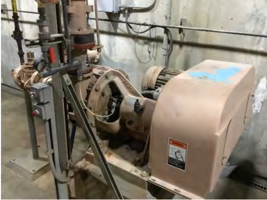
Picture 1. Grit Pump 2
