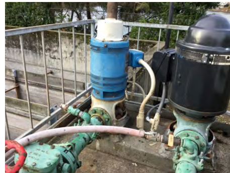
Picture 31. Non-Potable Water Pump 2
