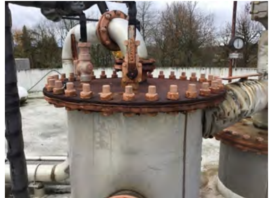
Picture 54. CAS Anaerobic Digester Tank 1
