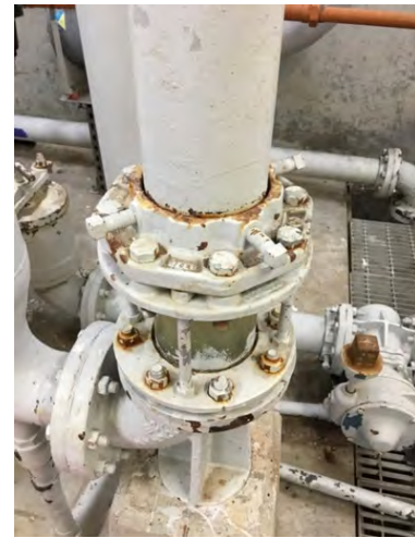
Picture 11. Primary Pump Station Piping General
