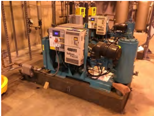
Picture 25. CAS Plant Service Air Compressor 1
