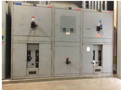
Picture 4. Influent Pump Station Switchboard
