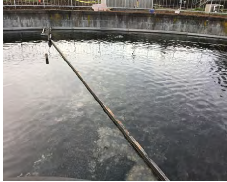
Picture 25. Secondary Clarifier Basin 1 Rake Arm
