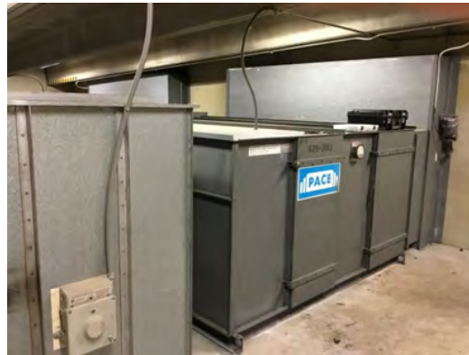
Picture 26. CAS Blower Building Air Supply Unit 2
