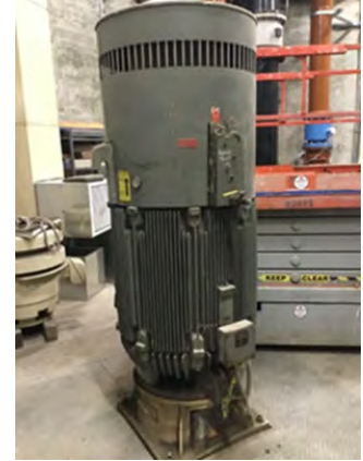
Picture 3. Main Lift Influent Pump 2 – Motor
