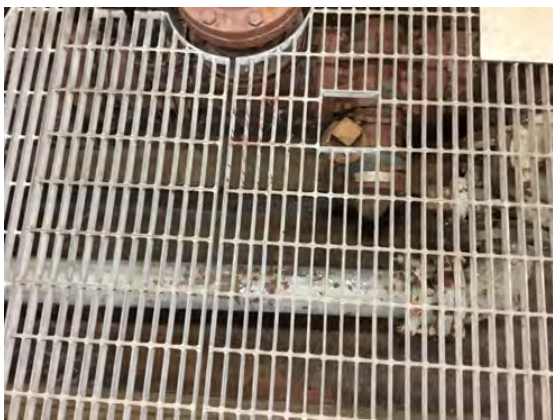
Picture 12. Primary Pump Station Piping General
