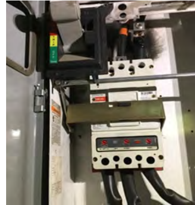
Picture 5. Blower Motor Control Center MCC 7
