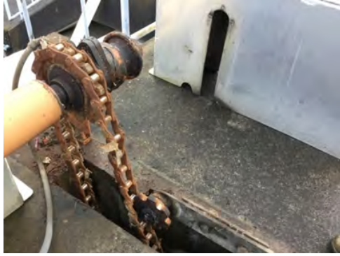
Picture 9. Primary Basin 1 Sludge Collector
