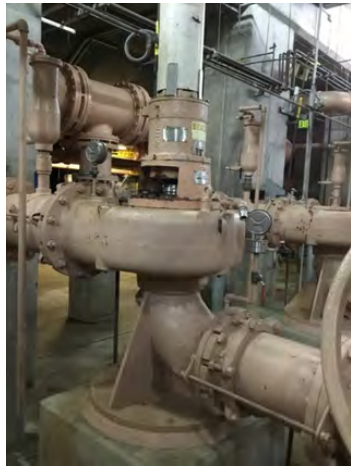
Picture 35. CAS RAS Pump 2
