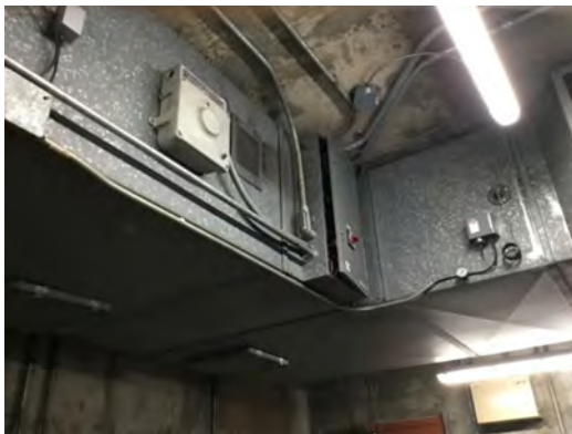
Picture 27. CAS Blower MCC Room Duct Heater
