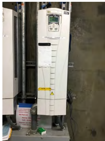
Picture 28. CAS Plant Service Air Compressor 1 PLC
