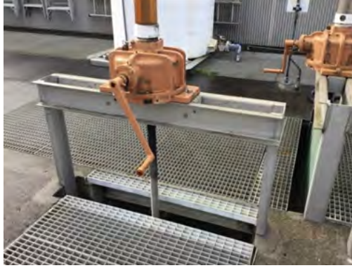
Picture 17. CAS AB3 Complete Mix Effluent Channel Isolation Gate
