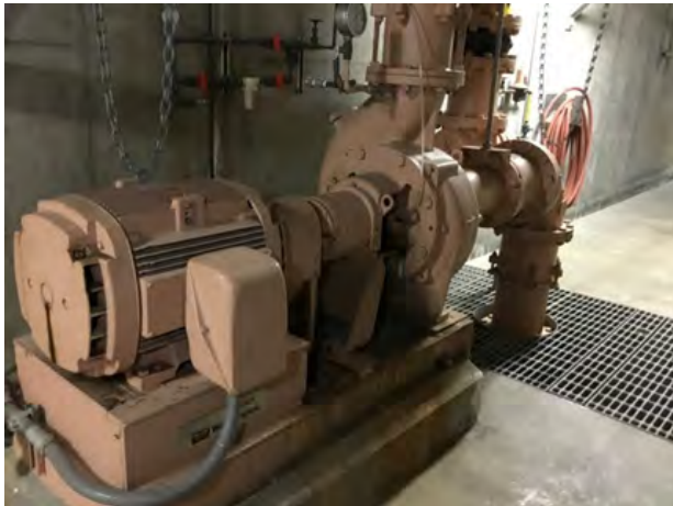
Picture 21. CAS AB1-2 Dewatering Pump
