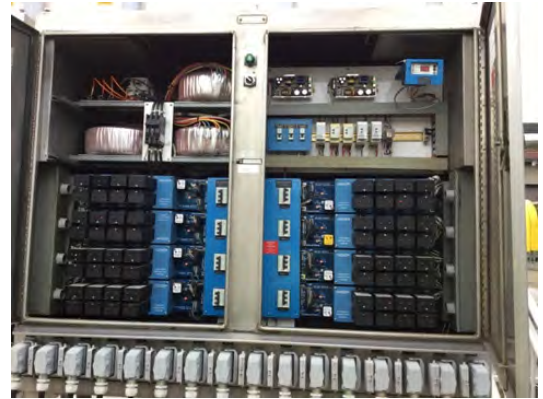
Picture 33. UV Channel 1 Cassette 1A Control Cabinet
