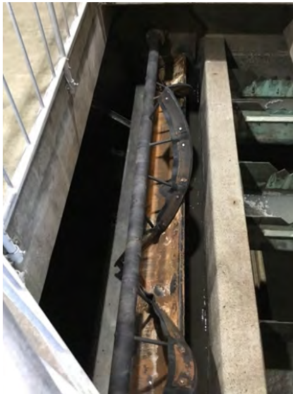
Picture 15. Primary Helical Skimmer Basin 2
