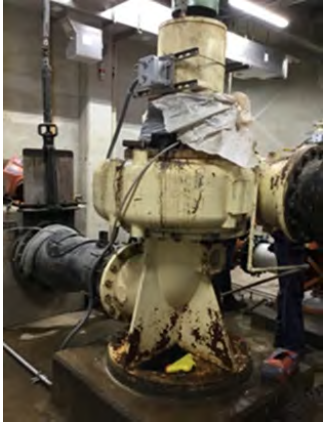
Picture 1. Main Lift Influent Pump 2
