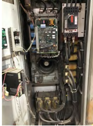
Picture 2. Influent Pump 4 Variable Frequency Drive
