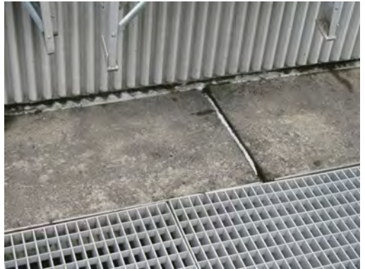
Picture 20. CAS Aeration Basin 1
