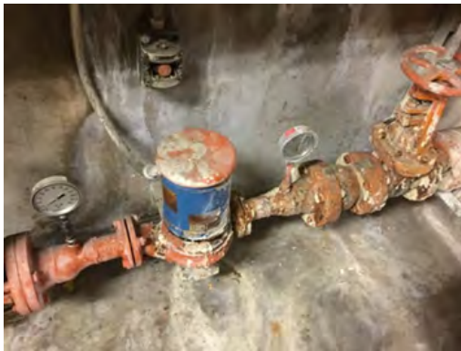
Picture 44. Digester Complex Piping General
