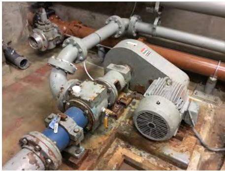
Picture 28. Secondary Scum Pump
