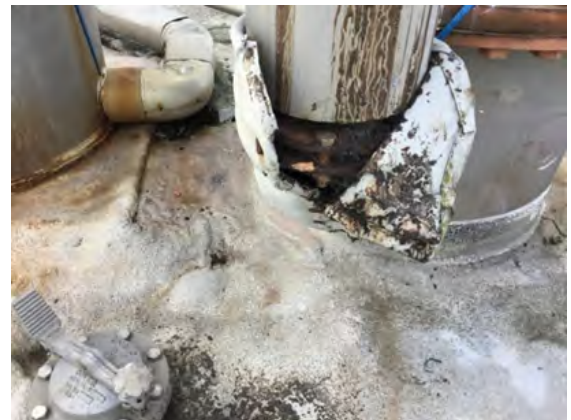
Picture 56. CAS Anaerobic Digester Tank 1
