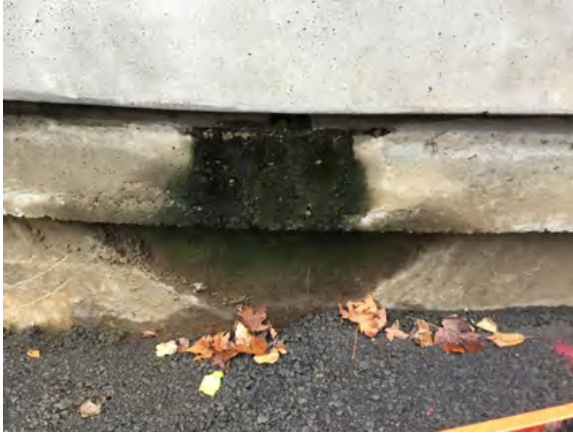
Picture 51. CAS Anaerobic Digester Tank 1
