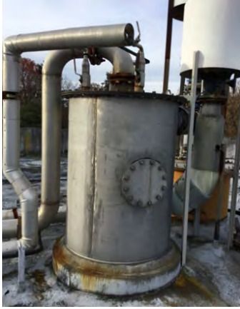
Picture 36. Digester 1 Foam Separator
