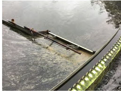
Picture 27. Secondary Clarifier Basin 2 Scum Skimmer
