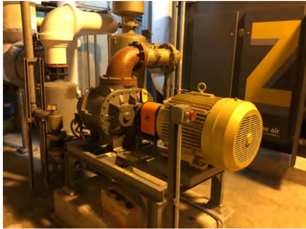
Picture 24. CAS Channel Blower 2
