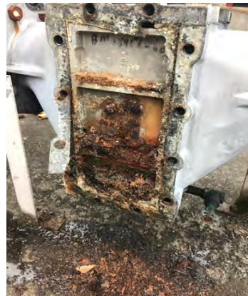
Picture 49. Sludge Holding Tank Flame Arrestor 1
