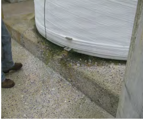
Picture 41. CAS Chlorine Contact Basin
