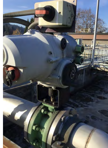
Picture 15. AB4 Zone 4 Air Flow Control Valve
