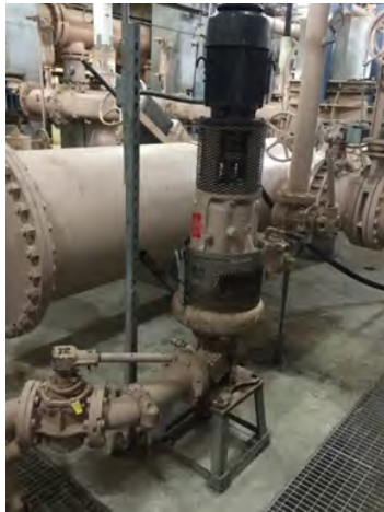
Picture 37. CAS Secondary Scum Underflow Pump
