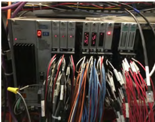
Picture 4. Local Control Panel 1 - PLC01
