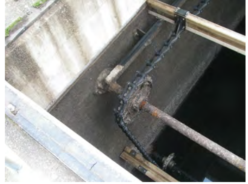
Picture 10. Primary Sedimentation Basin 1
