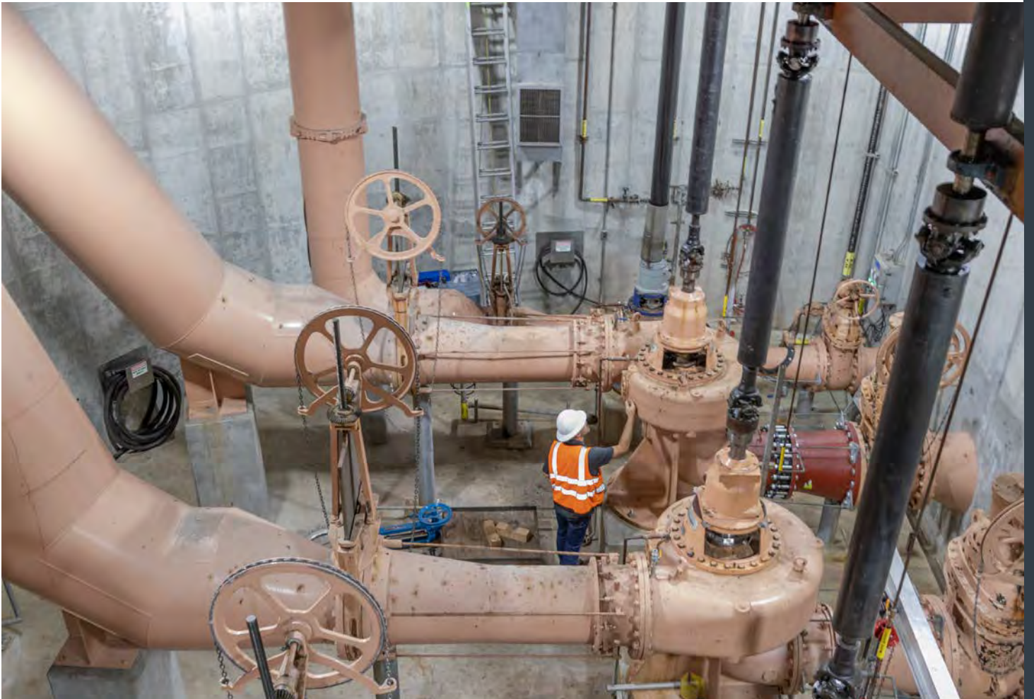
Checking pumps at the Tri-City Water Resource Recovery Facility
