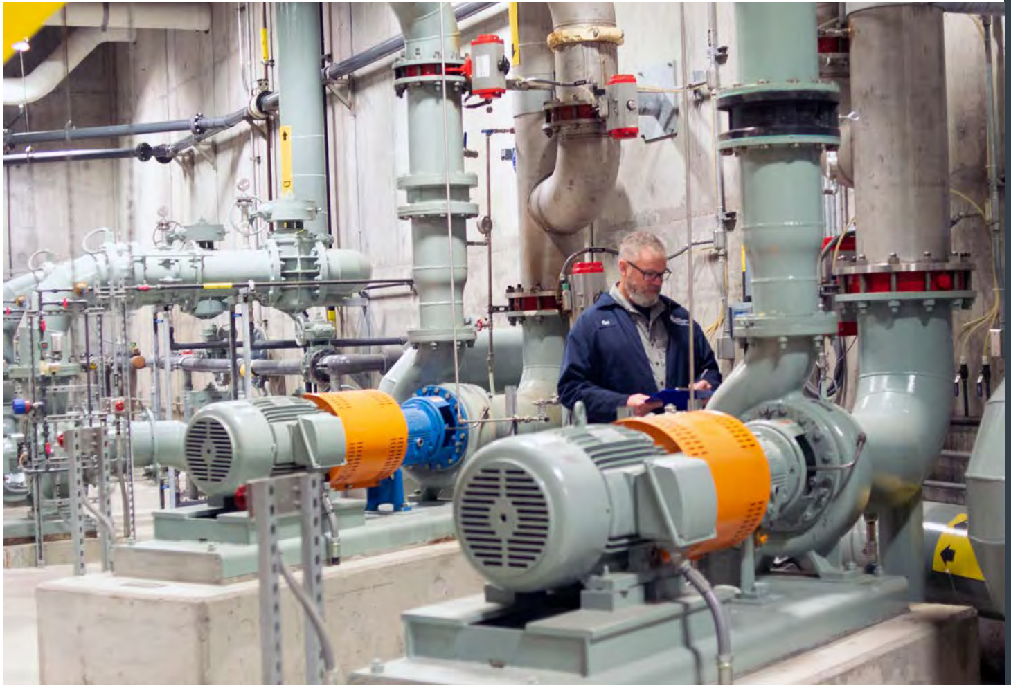
Checking the blowers at the Tri-City Water Resource Recovery Facility
