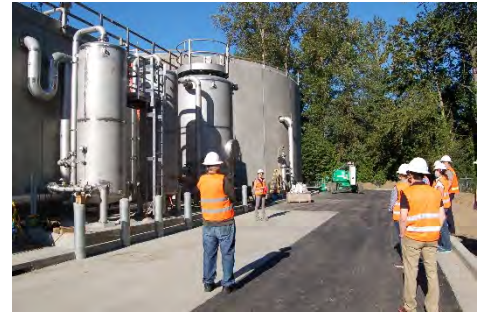
2022 – Touring the new digester at the Tri-City WRRF
