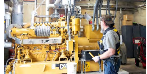
2023 – Biogas cogeneration engine at Tri-City WRRF
