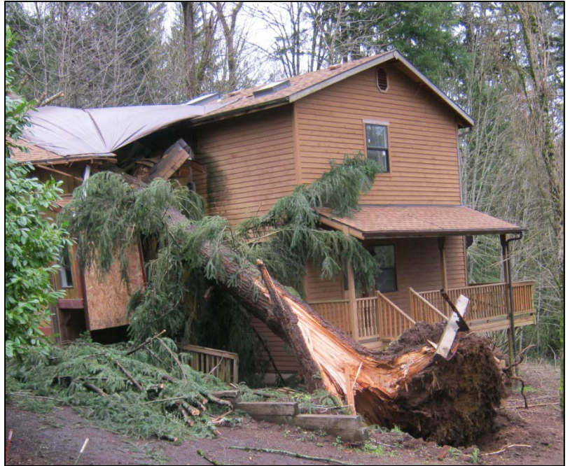
Windstorm damage – March 13, 2011
