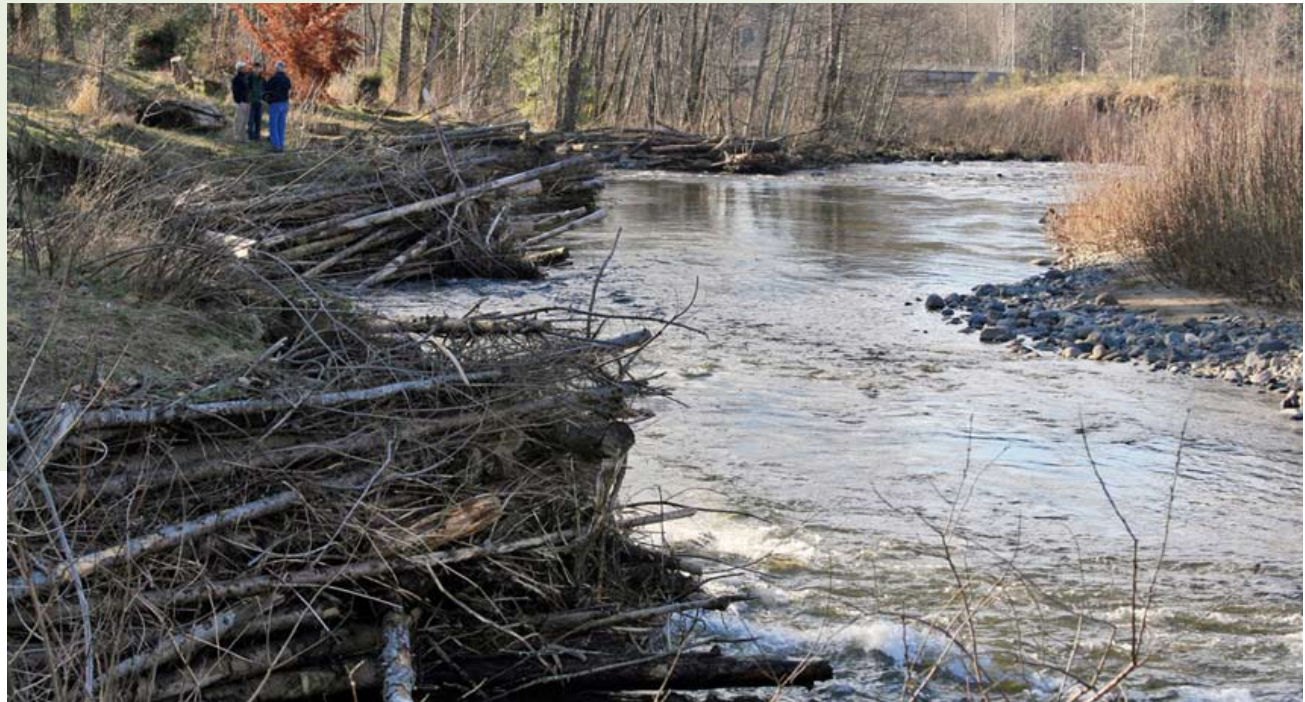
Four of the engineered logjams designed by Herrera Environmental Consultants on the Mashel River outside of Eatonville, WA.
