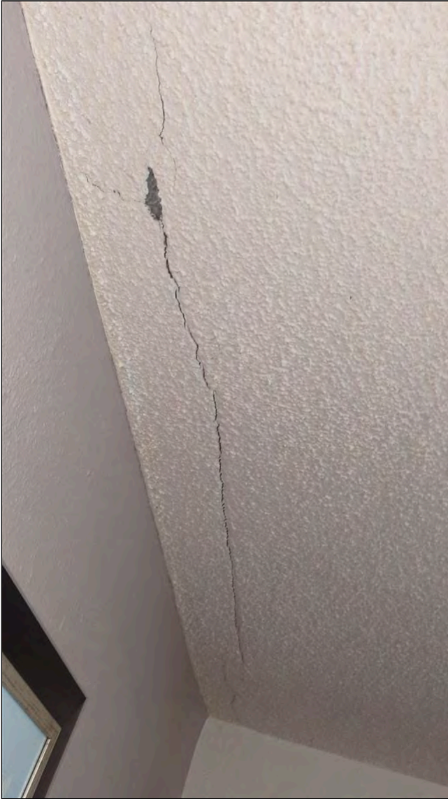
A.12. Item 1(Picture) Cracking damage in ceiling
