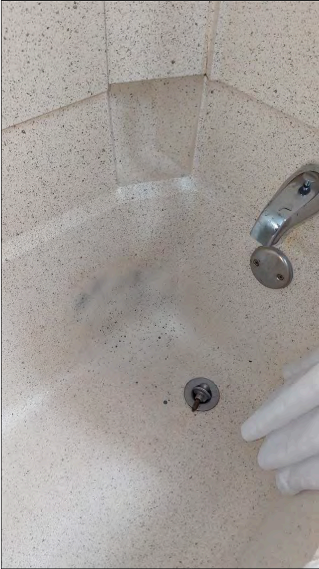
A.38. Item 3(Picture) Chipping and discolored paint and bathtub
