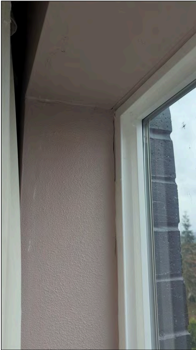
E.24. Item 3(Picture) Window caulking damage needs repaired
