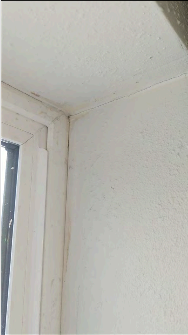
E.12. Item 3(Picture) Window seal needs repair
