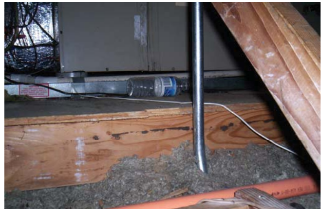
Attic mechanical platform
