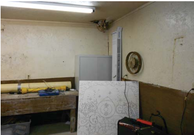
Roof leak damage (2014)
