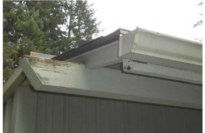
Entry beam decay
