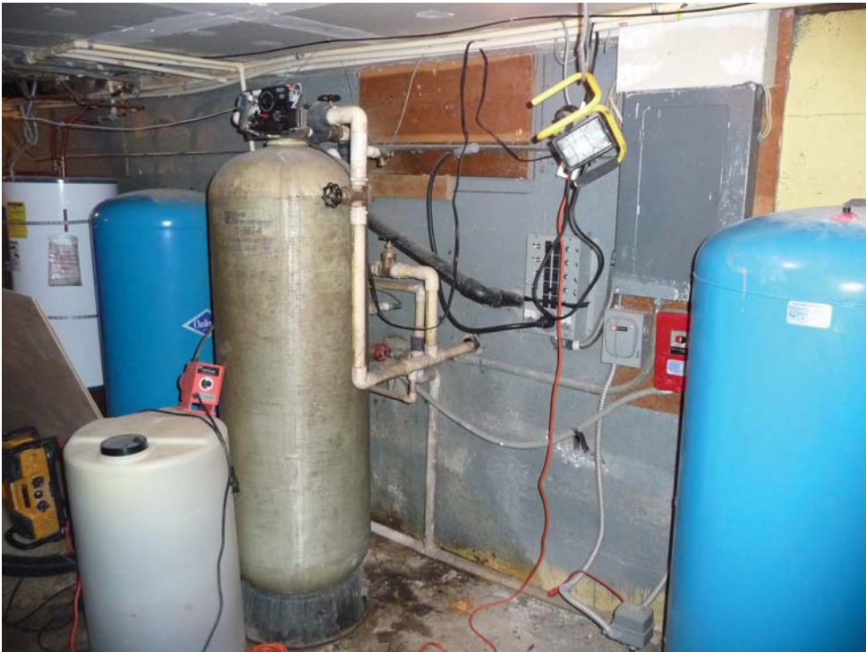
Two pressure tanks (blue), water softener (grey) and chlorine dosing tank (white)
