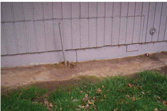
Stem wall crack
