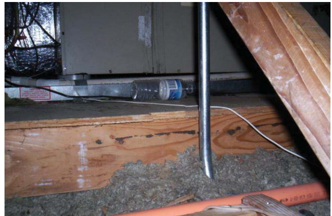
Attic mechanical platform
