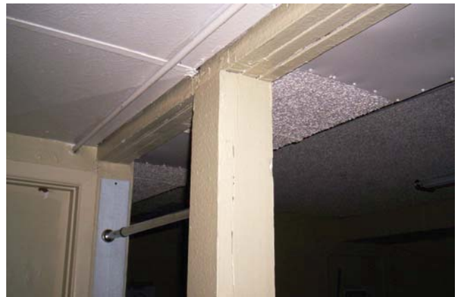
Basement post top
