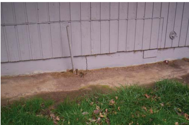
Stem wall crack
