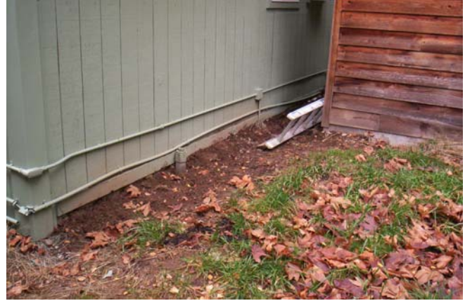
Soil against siding
