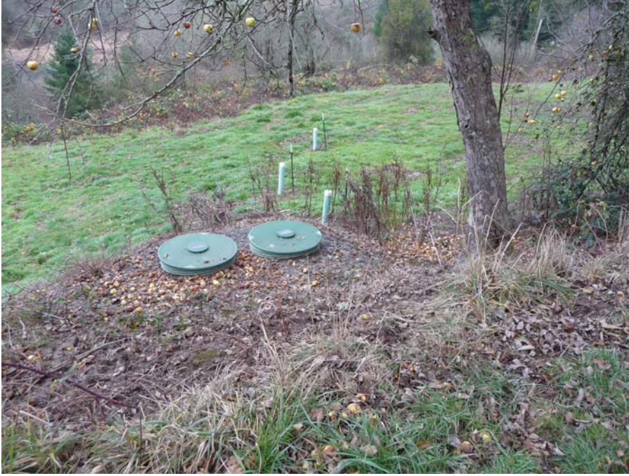
Two hydrosplitters at the west drainfield
