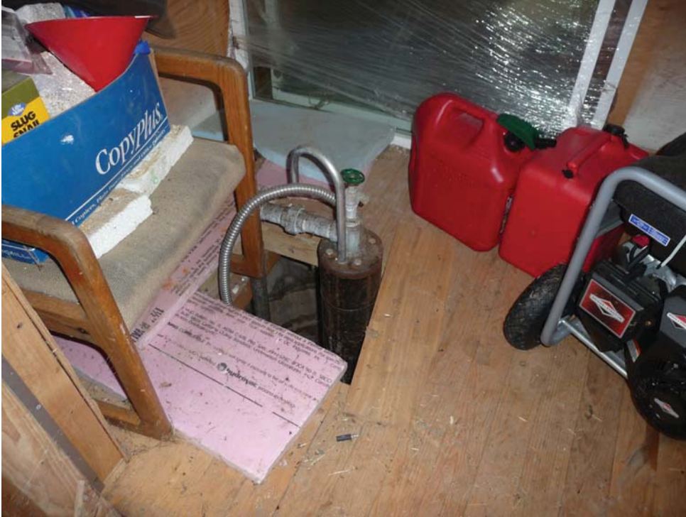
6" Wellhead within the pump house.
