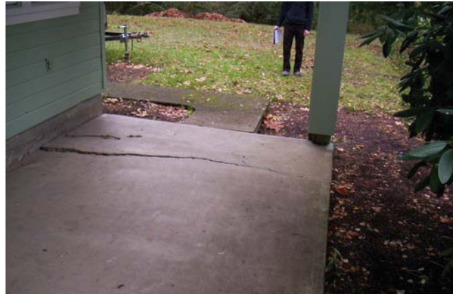
Settlement at entry porch and decayed post base
