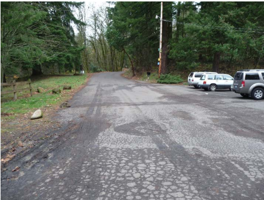
Pavement base failure (cracking) at main entrance
