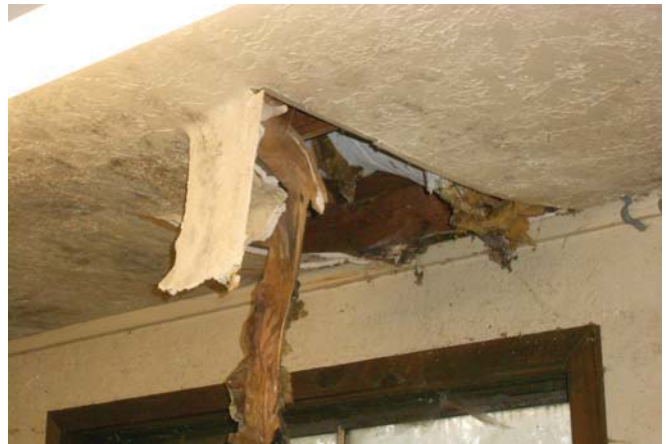
Roof leak damage (2014)
