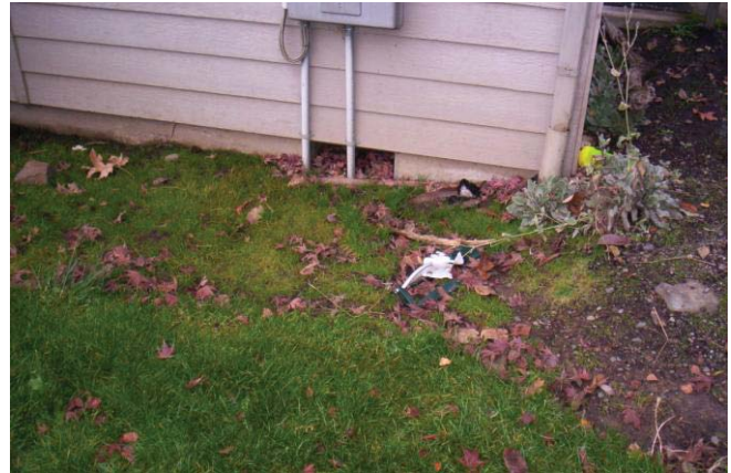
Grade at crawl space vent
