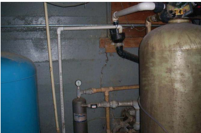
Basement north wall crack
