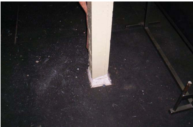
Basement post base
