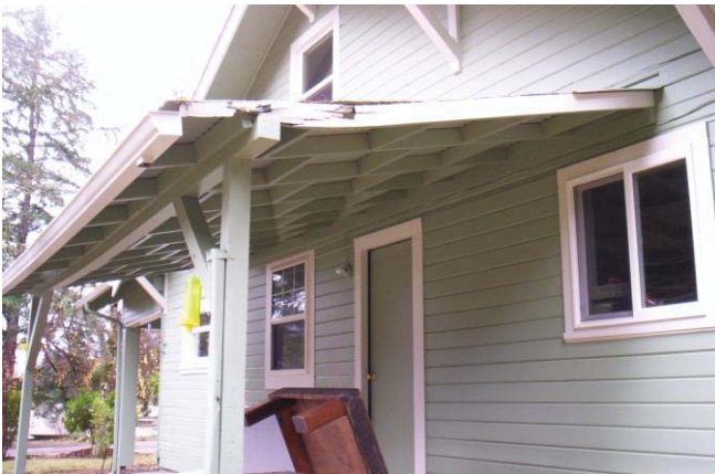
Patio beam and decayed fascia
