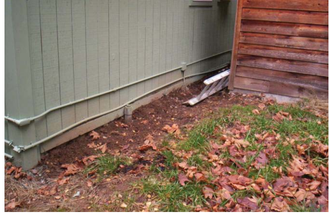
Soil against siding
