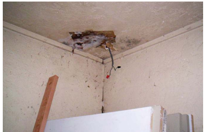
Roof leak damage
