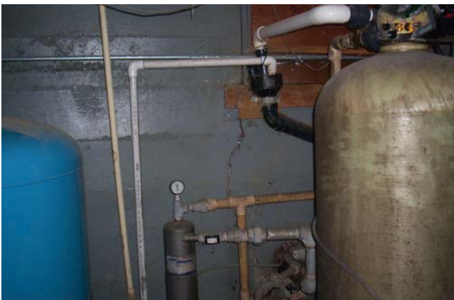
Basement north wall crack
