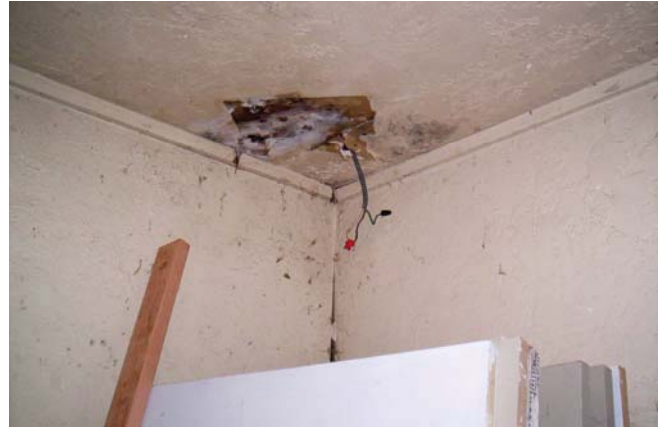
Roof leak damage (2009)
