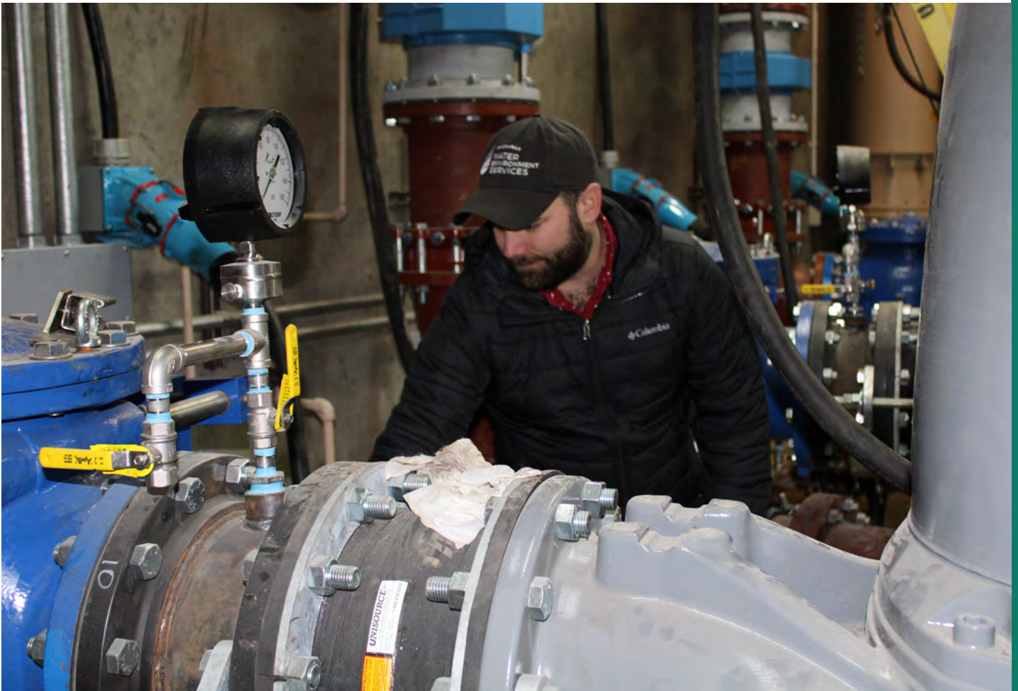
The inner workings of a pump station
