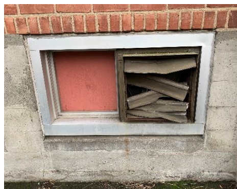
Louver into mechanical space
