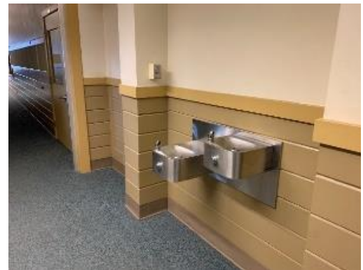
Accessible drinking fountains, upper level, north wing
