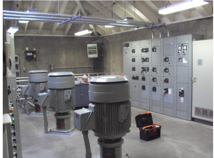
Willamette Pump Station
