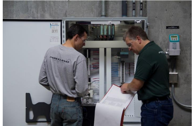
Site Acceptance Testing at Tri-City PLC7R
