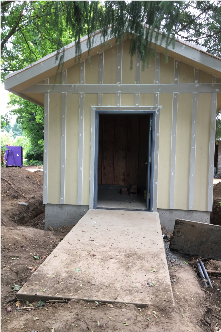
New pump house
