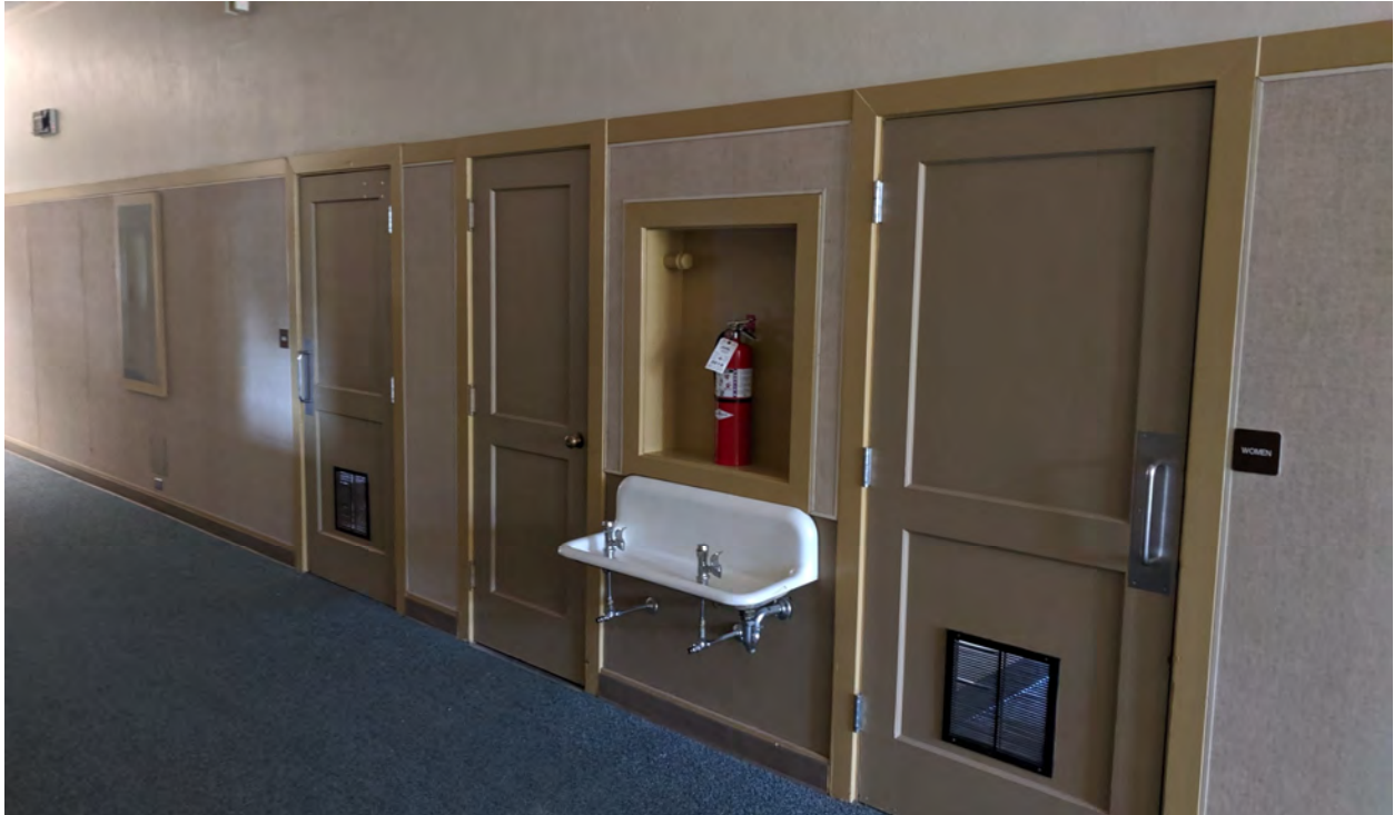
Representative view of paneled wood doors and drinking fountain in upper-floor central corridor in 1936 building (ARG, October 2019).
