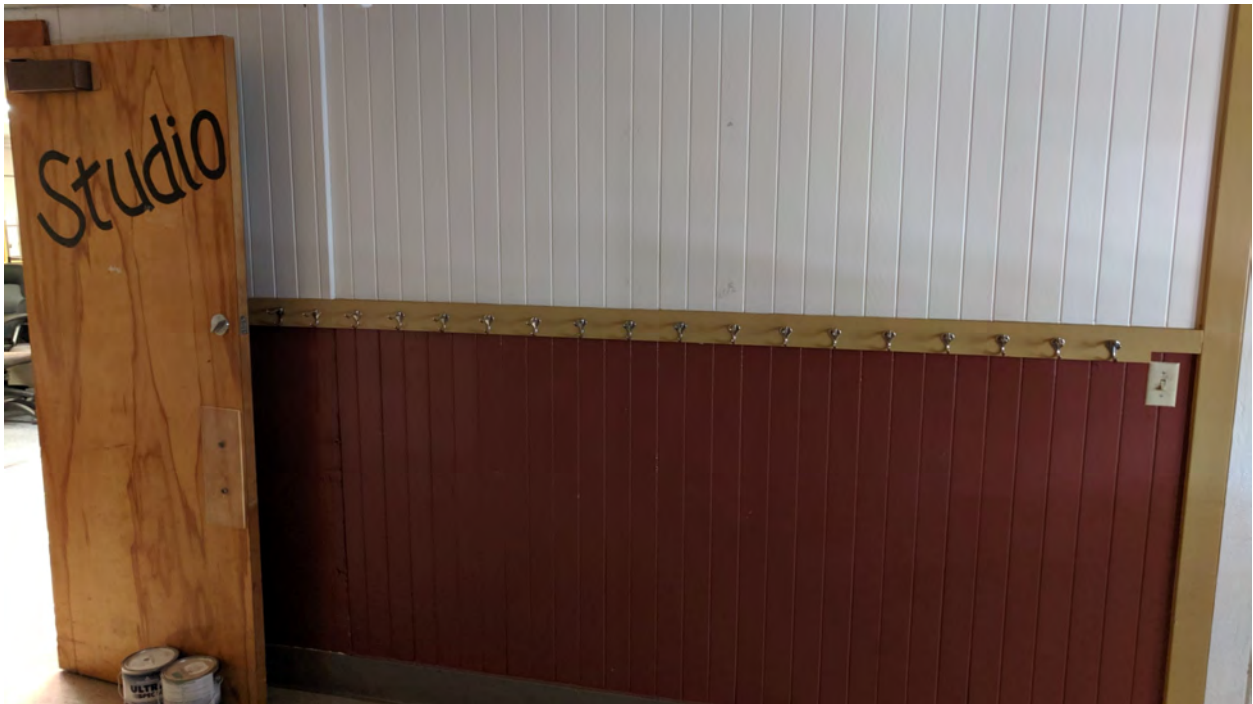
Representative view of beadboard wall paneling in basement of 1936 building (ARG, October 2019).
