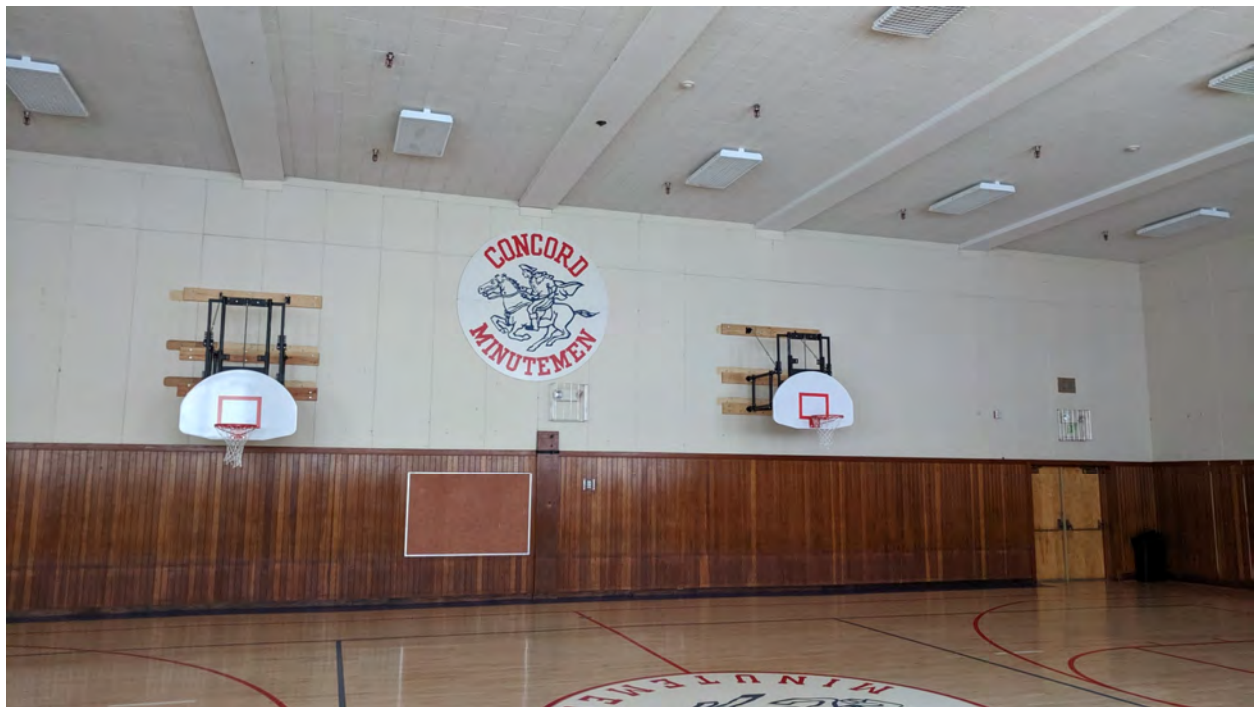
Representative view of wainscot in gymnasium/auditorium in upper floor of 1936 building (ARG, October 2019).
