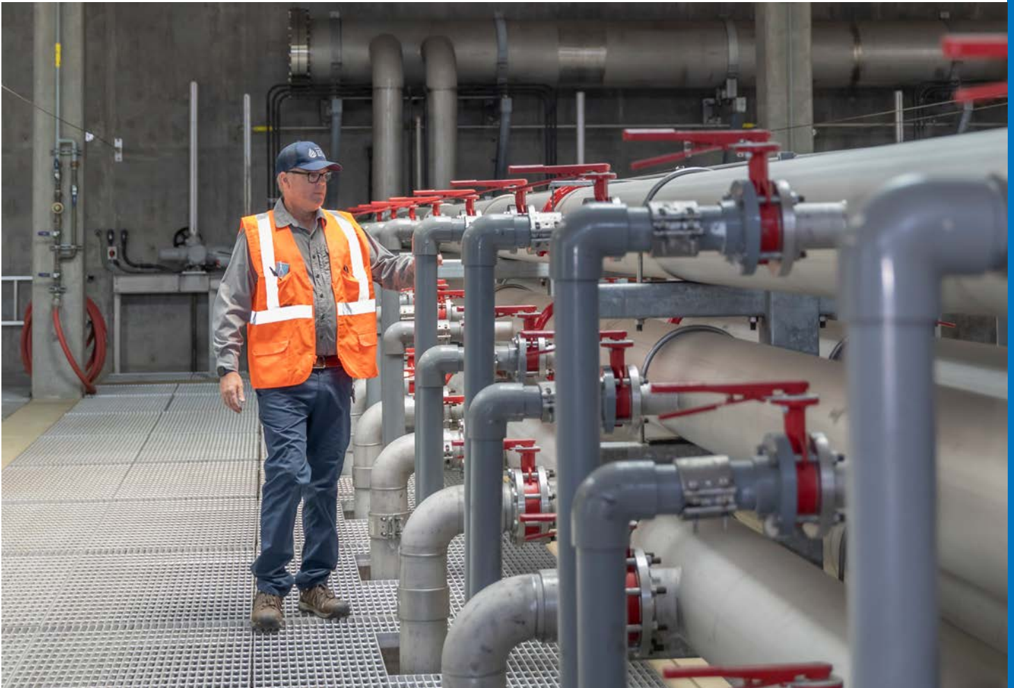
Keeping everything running smoothly at the Tri-City Water Resource Recovery Facility
