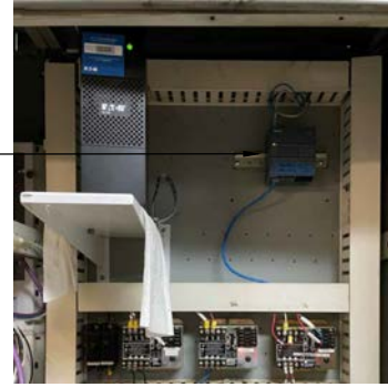
EXISTING CONTROL PANEL INTERIOR DETAIL ①
