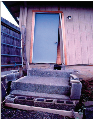
House cracks. Photo credit: Scott Burns.
