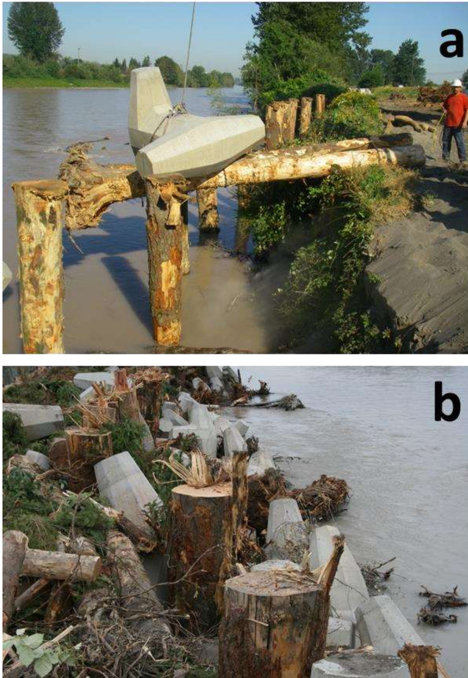
Figure 44A/B. Using a combination of timber and dolosse has been used in Washington State as a more restorative alternative to traditional measures to protect levees and roads. The dolosse are eight ton unreinforced concrete jacks that provide a complex interlocking shape emulating the function of natural snags. The top photo (a) shows how a dolo and attached log can be easily lowered into place and avoid expensive dewatering. Using the dolosse with logs creates a complex structure as shown in bottom photo (b) that can settle if undercut by scour, but without the need of rock or cable. The structures can be designed with lots of wood so the dolosse aren't even visible. Since they are self-settling, these structures don't need to be deeply
