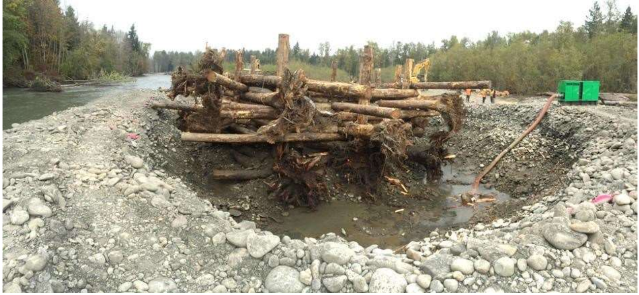
Figure 43. Example of engineered logjam that doesn't have self-settling elements of previous examples. This structure is deeply embedded into the river so that it can withstand scour without being compromised. Note people on right side of the structure. Pit is 16 feet deep and timber posts extend deeper. Elwha River 2014.
