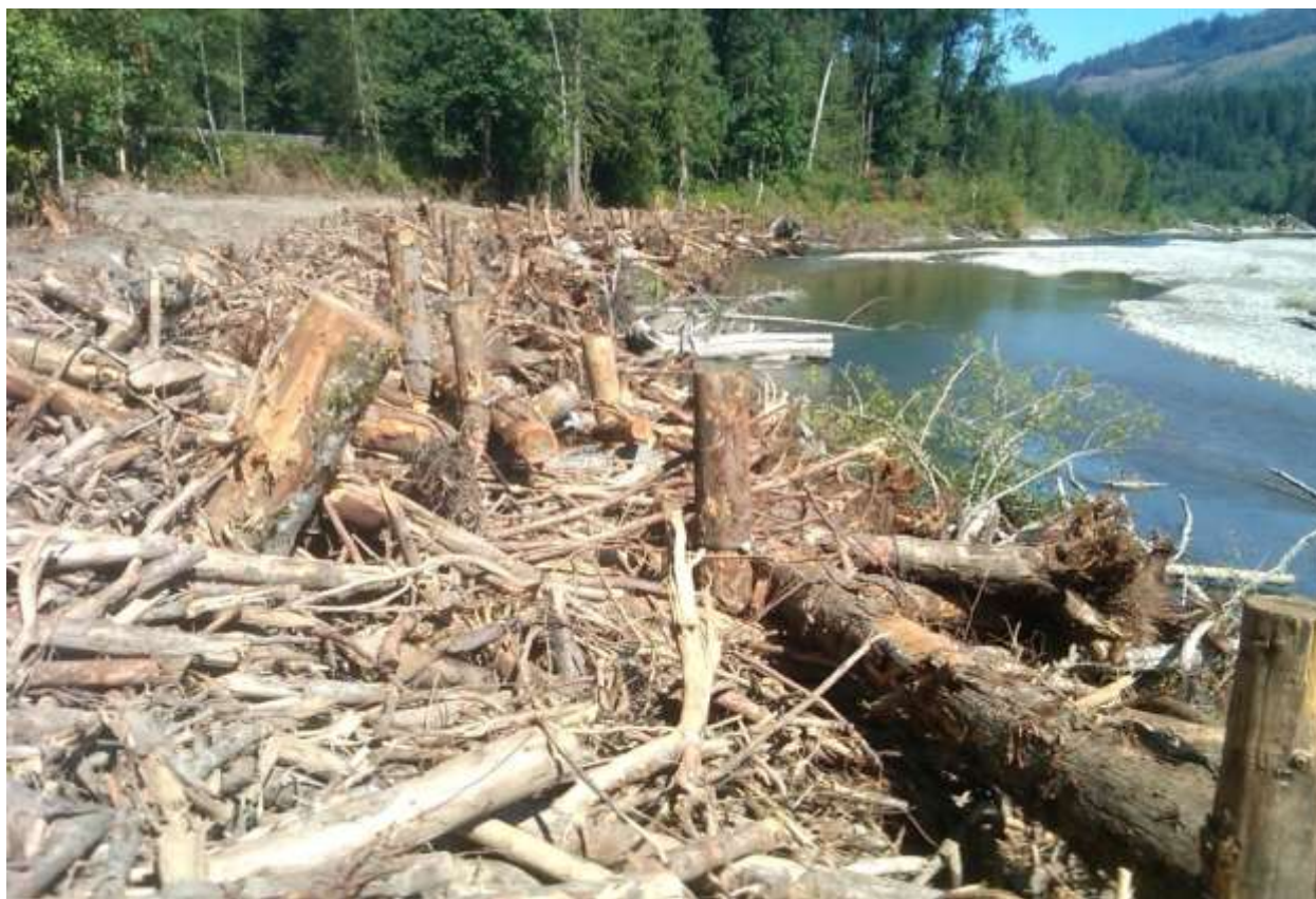
Figure 46. Example of an engineered complex timber revetment bank protection creating a rough shoreline very different than traditional rock revetments found along Sandy River. The structure along the South Fork Nooksack River in northwest Washington is stabilized with timber piles and rock collars (no dolosse). Structure was built in 2011 by Lummi Indian Nation.
