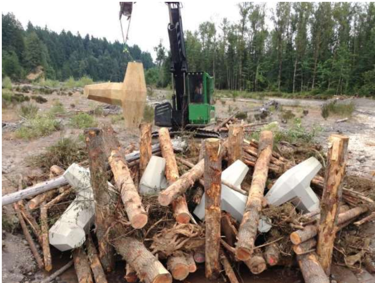
Figure 45. Construction of ELJ using 8 ton dolosse in Upper Puyallup (same structures depicted in Figure 40). The dolosse offer an interlocking ballast the structure can settle into river bed if undermined without coming apart. This means the structures don't require as much excavation, lowering construction impacts and costs. Dolosse are covered with alluvium and wood so they are barely visible in completed structure. View is looking upstream into core of the structure.
